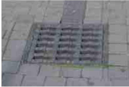
✓ Cast iron covers without visible concrete surround
