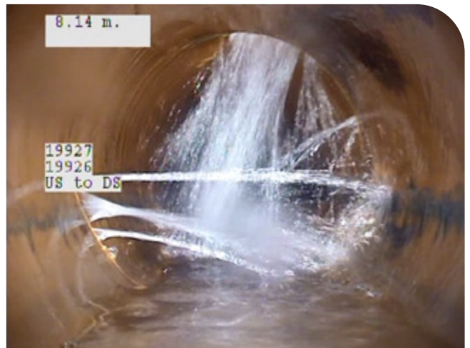
CCTV footage of groundwater infiltration getting through cracked pipes
