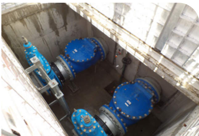
Tay Street Drain #1 check valves, part of Flockton Basin flood mitigation work stormwater
