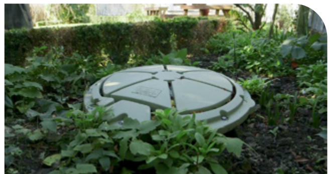
Residential pressure wastewater unit, east-central Christchurch
