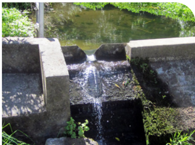
Intake for Duvauchelle water supply, Piper Stream
