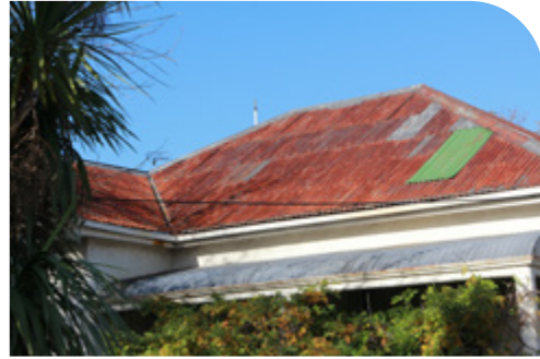
Rusting unpainted roof
