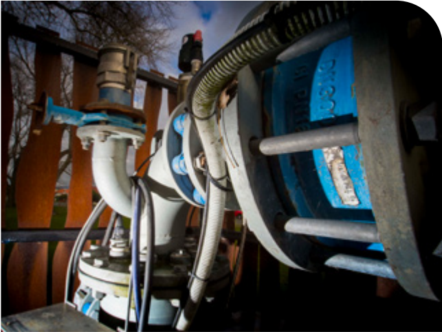
Above-ground well head
