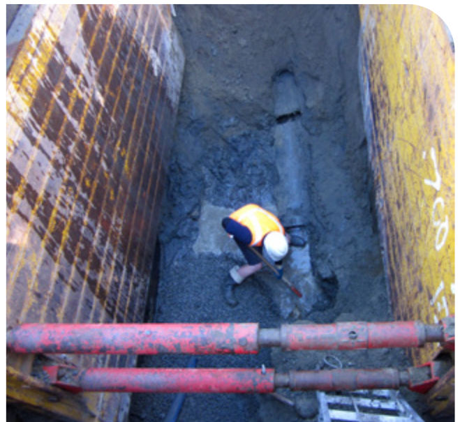
Wastewater pipe damage in February 2011 earthquake
