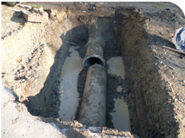
Earthquake damaged pipe
