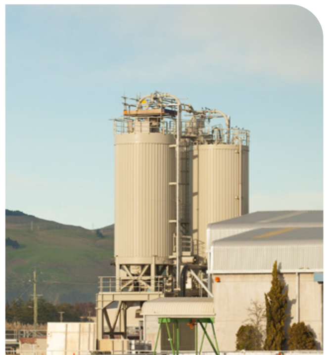
Biosolids dryer, Christchurch wastewater treatment plant
