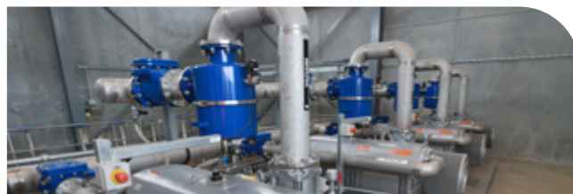
Vacuum wastewater pump station in Aranui is an example of greater infrastructure resilience
