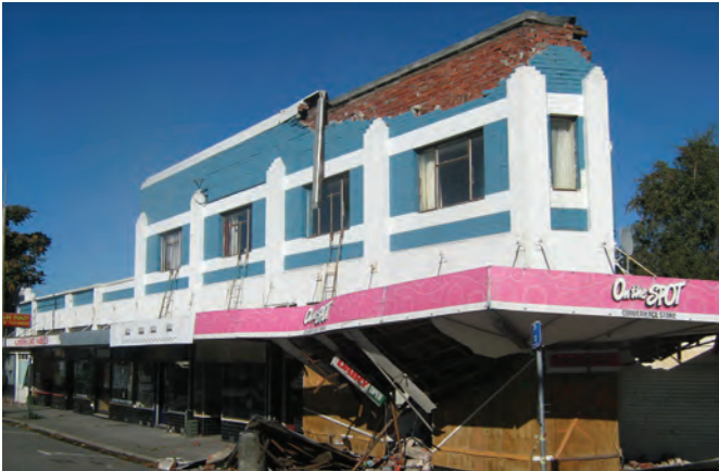
Figure 5. March 2011, damage to 299 Selwyn Street block
