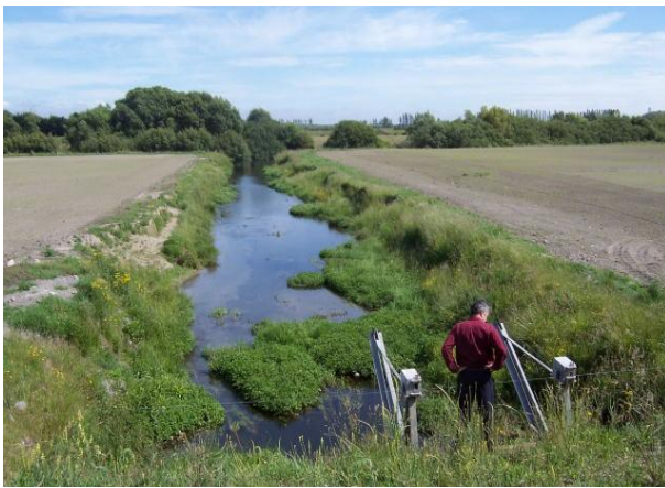
Twin culverted Outlet West of Motorway
