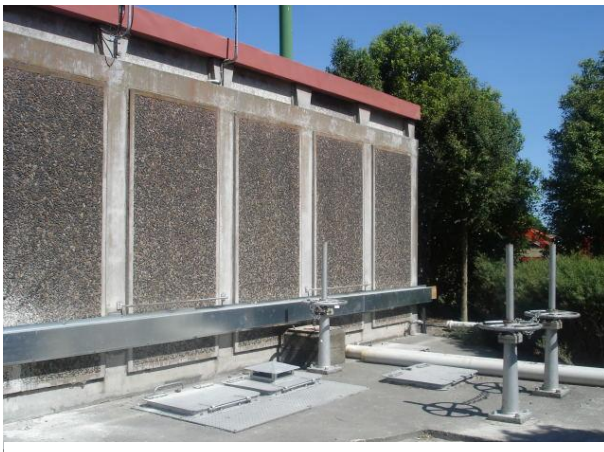
Tyrone Street Wastewater Pump Station
