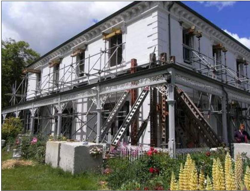
Godley House post earthquake. http://www.civicassurance.co.nz/bigone.htm
