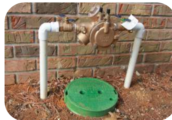
Backflow Prevention Device
