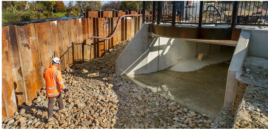
A control structure at a facility to provide storage to mitigate flood flows.
