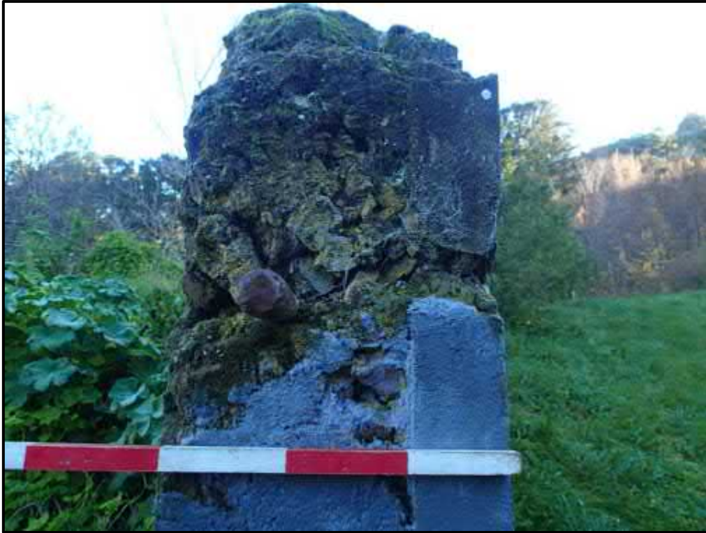
Figure 25. The Fort Erskine concrete perimeter wall, showing the local volcanic rock as aggregate and pin that would have held the entrance gate.
