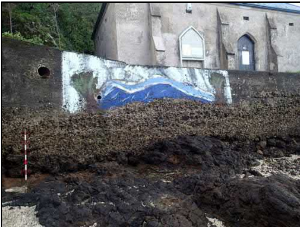
Figure 35. The 1874 sea wall with magazine building in the background. Note how the sea wall has been constructed directly atop the existing rocks, and that there is weathering of the lower part of the wall from the action of the sea.
