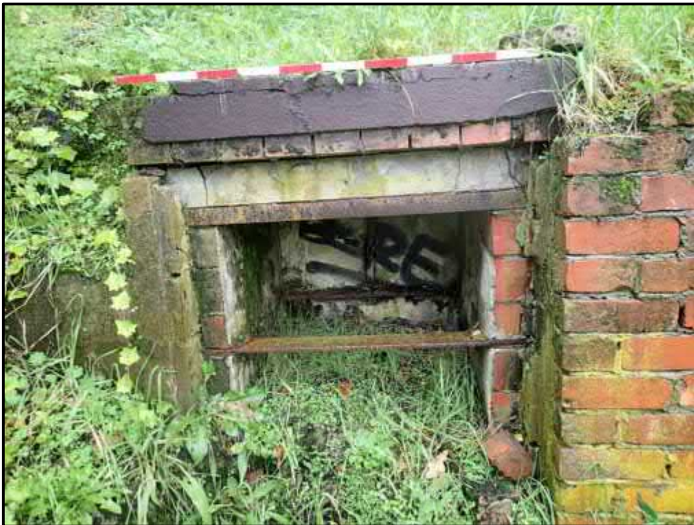
Figure 31. The meat safe built into the northern end of the retaining wall.
