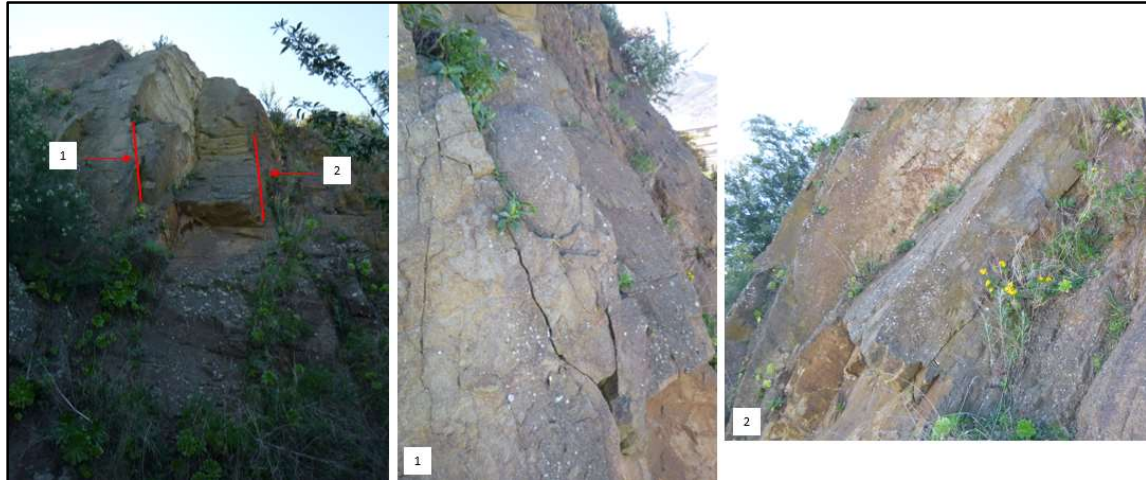
Figure 4 Left image - unstable site (previous wedge failure), red lines indicate location of persistent defects on each block, arrows indicate the direction that the close up photo has been taken. Right images – images to illustrate the defects outlined in the left image.
