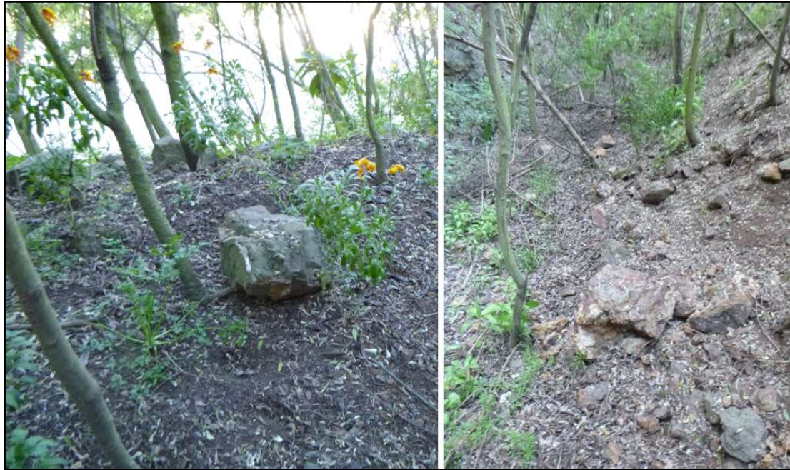
Figure 5 Left image - rockfall observed on the top of the bund. Right image – rockfall observed on the upslope side of the bund.
