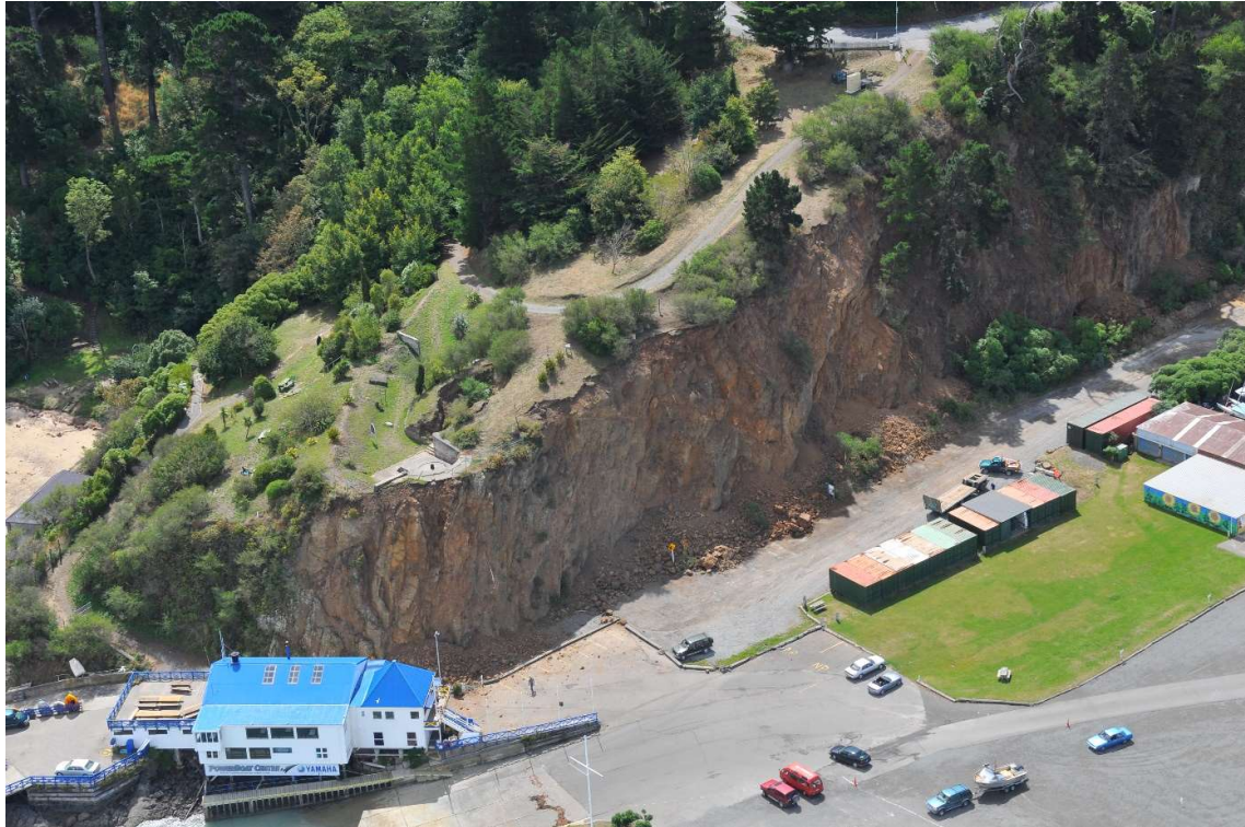
Figure 2 Naval Point on February 24, 2011. Fresh rockfall can be seen in the car park adjacent to the yacht club (blue roofed building). Much of the rockfall visible at the base of the cliffs is fresh, though some is likely to have been present already. Photograph by G Hancox, GNS Science.
