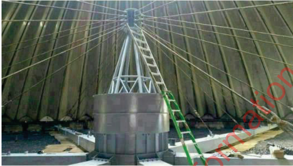
Image 3: The internal structure during a maintenance project several years prior to the fire. Circa 2016. Detail showing the central pivot and supports. (Photo supplied by CCC).
