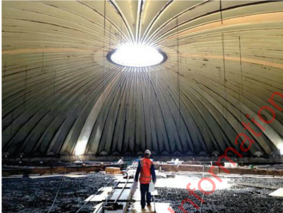
Image 11: The internal structure of the roof dome. No forms of electrical hazards were present within this area of the processing plant.
