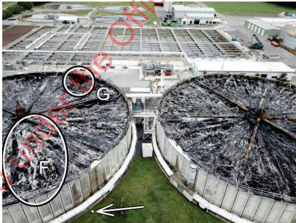
Photo 9: Two areas of significant damage in the Trickling Tank #2 were identified. Circle "F" is believed to be where the first collapse of the roof occurred. Circle "G" is downwind from this location at an intensified area of burning. (Photo supplied by FIS DJI_0226.jpg)
