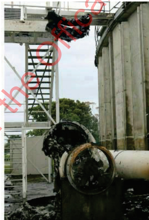
Photo 4: Ventilation fan area at the base of the access stair between the tanks identified as "C" in Photo 2. This area was consumed by fire after the fire was discovered on the roof of Tank #2.
