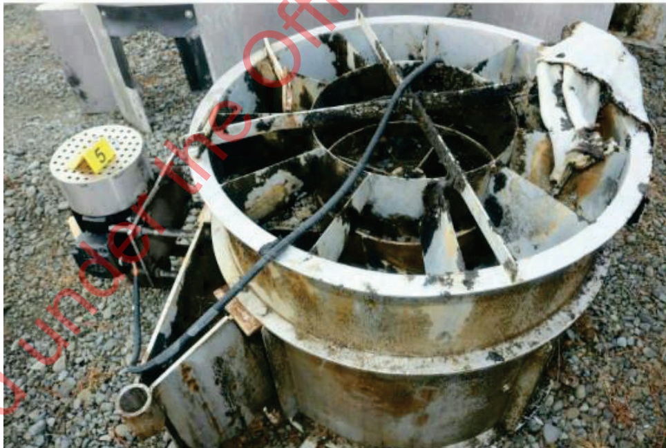
Photo 7: Motor and fan #5 showing burnt product within the cowling of the fan unit. Motor was unaffected by fire when electrically tested. Drive belt intact and unaffected by fire. Fan #5 was located Trickling Tank#2 North West corner.
