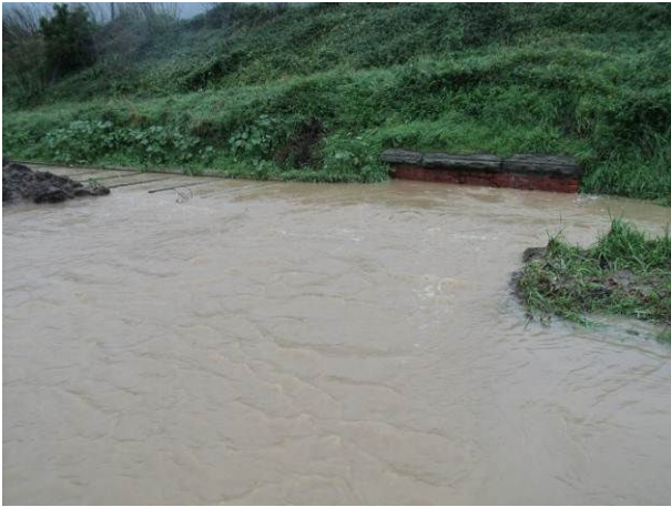
Figure 19 Truscotts Road outlet of 1200 mm brick barrel after trimming sections of berm
