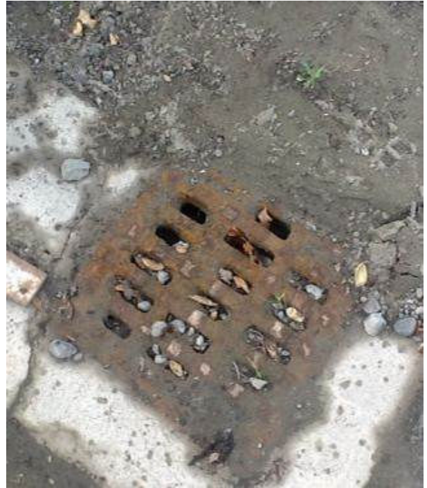
Figure 34 Blocked sump at PS11, possibly due to recent construction activity
