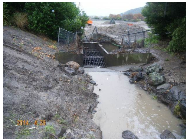
Figure 25 Bridle Path valley waterway - Inlet structure at south end of former malt works site
