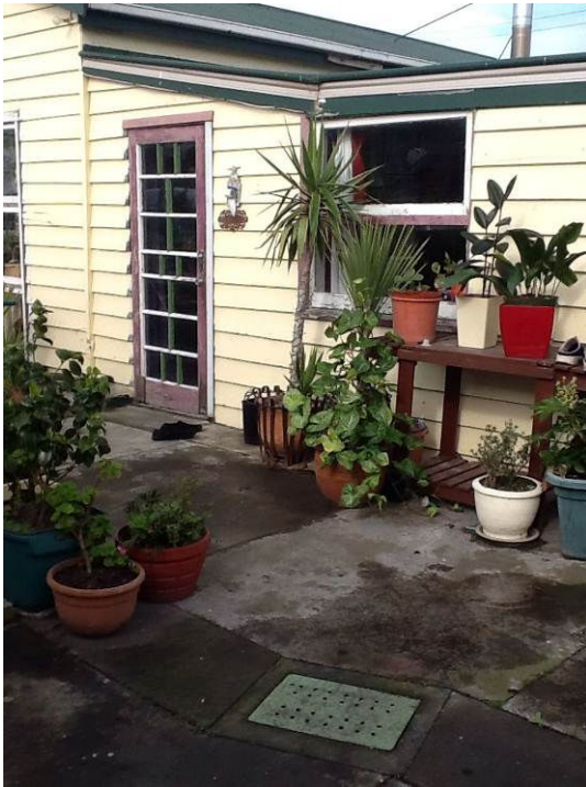
Figure 31 Photo of private grate that surcharges and enters nearby doorway due to lack of flow path away from building and freeboard above the adjacent paving
