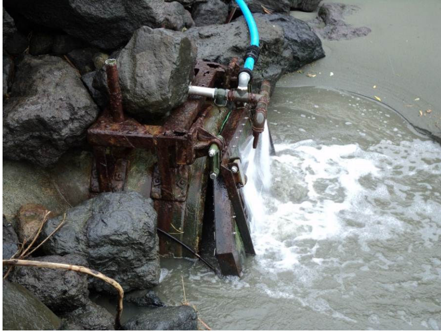
Figure 40 Cave Rock outfall during March event (flap gate partially open)
