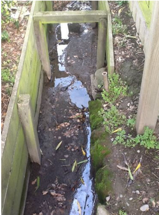
Figure 33 Silt in invert of drain at Okeover Street
