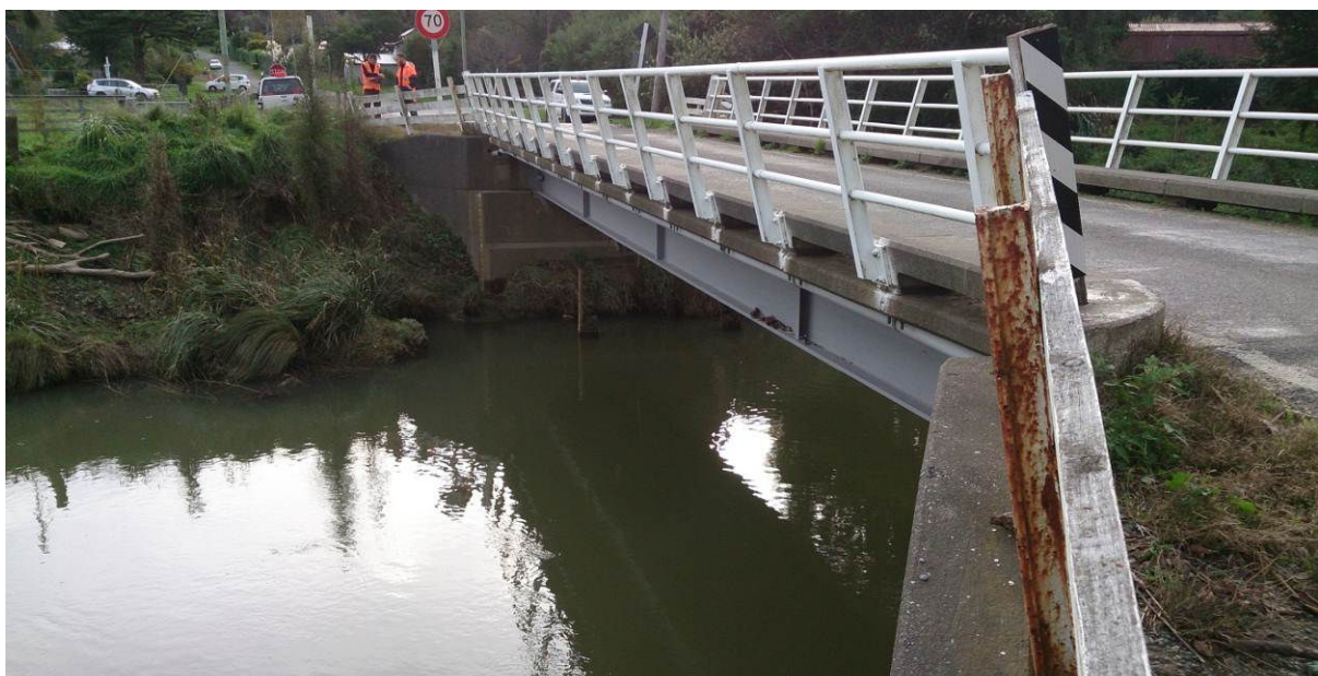
Figure 50 Little River – Wairewa Pa Road Bridge; a key constraint on the network
