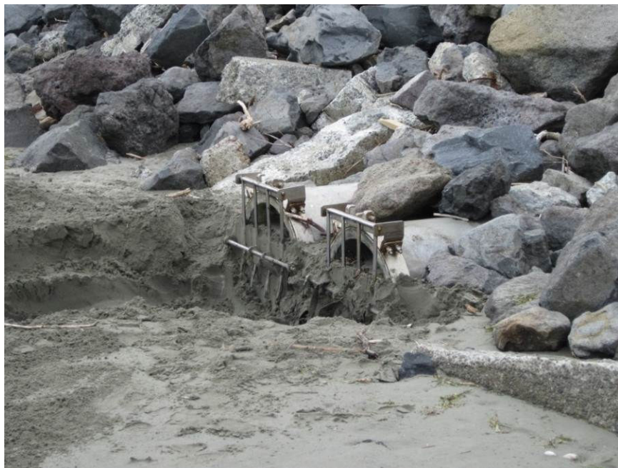
Figure 41 Burgess Street outfalls with sand build-up
