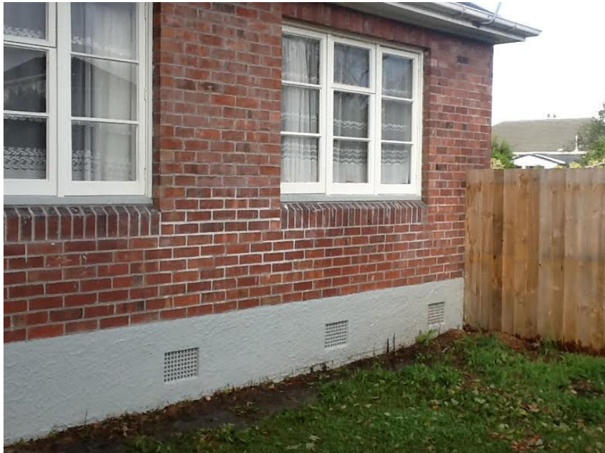
Figure 10 Debris mark showing water level on foundation of Kerrs Road property after March 5th event
