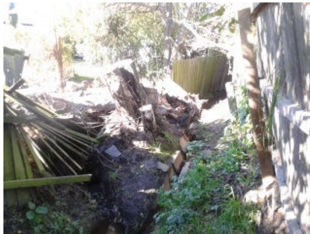
Figure 12 Large constriction in Brittans Drain (since removed)
