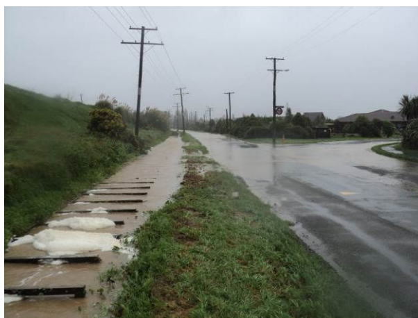
Figure 15 Truscotts Road showing subsidence of timbered drain
