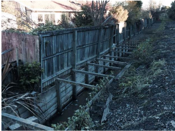
Figure 22 Bridle Path drain west of rail embankment property side timbering to the raised
