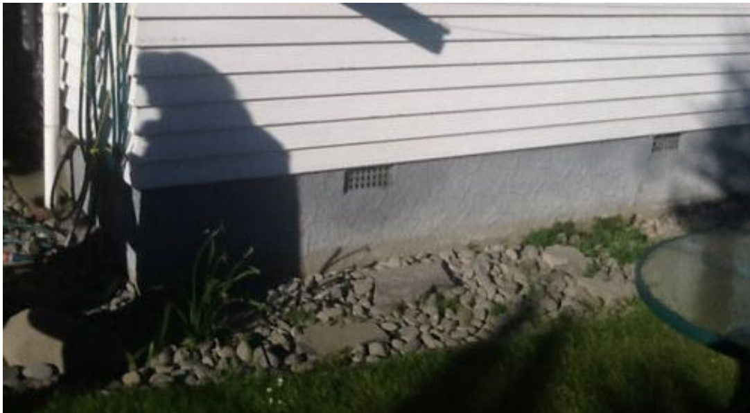
Figure 48: Dalkeith Street house after under floor flooding
