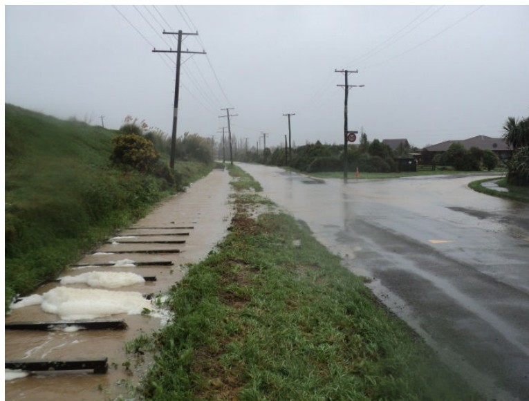
Figure 32 Truscotts Road – Deavoll Place – showing subsidence of timbered drain
