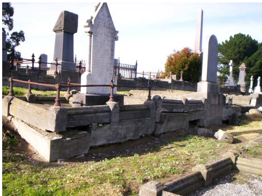
Subsiding grave surrounds, south west part of the hill
