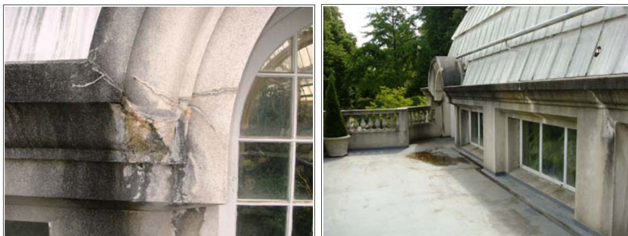
Figure 1.64. Cracks in the plaster and signs of efflorescence and spalling beneath the arch and along the cornice beneath the roofline. Source: DPAL
