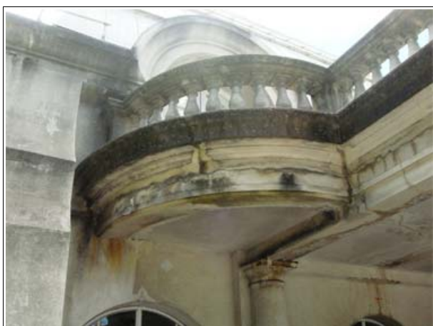
Figure 1.68. Evidence of cracking and moisture on the spandrel of the balcony.
