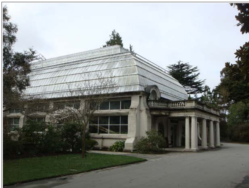
Figure 1.59. Cuninghame House Winter Garden looking towards the front entrance, 2012. The large concrete buttresses can be seen on the side of the building. Source: DPAL
