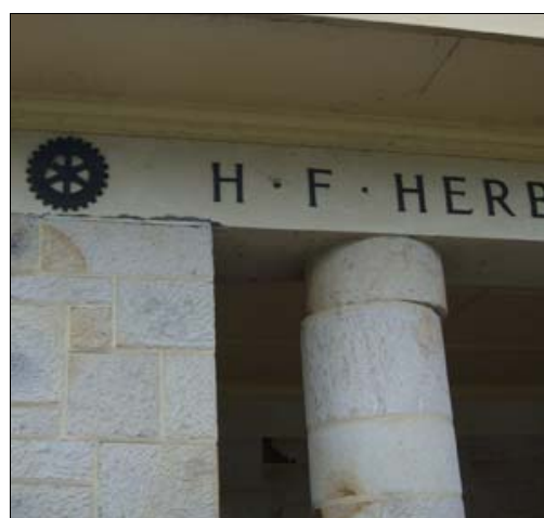
Figure 1.41. Displaced drum columns and cracking. Source: Dave Pearson, July 2012
