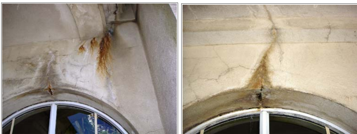
Figure 1.67. Cracks and signs efflorescence and rust stains above windows on the ground floor portico.
