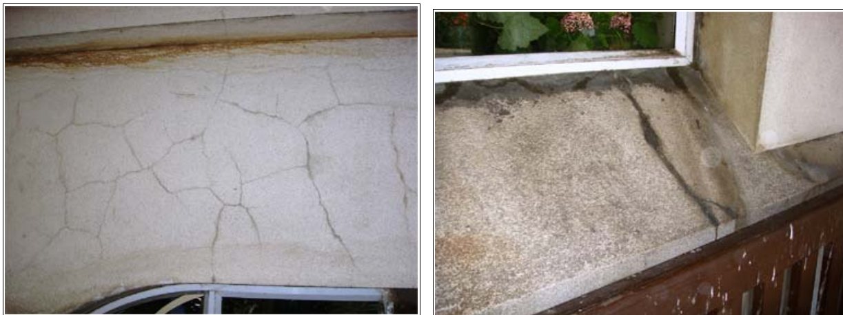
Figure 1.66. Crazing of the plaster work on ground floor verandah wall (left) and cracks in the window sill (right).
