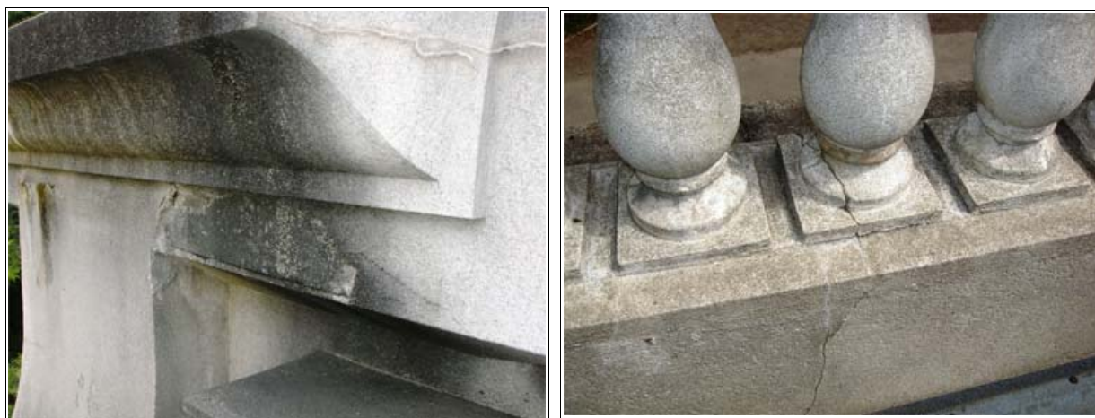
Figure 1.65. Plaster spalling (left) and cracks in the balustrade (right). Source: DPAL
