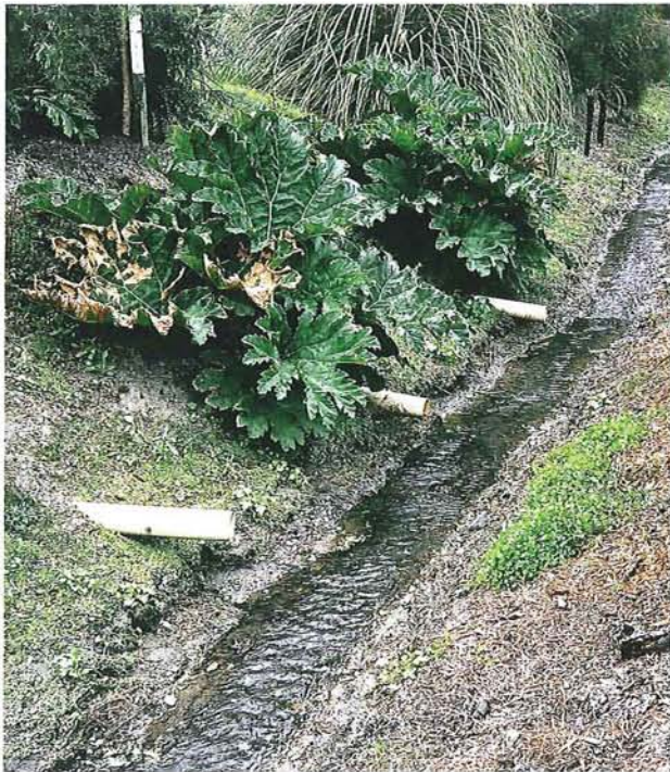
Figure 9-16: Outfalls extending past the stream bank (as above) in new waterways illustrates a lack of consideration for waterway values, and is unacceptable.
