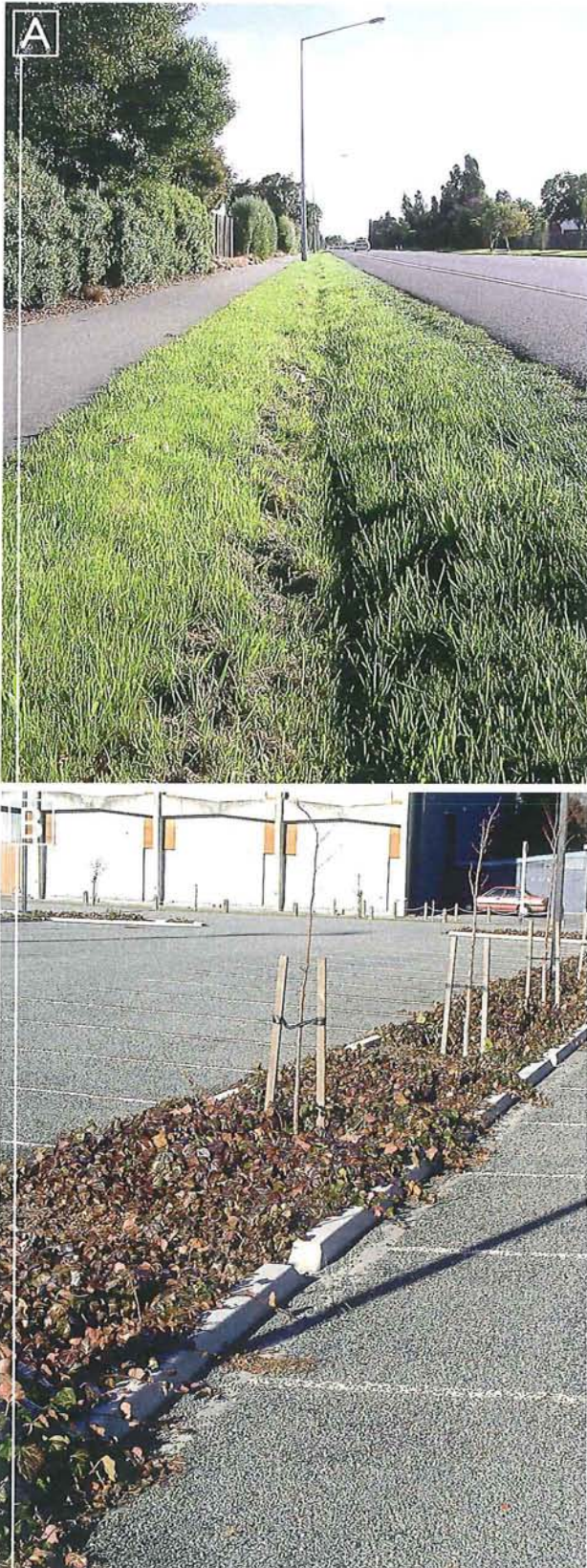
Figure 5-1A: Grassed swales primarily convey stormwater, but have significant water quality and quantity benefits. Grassed swale alongside QEII Drive.
