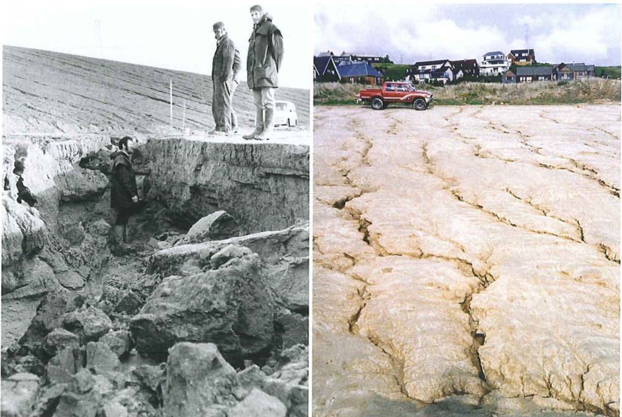
Figure 4-5: The urban development of Westmoreland caused severe ongoing problems with deep erosion of loess soils from the 1970's (above left) to the 1990's (above right).
