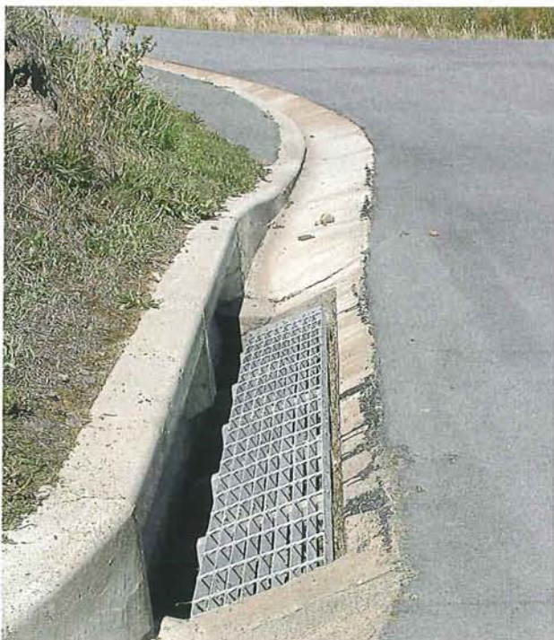
Figure 14-3: The design of hillside sumps requires special consideration to ensure the capture of adequate channel flow during stormflow conditions.
