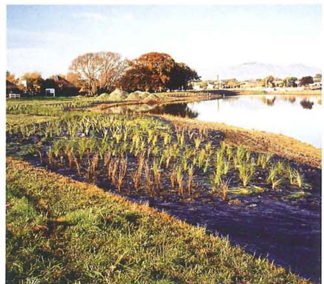
Figure 11-7: Weed mats can prevent the growth of weeds and protect the otherwise exposed soil while plants are becoming established. Barkers Waterway on Anzac Drive.
