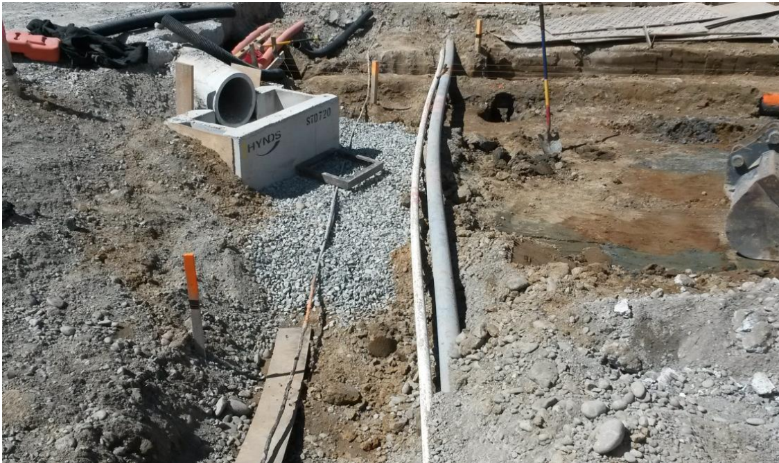
Figure 32 Construct Overflow structures if needed. Ensure services are identified and protected appropriately.
