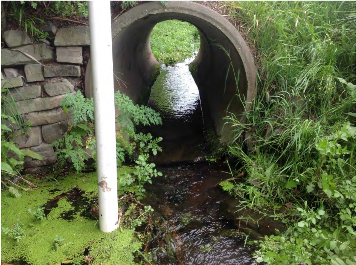
P5: Culvert on lower Henderson Waterway, has potential to be a barrier in both high and low flows.
