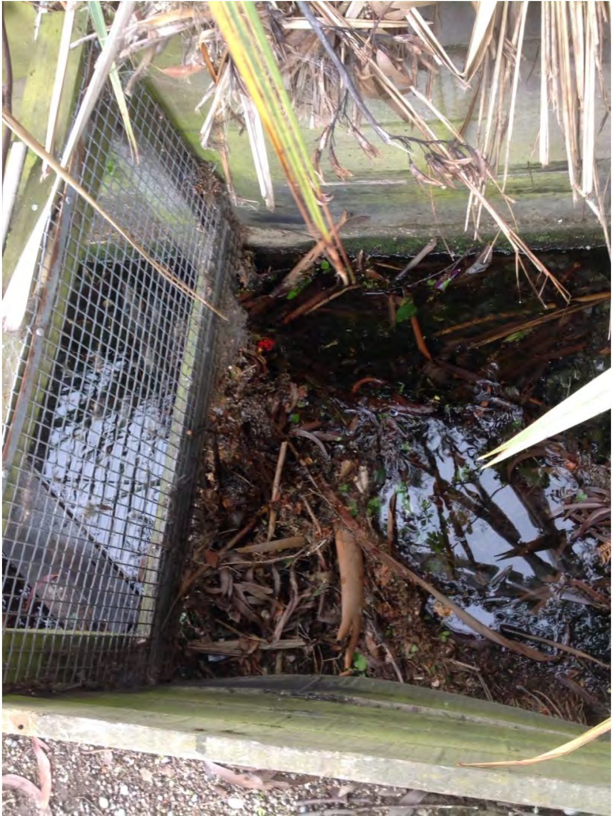
P1: Debris gate does not reach below water level, but could be a barrier to fish passage when debris builds up.
