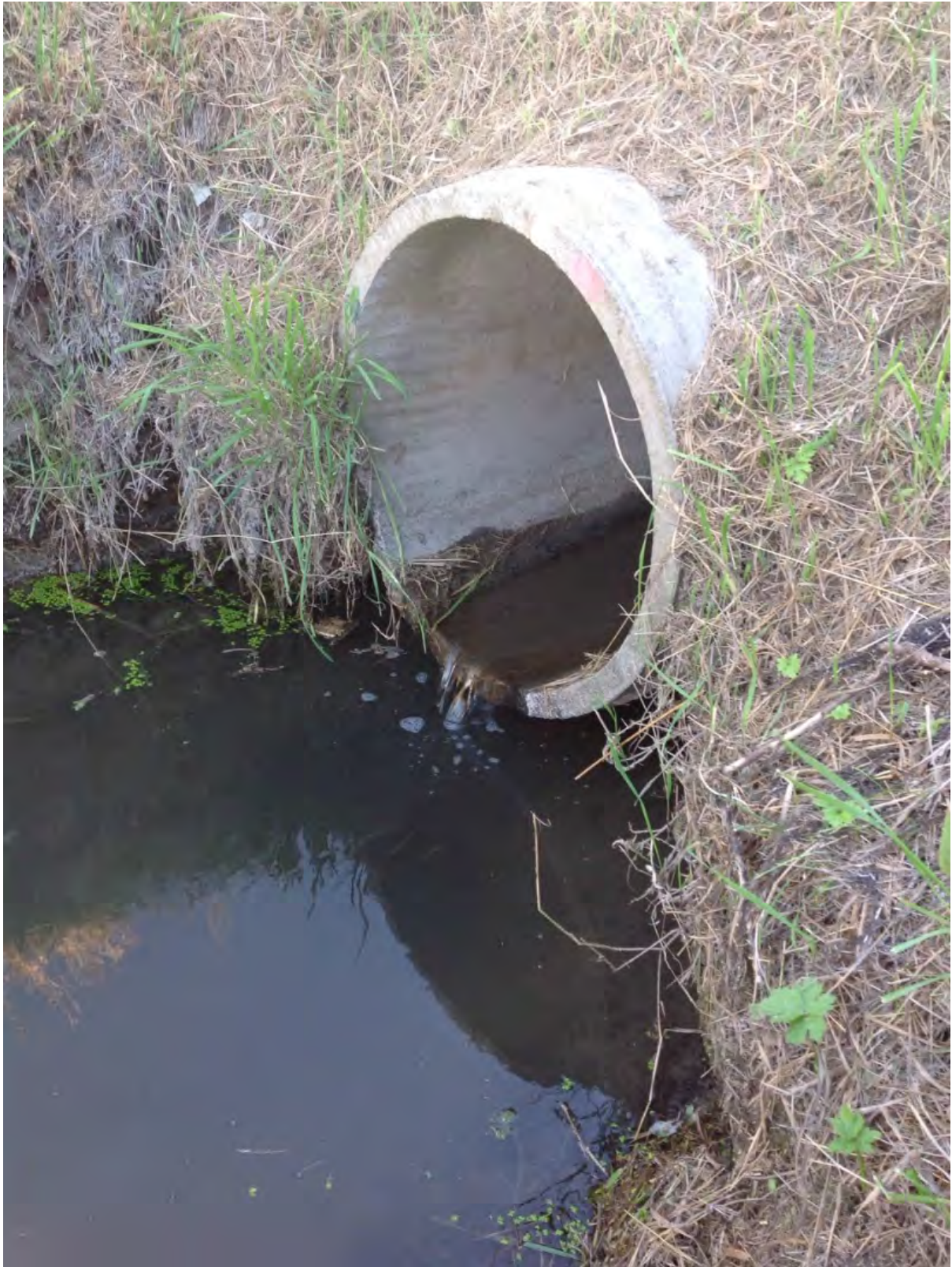
A4: Perched culvert along Dunbar Waterway, downstream of Sparks Road, upstream of Site 2.
