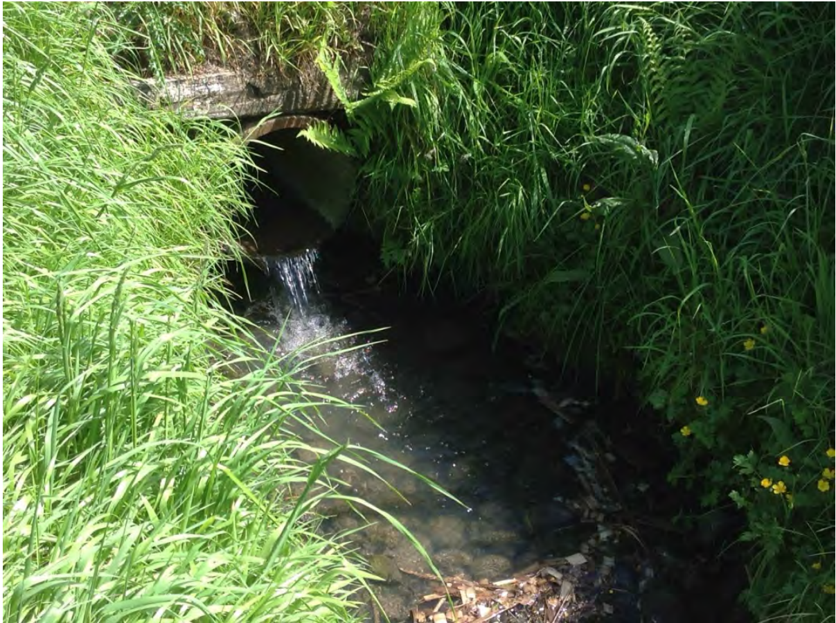
A2: Perched culvert along Dunbar waterway.
