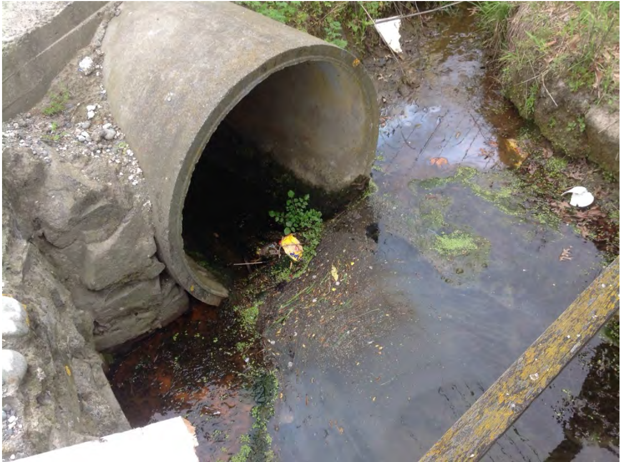
P4: Road culvert, upstream of Sparks Road, may collect woody debris and litter, which may be a barrier to fish passage.
