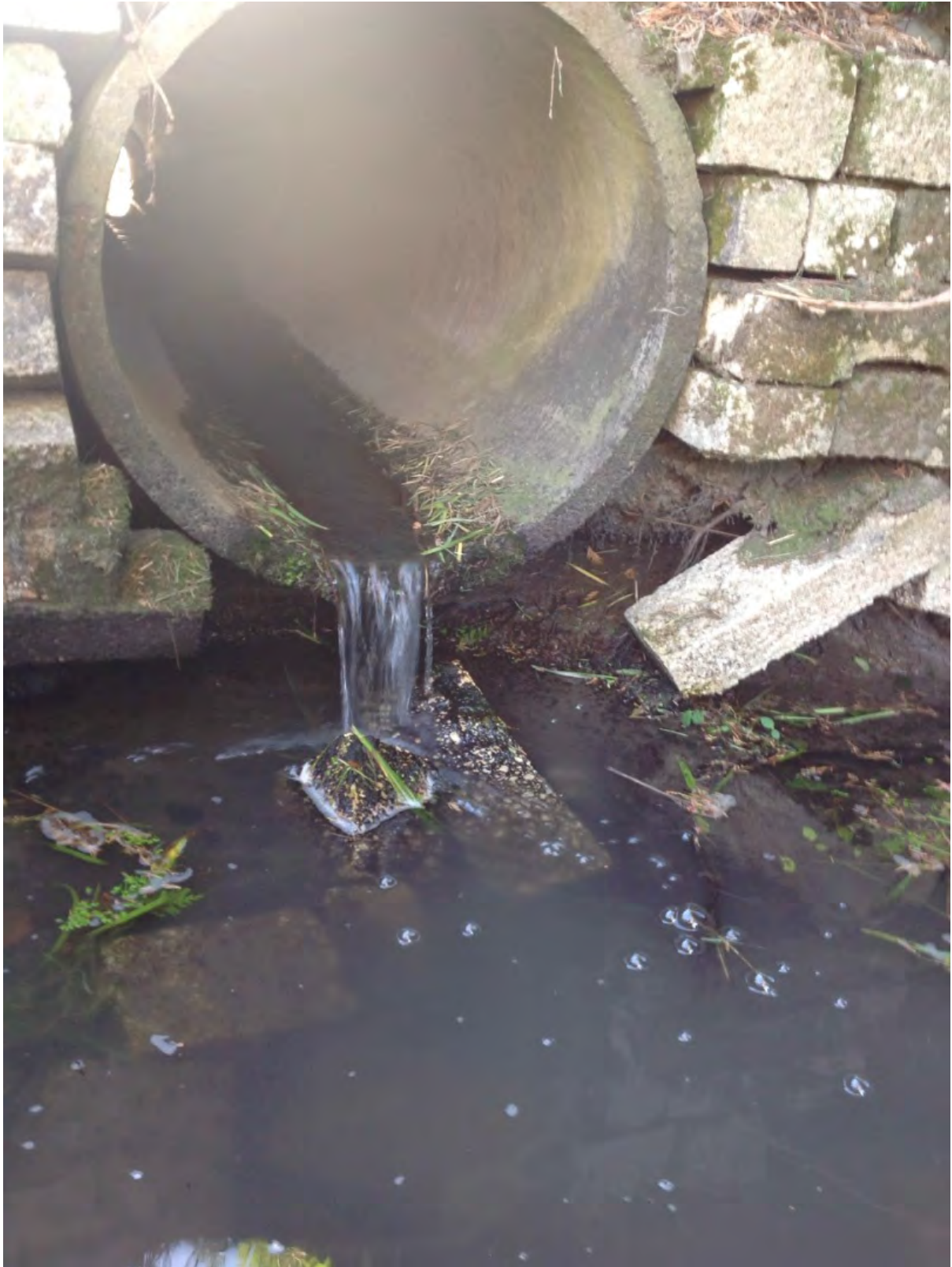
A3: Perched culvert along Dunbar Waterway, at Sparks Road, upstream of Site 2.
