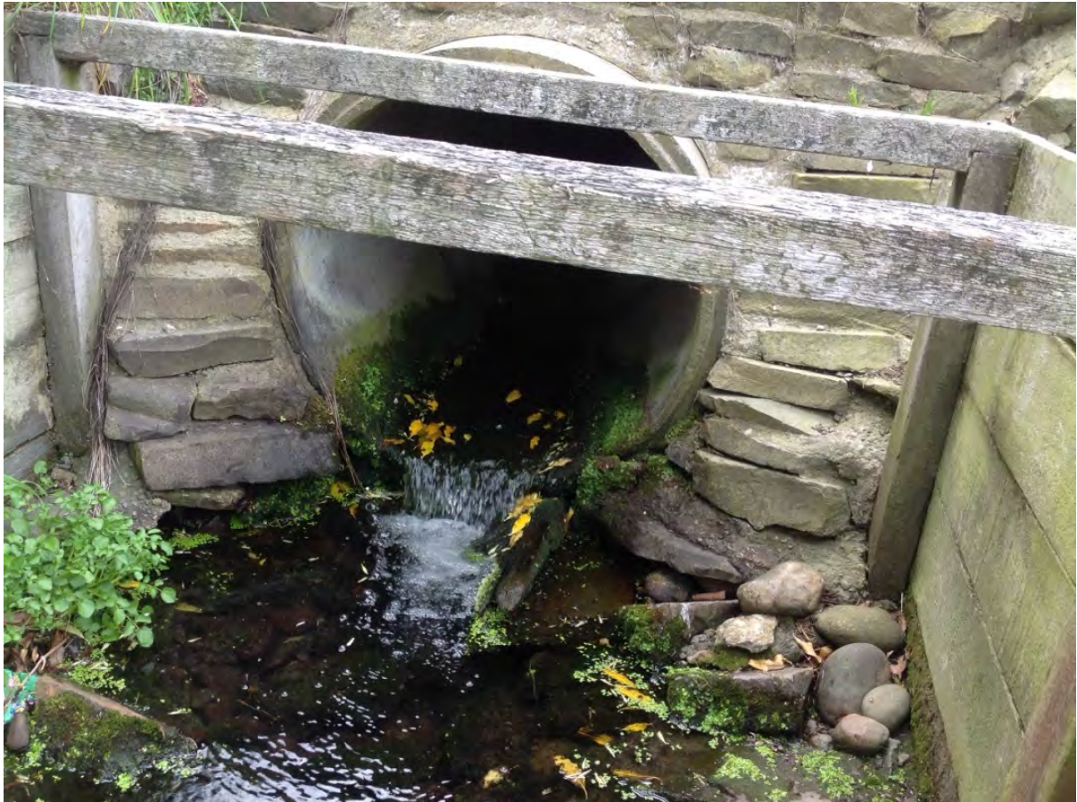
A1: Perched culvert under driveway, Henderson Waterway, 150 m upstream of Site 6; Inanga observed in pool below culvert.
