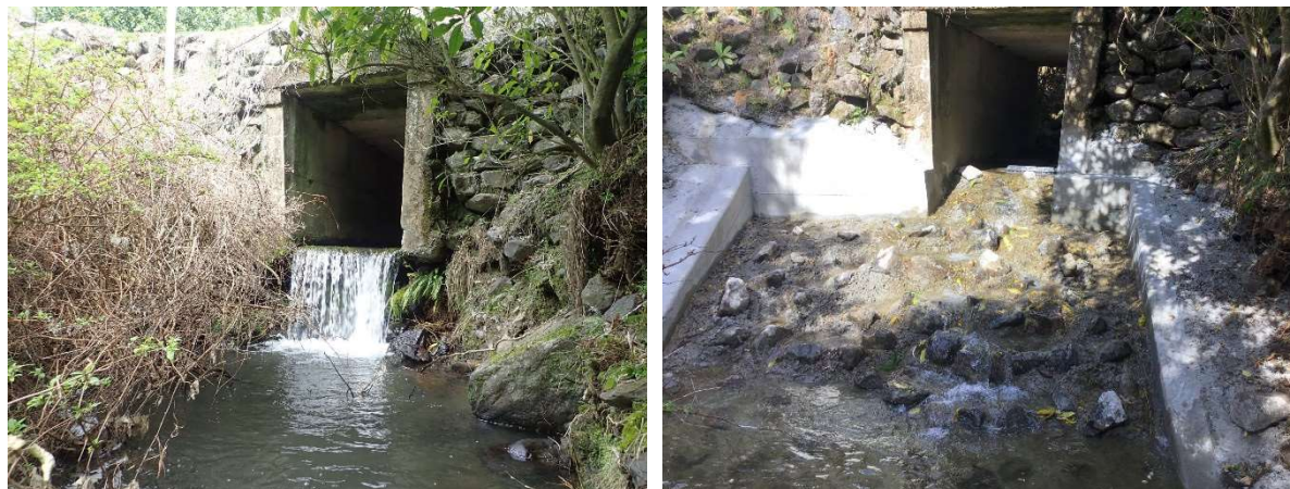
Figure 11: The perched culvert in Kaituna Valley before (left) and after (right) remediation.
