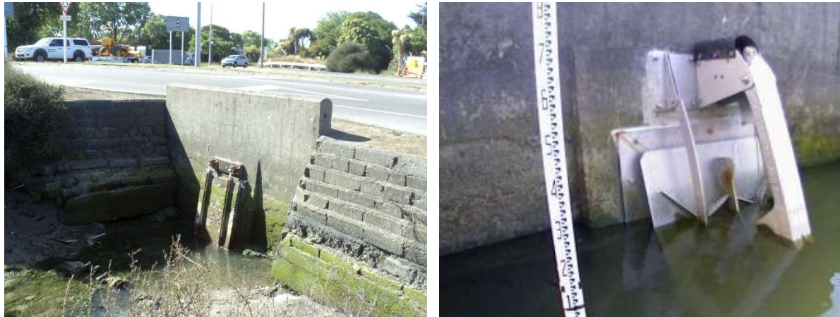
Figure 13: Steamwharf Stream tide gate before (left) and after (right) remediation. The right-side photograph shows the structure on an incoming tide, with the counterweight delaying gate closure.
