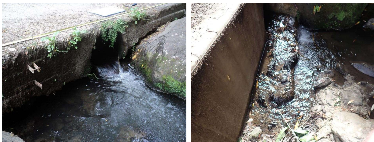
Figure 12: The perched culvert in Hukahuka Turoa Stream before (left) and after remediation (right).
