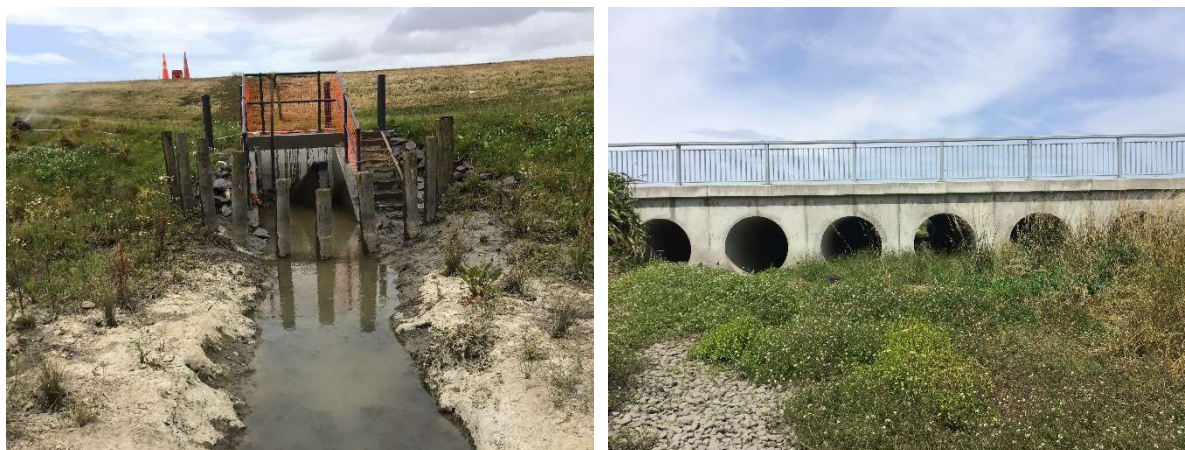
Figure 6: Site 7b (left) and Site 34 (right) were deemed low risk by the assessor but classified as high risk by the FPAT website. The outlet of Site 7b was temporarily sealed to retain water for watering new plants in the stormwater wetlands, but was assessed as if the seal was absent.
