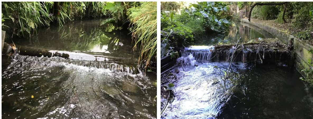
Figure 5: A low wooden weir (Site 19, left) presents less of a barrier to fish than a taller weir (Site 17, right), but both were assigned a very high risk to fish passage by the FPAT website. In the assessor's opinion, the low weir represented a medium risk, while they agreed that the taller weir presented a very high risk to fish passage.
