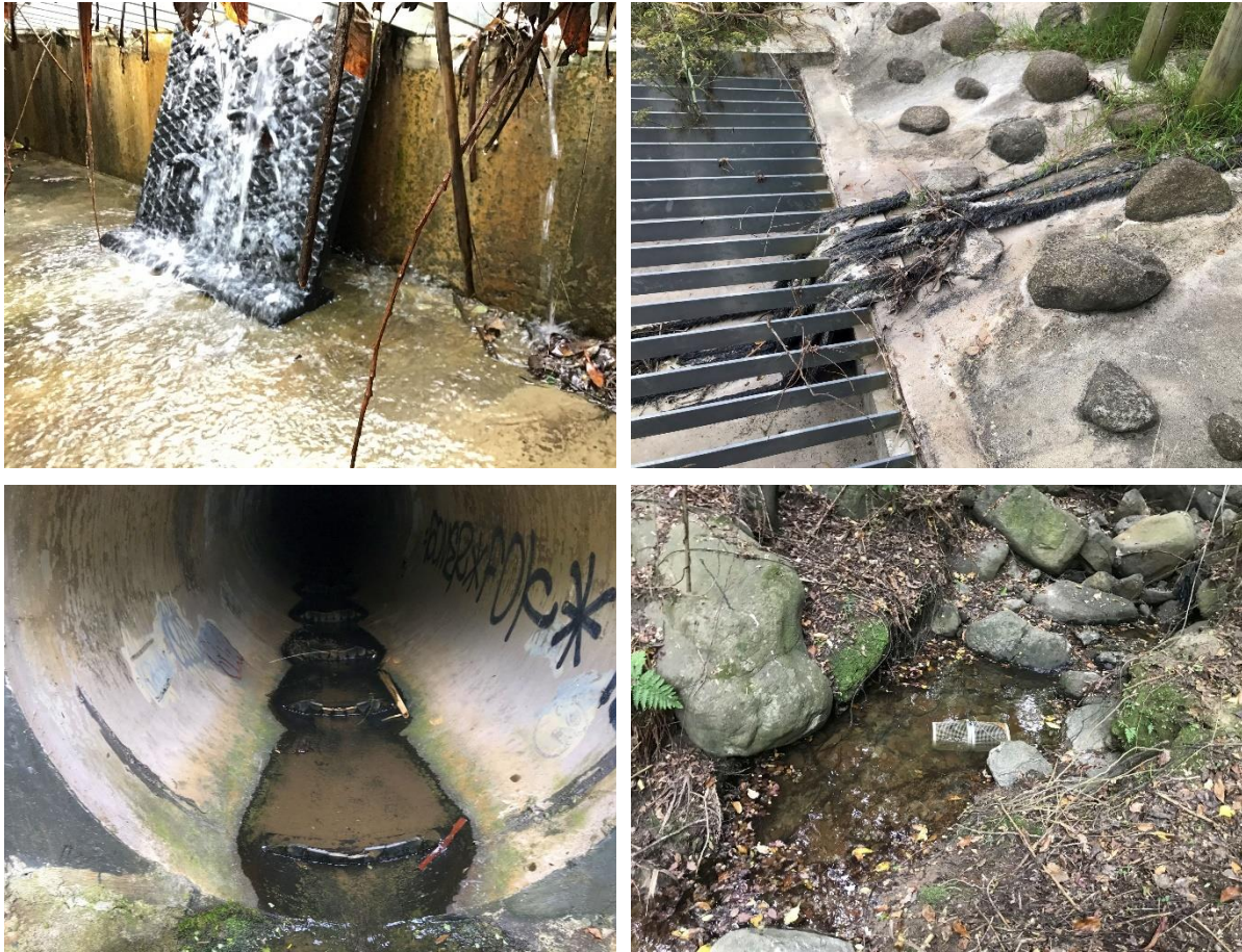
Figure 9: The weir structure and steep fish ramp during the associated FPAT assessment (top left), the structure during the fish survey (note the addition of mussel spat rope; top right), the culvert downstream under Harbour View Tce which includes baffles increasing water depth (bottom left), and an example of the habitat in the Upstream 1 sampling reach.
