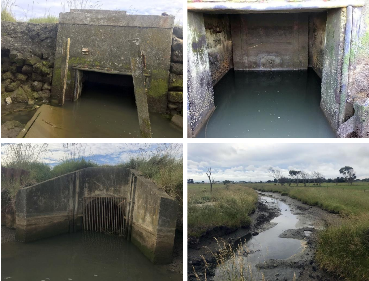
Figure 6: Charlesworth Reserve Drain downstream view of culvert and flap gate externally (top left) and internally (top right). Upstream end of structure (bottom left) and upstream sampling reach (bottom right).
