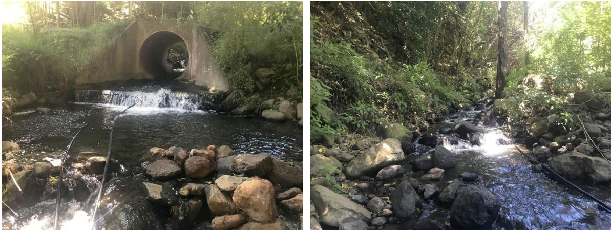
Figure 14: Owhetoro Stream Branch No. 4 culvert with perched apron (left) and the upstream sampling site (right).
