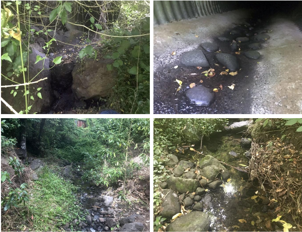
Figure 11: The perched apron at the downstream end of the culvert (top left), rocks imbedded through the culvert to enhance fish passage (top right), the Downstream 1 sampling reach, and one of the sampled pools upstream of the culvert (bottom right).
