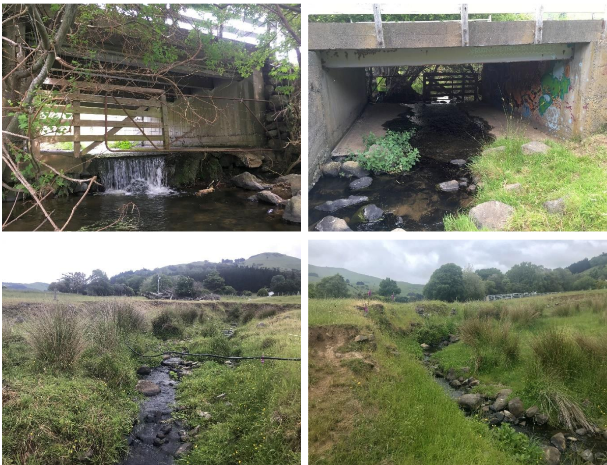
Figure 15: Totara Stream culvert with perched apron (top left), upstream view showing shallow water depth through the culvert (top right), downstream sampling site (bottom left), and upstream sampling site (bottom right).
