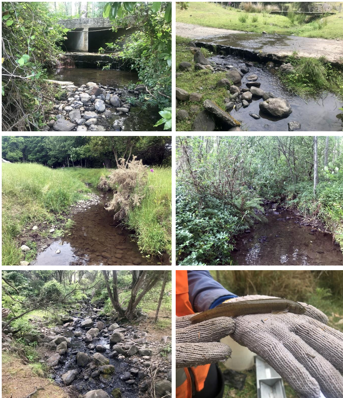
Figure 18: Culvert with perched apron in Kinloch Stream (top left), upstream ford with culvert (top right), and Downstream 1 (mid left), Upstream 1 (mid right), and Upstream 2 sampling sites (bottom left). Kōaro caught at Upstream 2 site (bottom right).
