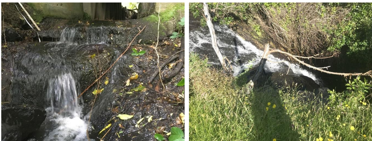
Figure 13: The perched culvert outlet (left) and the 6 m high vertical waterfall located 40 m downstream from the culvert (right). Note that this photograph only captures the entry to the waterfall, not the vertical face, as this could not be photographed safely.
