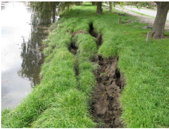
Figure 11a. The deep cracks formed by a bank section suffering particularly severe lateral spread at the Avondale site.
