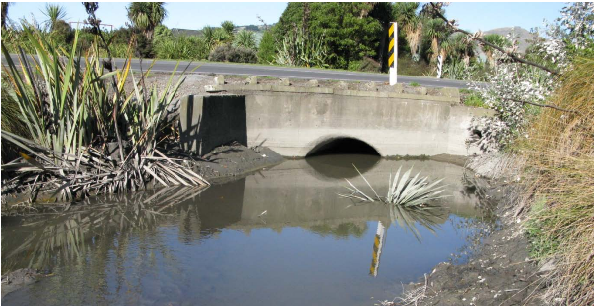
Figure 8b. Steamwharf Stream, looking downstream at Dyers Road. The disruption to the bed is evident here with flaxes on the banks slumped and collapsed into the channel.
