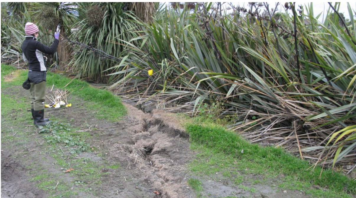
Figure 16. Both lateral spread and uplift on the eastern site of Lake Kate Sheppard. However, the esplanade has also been subject to compaction by heavy-construction vehicles.
