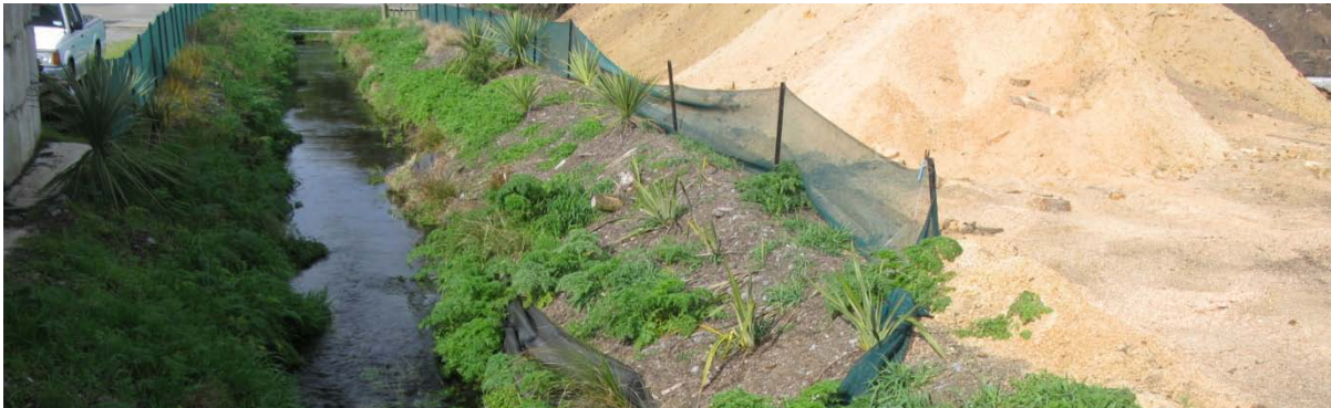
Figure 19b. Photo 2 Sept 2010. Recent riparian fencing and planting to prevent sawdust from entering Smacks Creek. Some improvement to the riparian fencing and sparse planting on the (true) right bank would be beneficial to instream habitat by intercepting loose wood chip material.
