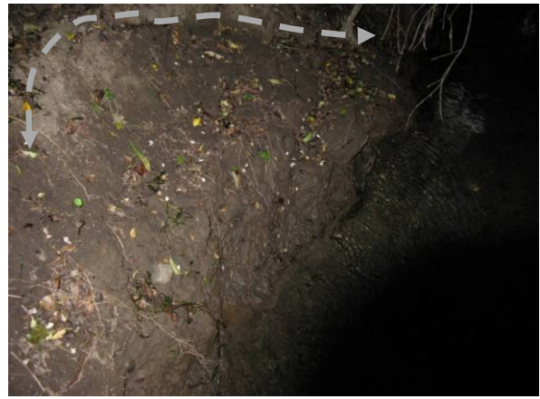
Figure 32d. 8/9/10, slumping on the true right bank, probably due to seismic activity on the 4 th September 2010.
