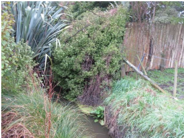
Figure 32c. The same site 8 September 2010, this photo left bank was subject to significant lateral spread from the 4 September 2010 earthquake.
