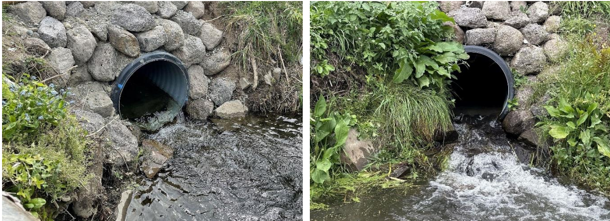
Figure 3: Downstream end of Cashmere Stream culvert at Sutherlands Road, in October 2022 (left) and March 2023 (right), when water levels were lower and the FPAT assessment was made.
