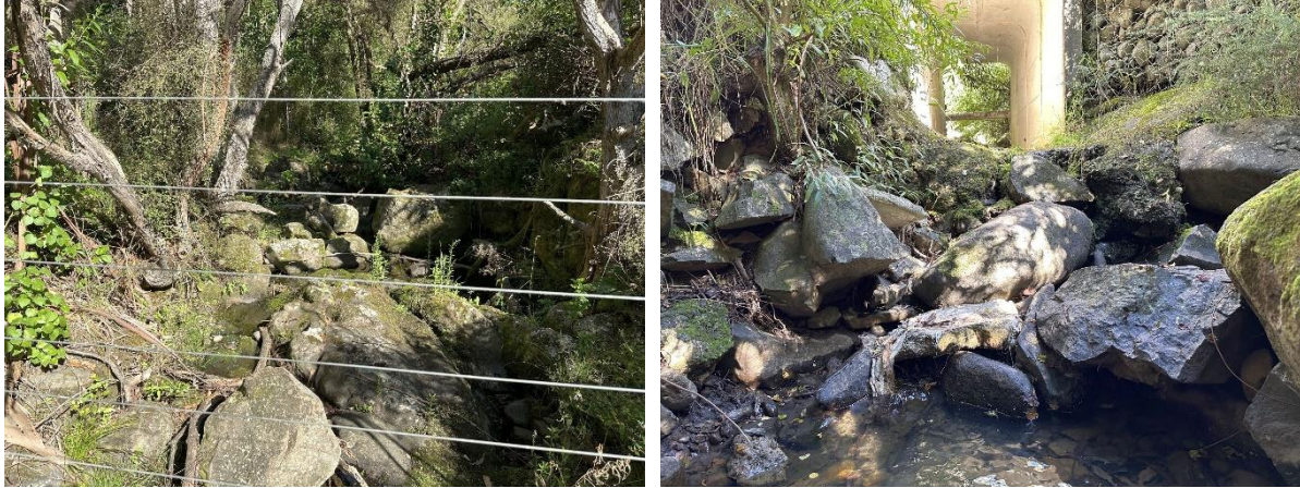
Figure 1: Church Gully Stream upstream of the road culvert (left) and immediately downstream of the culvert (right), showing the perched apron.
