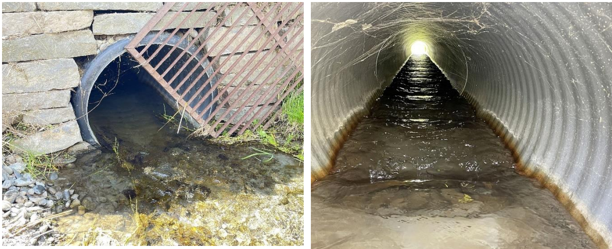
Figure 4: Upstream end of Sutherlands Road culvert in March 2023, showing the inlet (left) and weir baffles (right).
