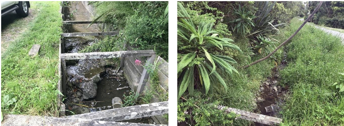
Figure 5: Site 5 (Mt Pleasant Waterway), showing minnow traps set in pools located in the broken concrete lining (left) and in a section with natural lining (right).
