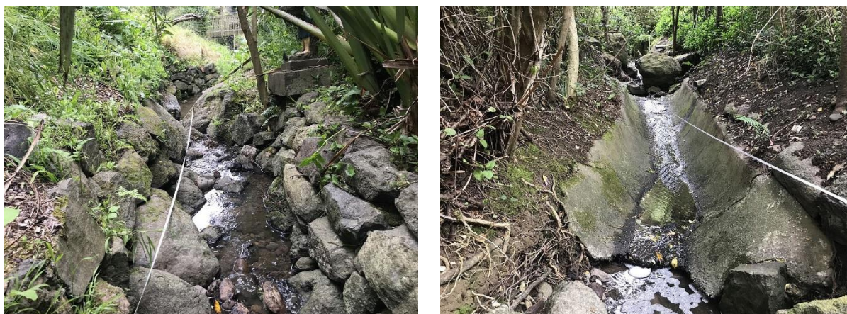
Figure 9: Site 11 (Patchetts Drain), showing sections of waterway with natural stone rock lining (left) and concrete lining (right).
