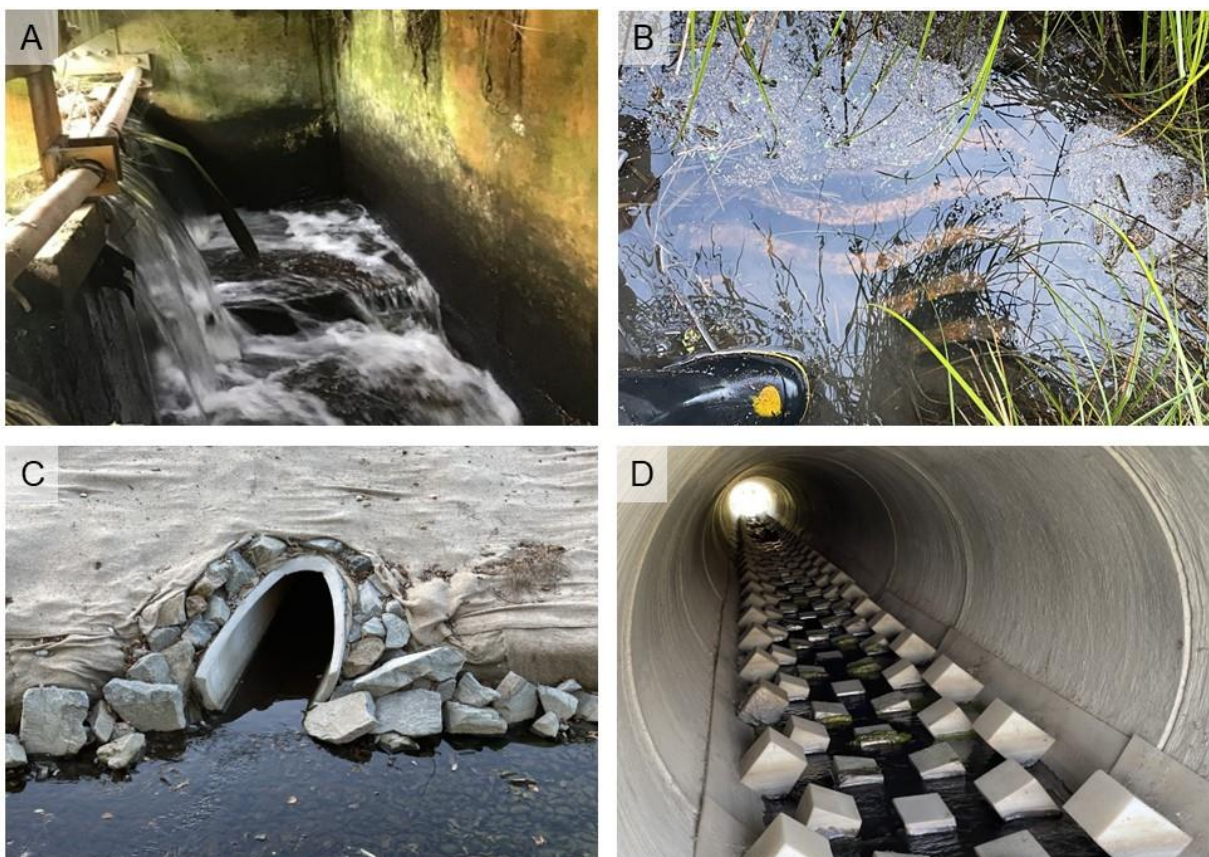
Figure 7: Examples of structures assessed for fish passage risk at the wetlands sampled. These include a very high-risk structure at A) Site 16 (Arthur Adcock), a medium-risk structure at B) Site 18 (Douglas Clifford), and low risk structures at C) Site 21 (Te Oranga Waikura) and D) Site 13 (Burlington).
