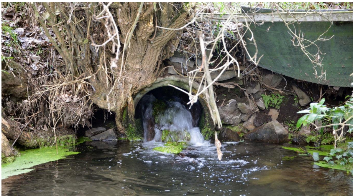
Figure 6: Sutherland Road culvert. Photograph taken on 14 July 2016 following recent rain.
