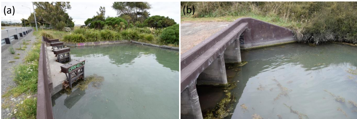
Figure 7. Linwood Canal outlet structure at the Avon Heathcote Estuary Ihutai on Humphrey’s Drive. (a) View of the four flap-gates in operation on a high tide. (b) Tidal ingress into Linwood Canal through the southern culvert on an incoming tide.
