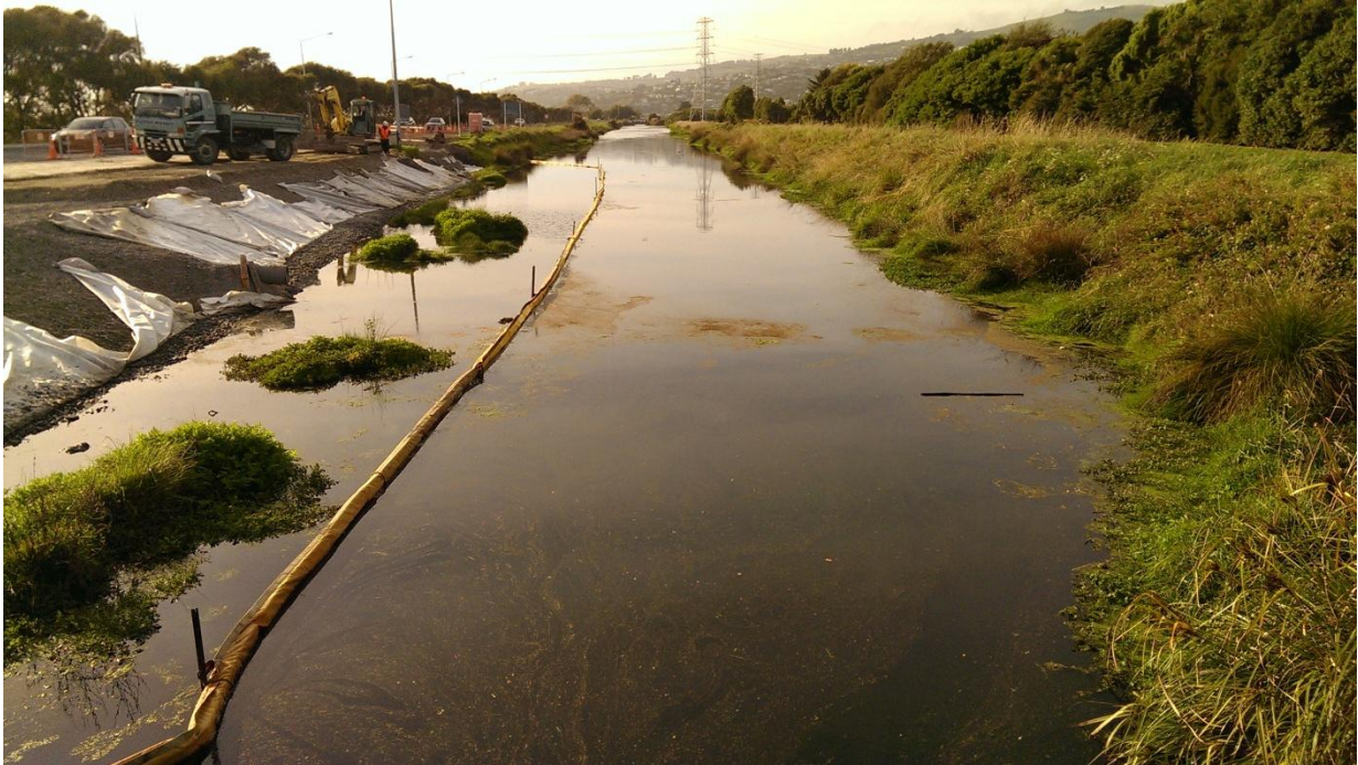
Figure 2. Linwood Canal looking downstream from Dyers Road showing current road works in the riparian zone. A silt curtain can be seen protecting the waterway from construction site run-off.
