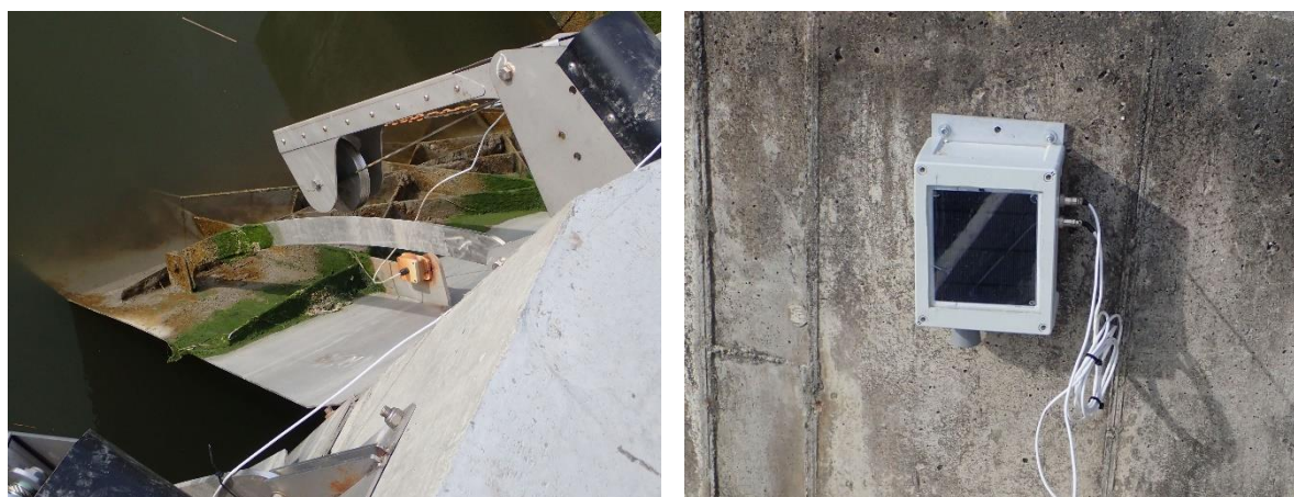
Figure 7: Gate monitoring accelerometer (left) and water level recording (right) at Avoca Valley Stream tide gates.
