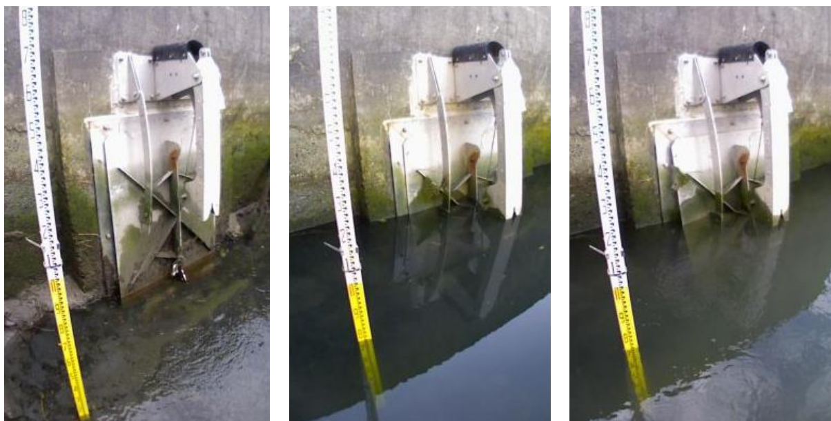
Figure 12: Steamwharf Stream tide gate with the counterweight temporarily disengaged. The left and middle photographs are on an incoming tide, while the right photograph is on an outgoing tide.
