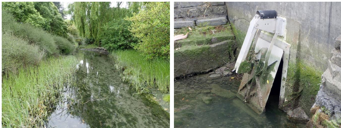
Figure 3: Steamwharf Stream (left) and its fish-friendly tide gate (right).
