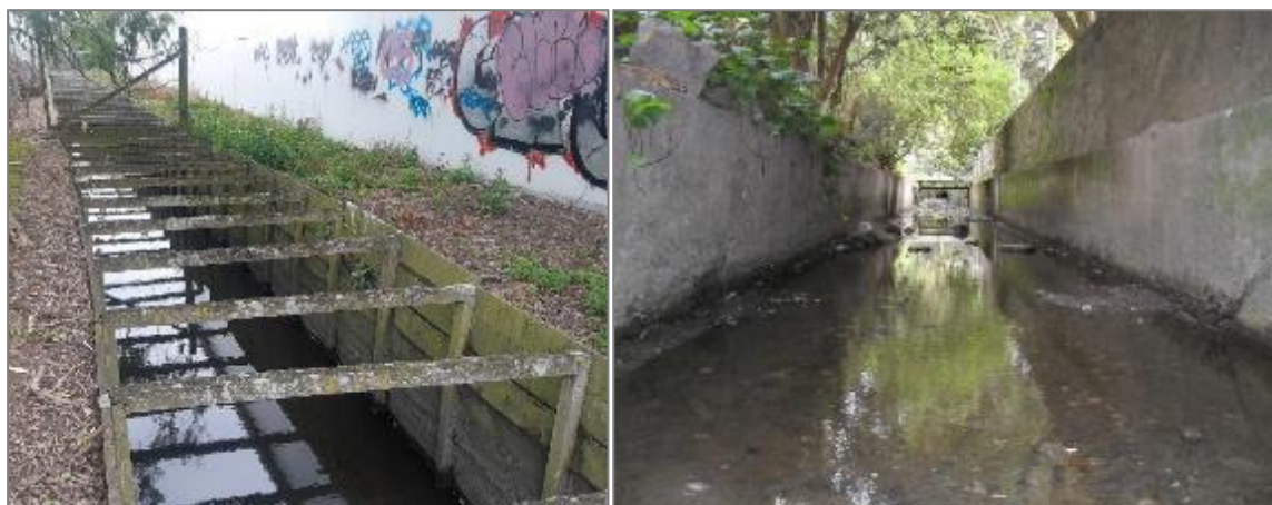
Figure 2-4: Lined streams in Ōtautahi City, demonstrating minimal habitat variability. Left: Timber-lined section of Curlett Stream upstream of the motorway. Photo credit M. Flanagan (NIWA). Right: concrete-lined section of Sumner Stream at Scarborough Beach, photo from Allan et al. (2012).
