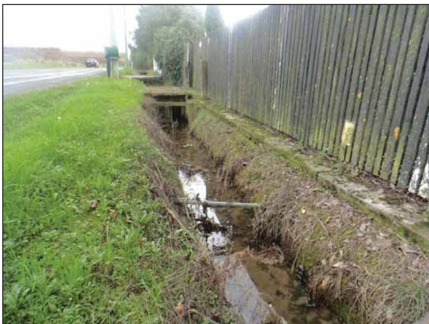
Figure 4: Viewing northwest along the north side of Radcliffe Road. The drain in on a slightly raised embankment, invert is approximately 0.5 metre deep below existing ground level, and is timber-lined and strutted to provide access to properties.
