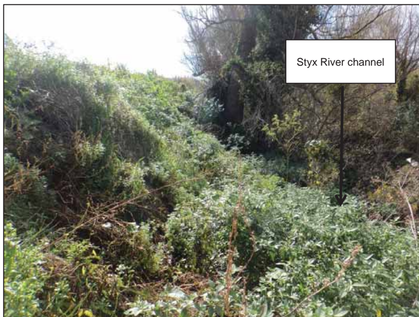
Figure 7: The steep Styx riverbank geometry at Point 3. Similar steep geometries were observed at Points 2, 4, 5 and 8.
