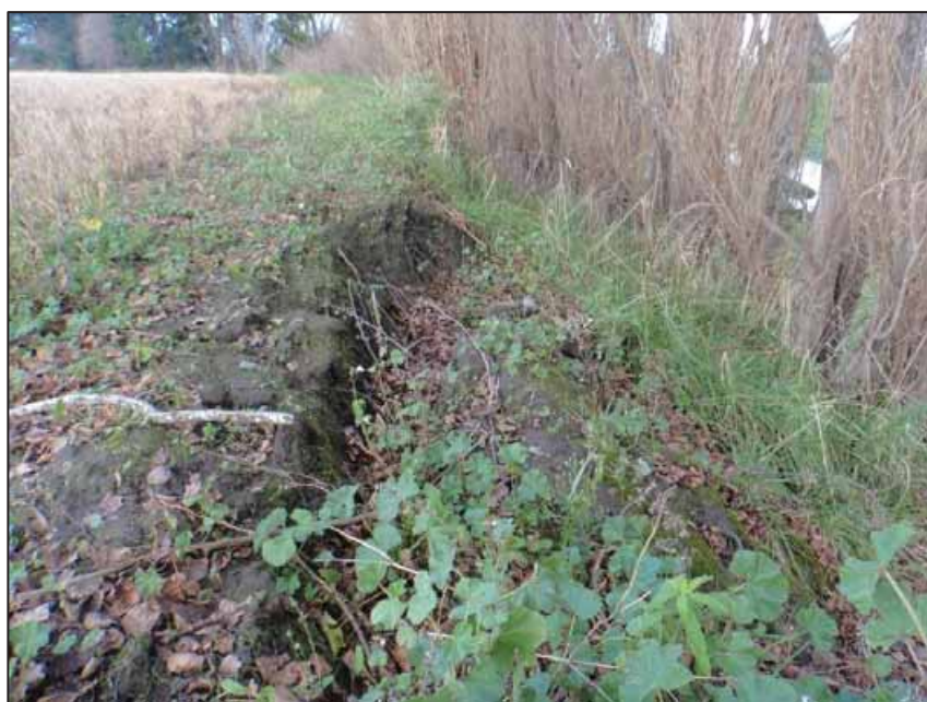
Figure 10: Slope instability along the Styx River channel at the boundary of the SE and SW Areas
