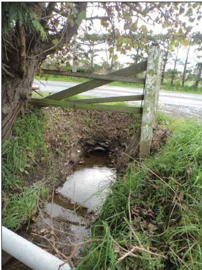
Figure 3: Viewing north along drain where it flows underneath Radcliffe Road at the entrance to 120 Radcliffe Road property. The drain invert is approximately 1 metre deep below existing ground level.
