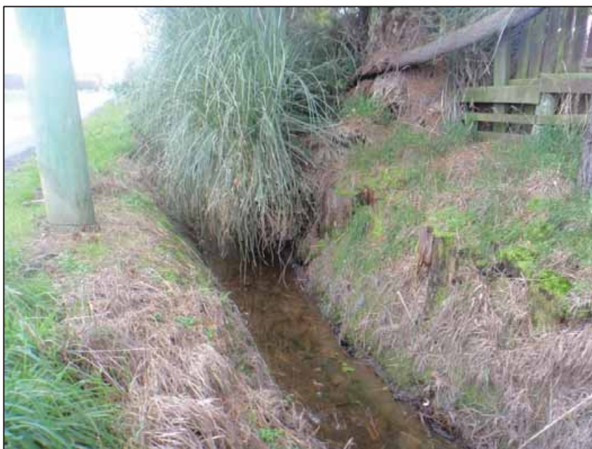
Figure 5: Viewing northwest along north side of Radcliffe Road. The drain invert is approximately 1 metre deep below existing ground level.
