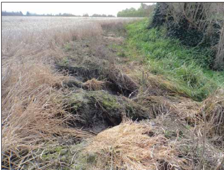
Figure 12: Erosion feature in the SE Area (refer to Figure 6 for the approximate location of this feature).
