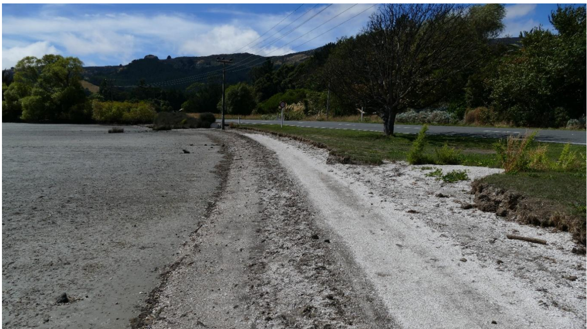
Figure G18 Eroding bank in southern area of Charteris Bay (Area A of Figure G16)
