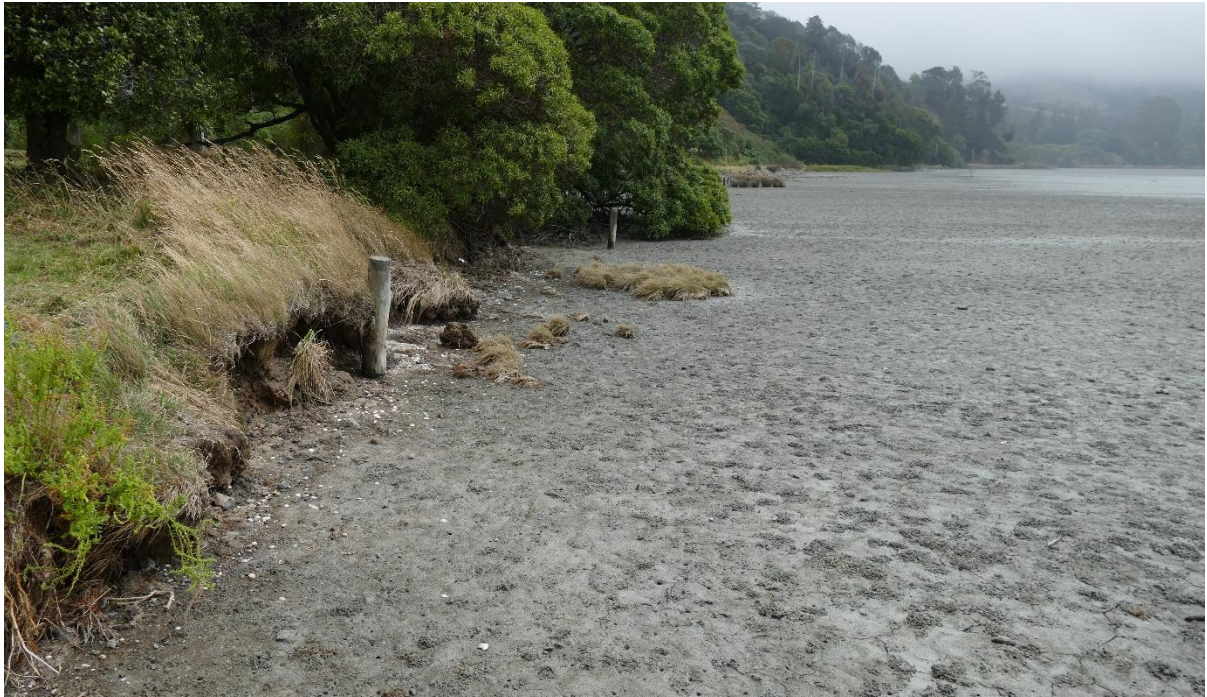
Figure G12 Allandale foreshore between the two streams showing a steep bank with some evidence of erosion and a flat muddy/sandy intertidal area
