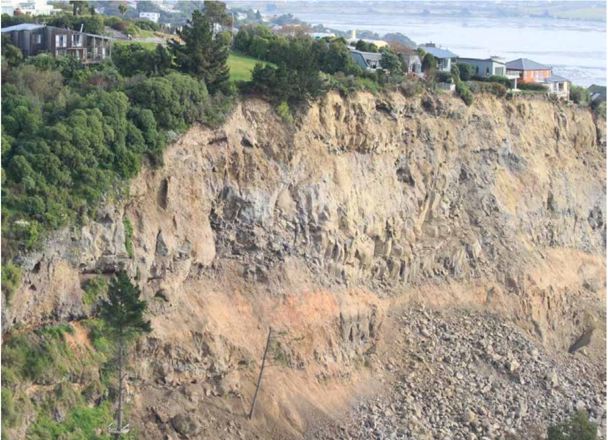
Figure 9 Aerial view of the Redcliffs rock slope after the 13 June 2011 earthquakes. Photograph taken by C. Massey.
