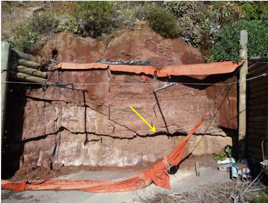
Figure 8 Earthquake-induced cracking in volcanic tuff with post-earthquake movement shown along a zone of discontinuous soft clay within a laterally persistent sub-horizontal discontinuity (yellow arrow). However, it is not known whether these displacements were only in response to the 22 February 2011 earthquakes, or include displacements in subsequent earthquakes.
