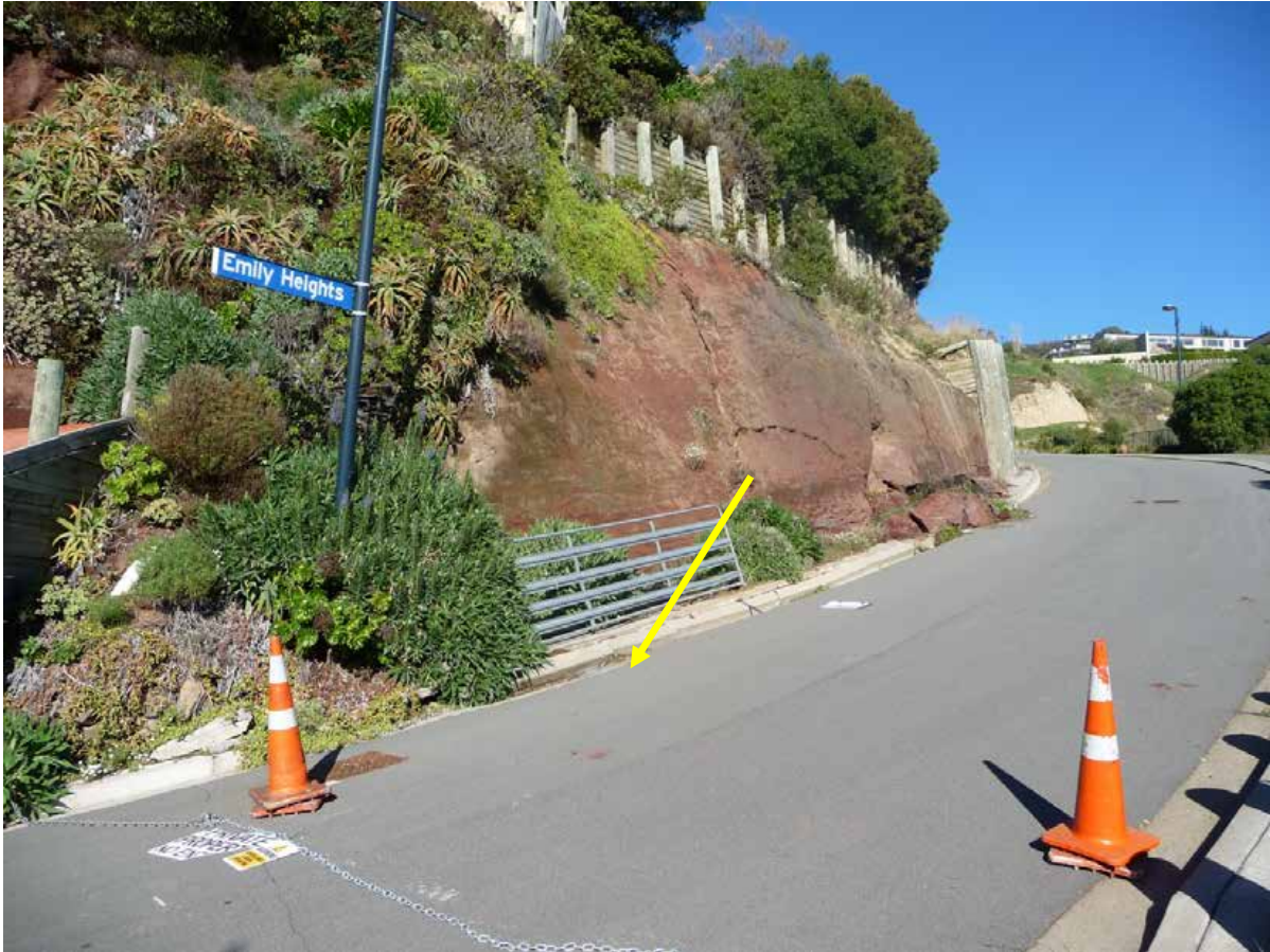
Figure 10 View southeast of the western end of the site. Emily Heights Road is in the foreground. Note the toe break out of the rock slope failure evident along the edge of Emily Heights Road (yellow arrow). This is an extension of the main discontinuities exposed in the car port for 12 Cliff Street (Figure 3).
