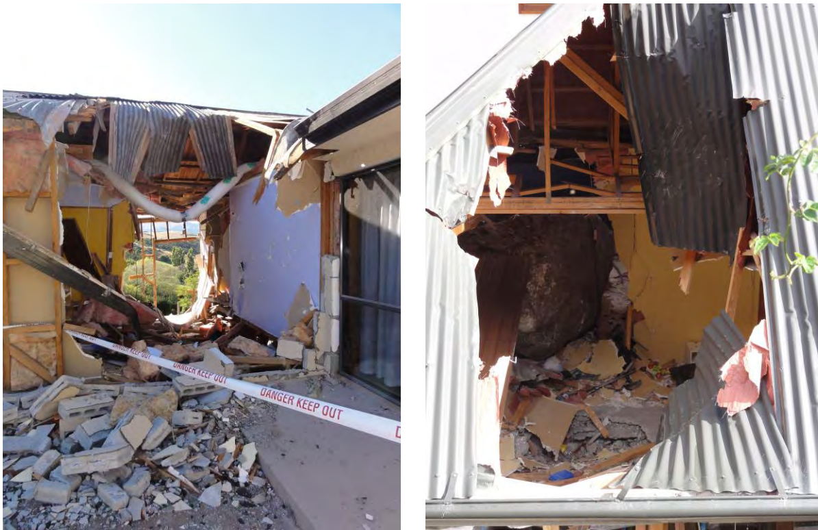
Figure 1 Rockfall damage to residential homes, A) Rapaki Bay and B) Morgan's Valley, Heathcote. This rockfall damage occurred in the main 22 nd February 2011 earthquake.
