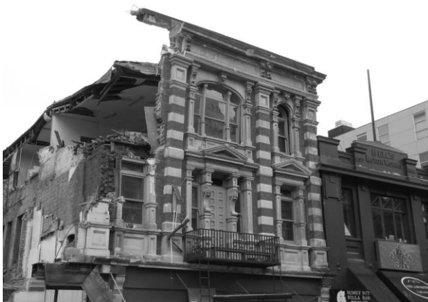
After the June 2011 aftershock, this commercial building on the corner of Manchester and Lichfield Streets was clearly damaged beyond repair.
