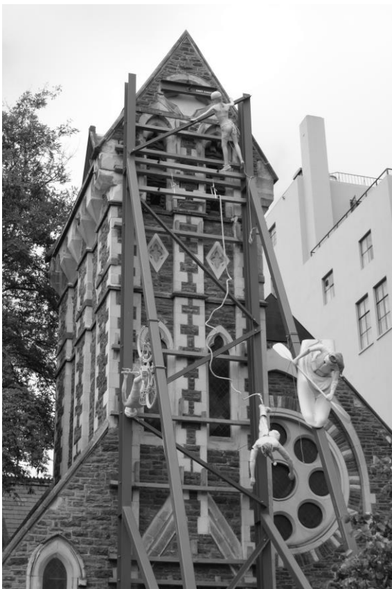
Between the earthquakes of 4 September 2010 and 22 February 2011 several damaged heritage buildings, like the former Trinity Church, were shored up in the expectation they could be repaired.
