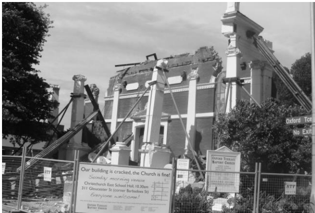
After the 4 September 2010 earthquake, it was thought that the Oxford Terrace Baptist Church could be repaired. After the 22 February 2011 earthquake repair was clearly impossible.
