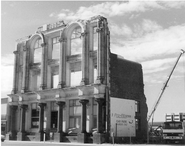
The demolition of the Kaiapoi Woollen Company building in the 1990s was strongly opposed by those concerned about the loss of the city's historic buildings.
