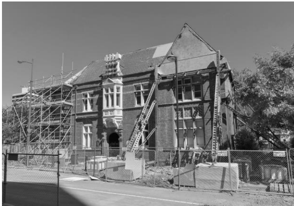
The damaged 1887 City Council Chambers, Our City/O-Tautahi, are to be retained.
