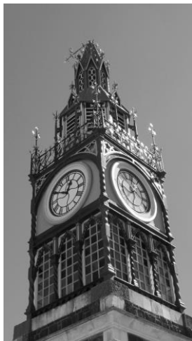
The visible damage to the Victoria Street Clock Tower was minor, but the structure needs extensive repairs following the earthquakes.
