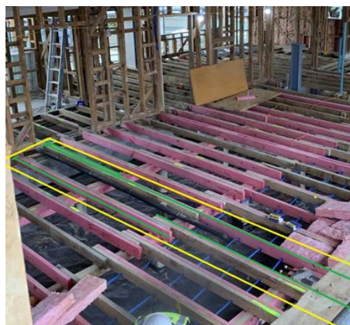
Image 5: - Example recent project showing extend of new framing to floors that may be required.
