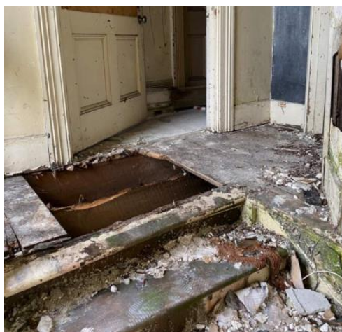
Image 4: Existing Floor Condition
