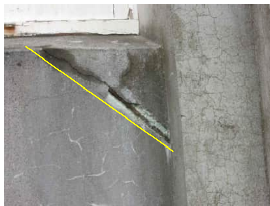
ES13 A-550 | CRACK EXPOSING REINFORCING BELOW SECOND FLOOR WINDOW AT GRID 7
