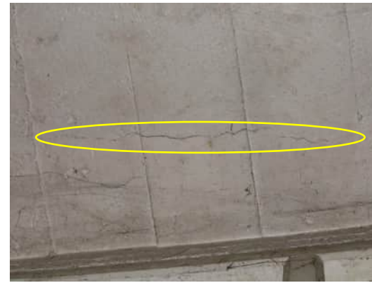
0.62 SIGNIFICANT CRACKS IN THE CEILING NEAR GRID 12/D A-500
