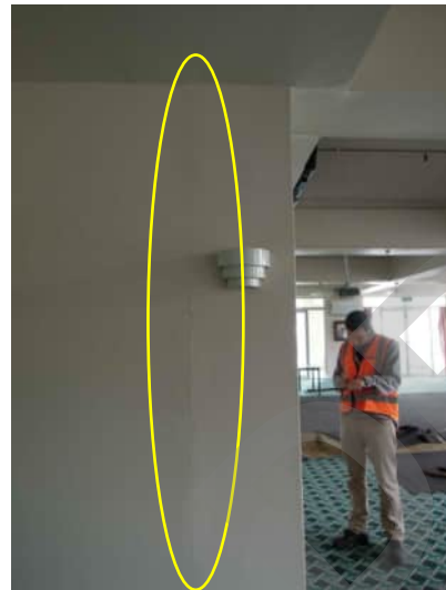
0.41 SEPARATION TO GIB LINING BETWEEN GRID 17 COLUMN AND WALL A-500
