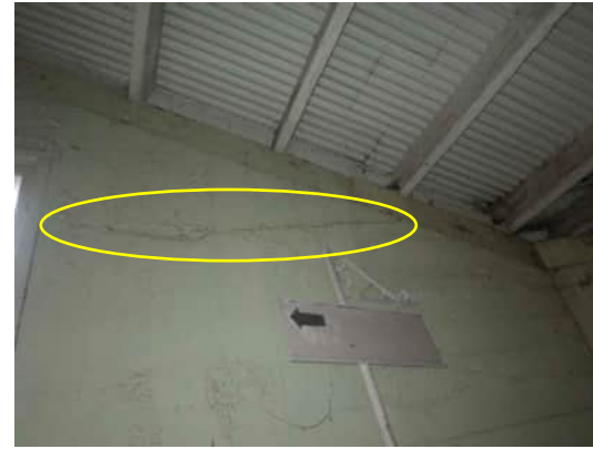
0.15 HORIZONTAL CRACK TO TOP OF WALL AT GRID A A-500
