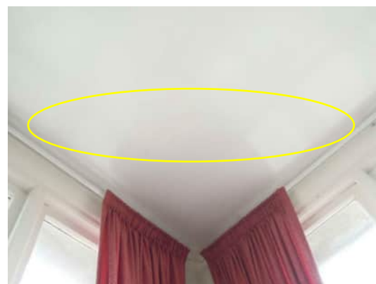
2.46 A-520 | CRACKING TO PLASTER IN CORNER OF SLAB SOFFIT AT GRID 21/D
