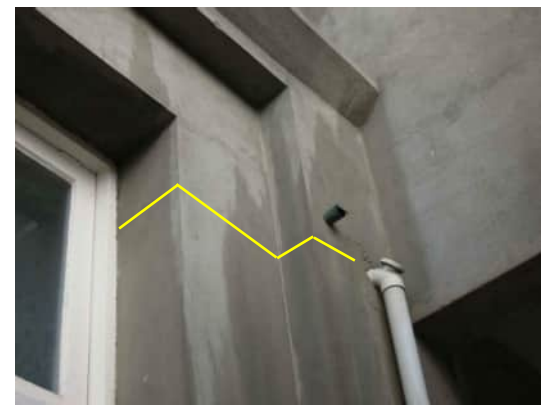
EW13 A-557 | HORIZONTAL CRACK NEAR CEILING LEVEL OF GROUND FLOOR, ON COLUMN BETWEEN GRID B AND GRID C
