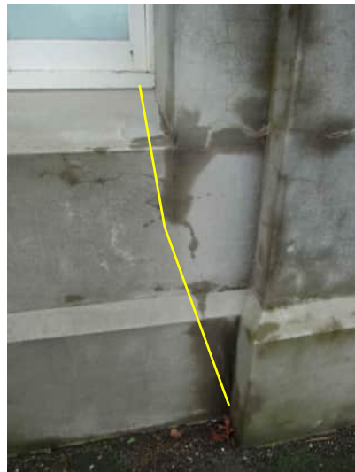
ES9 A-550 | VERTICAL CRACK UP TO 0.3MM FROM CORNER OF WINDOW ON GROUND FLOOR AT GRID 4 COLUMN
