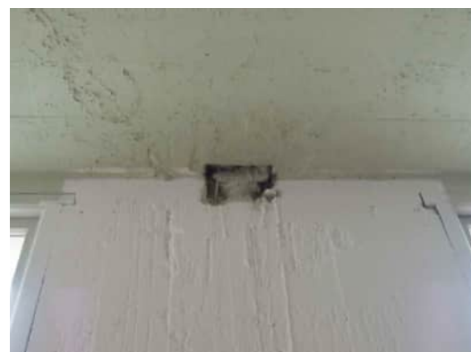
0.11 A-500 | HISTORICAL HOLE IN TOP OF COLUMN BETWEEN GRID C AND D
