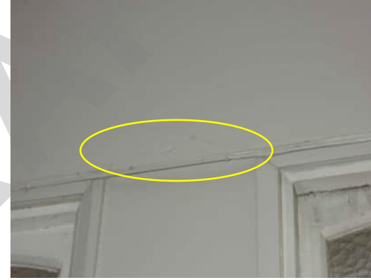
2.19 | CRACK BETWEEN WINDOWS BETWEEN GRID D AND A-520 | GRID E
