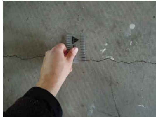
1.5 | CRACK UP TO 1MM PERPENDICULAR TO THE CRACKS BETWEEN GRID C COLUMNS A-510
