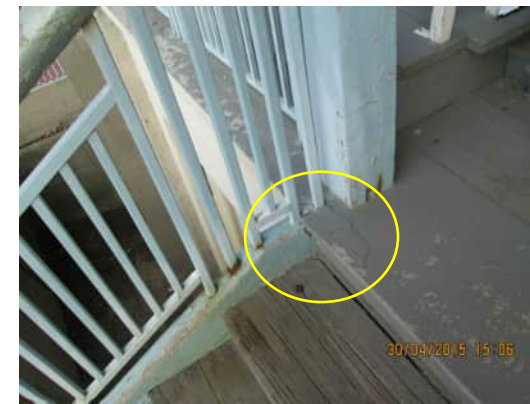
2.52 A-520 | LOWER STAND SLAB EDGE CRACKING
