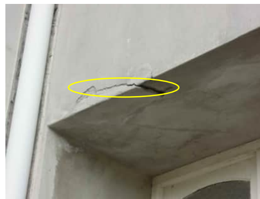
EW23 A-557 | RENDER BREAKING OFF ABOVE SECOND FLOOR WINDOW
