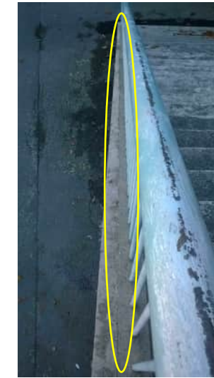
R20 A-810 | CRACK/JOINT ALONGSIDE THE HANDRAIL ON TOP OF STAIR STRINGER
