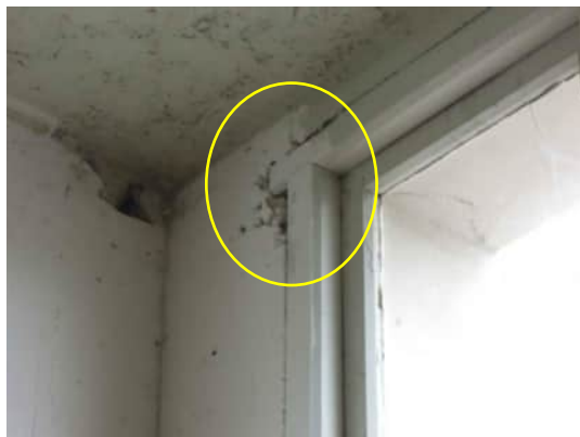
0.9 A-500 | POORLY COMPACTED CONCRETE AROUND WINDOW FRAME AT TOP OF GRID D COLUMN
