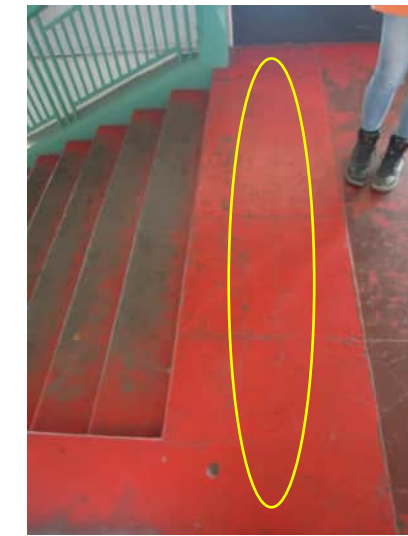
3.8 | CRACK IN COATING ALONG TOP OF STAIRS SPALLING UP TO 10MM WIDE AT SURFACE A-530
