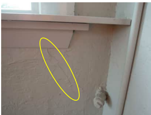
1.11 | 0.3MM DIAGONAL CRACK FROM BOTTOM OF WINDOW IN GRID C COLUMN A-510
