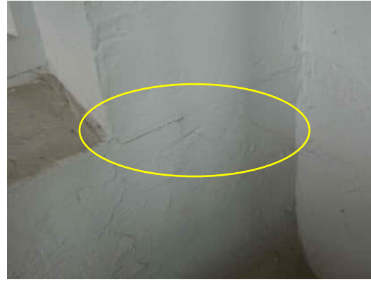
1.14 | CRACK FROM BOTTOM CORNER OF WINDOW IN GRID C COLUMN A-510
