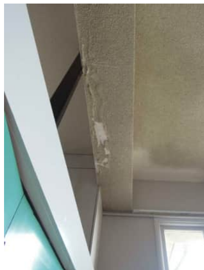
3.45 DAMAGE TO GRID 9 BEAM A-530
