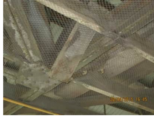
4.14 A-540 | LOOSE TIMBER PIECES CAUGHT IN THE PROTECTIVE MESH
