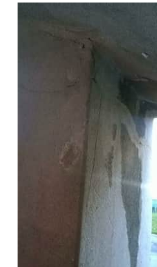
R24 A-810 | MULTIPLE CRACKS AT TOP OF COLUMN
