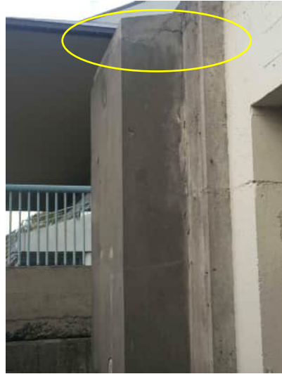
EN11 A-552 HORIZONTAL CRACK AT TOP OF GRID 20 COLUMN
