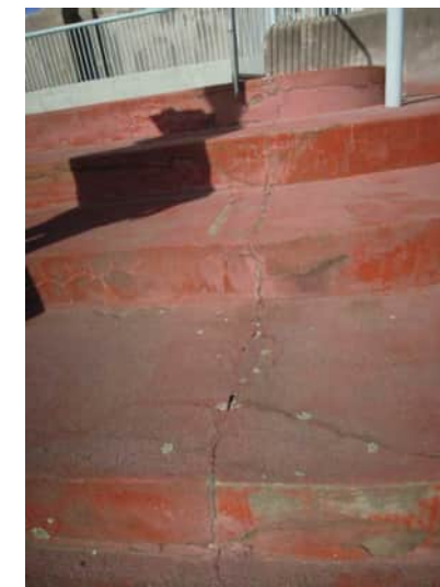
EXT.3 | CRACKS THROUGH STEPS, OCCURS THROUGHOUT A.710
