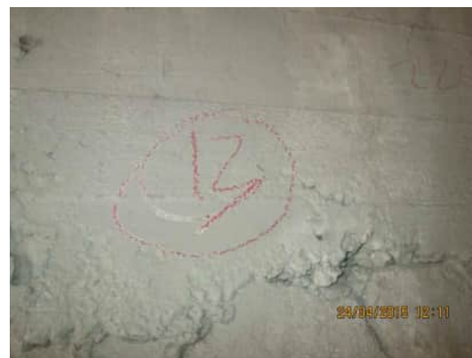
RW.11 SEVERE CONCRETE SPALLING A.710
