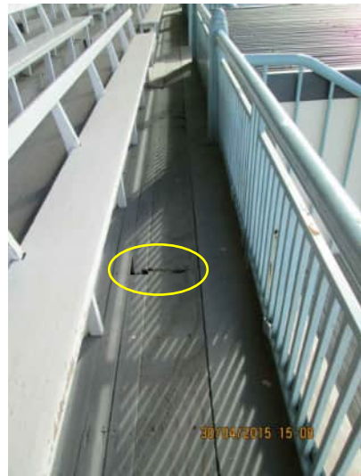
2.53 A-520 | LOWER STAND DAMAGE TO TIMBER DECKING
