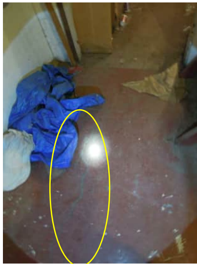
0.5 A-500 | MINOR CRACK TO SURFACE COATING ONLY
