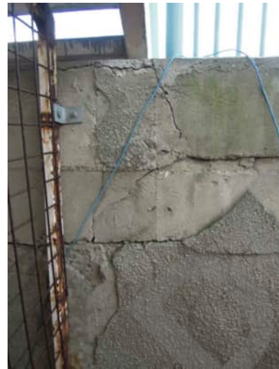
RW.6 SIGNIFICANT CRACKS BELOW STAIRS UP TO 3MM A.710
