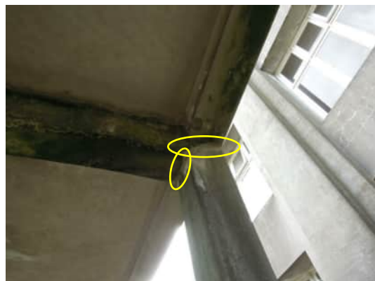
R9 A-810 HORIZONTAL CRACKS AROUND COLUMNS
