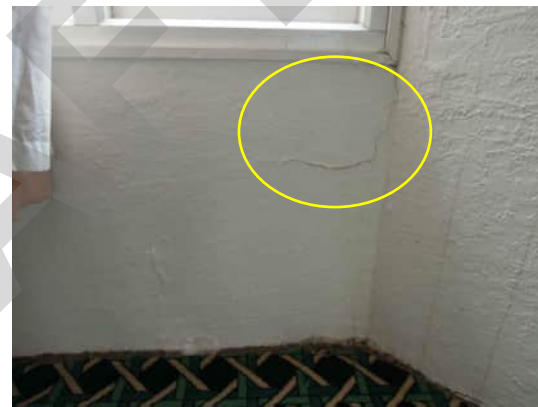
0.30 A-500 | CRACK UP TO 2.5mm BELOW WINDOW ON GRID 20
