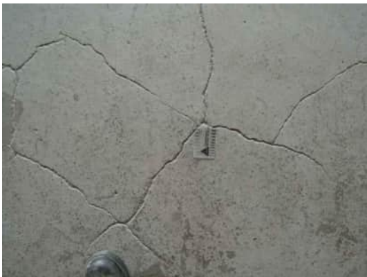
2.5 | CRACKING TO SLAB UP TO 5MM A-520
