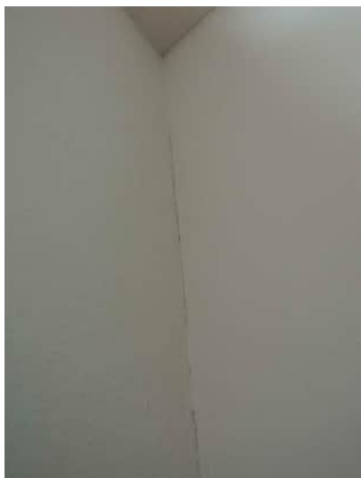
3.33 | SEPARATION BETWEEN COLUMN AND SERVICE SHAFT AT GRID 13 A-530
