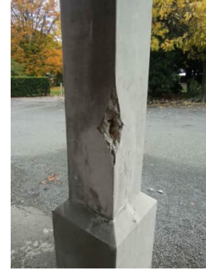
R4 A-810 SPALLING EXPOSING REINFORCING ON THE CORNER OF COLUMN
