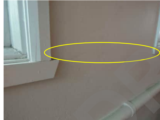
3.42 HORIZONTAL HAIRLINE CRACK ON GRID 12 COLUMN AT BOTTOM OF WINDOW A-530
