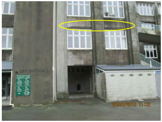
ES1 A-550 HORIZONTAL CRACK ABOVE FIRST FLOOR WINDOWS
