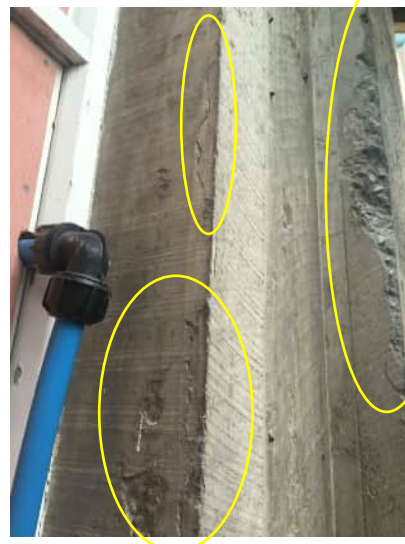
EN10 A-552 VERTICAL CRACK UP TO 0.4MM ON SIDE OF COLUMN AT GRID 11
