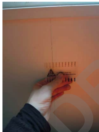
0.53 | TYPICAL SEPARATION BETWEEN PLASTER BOARD PANELS, OCCURS FROM GRID 13 TO GRID 20 A-500
