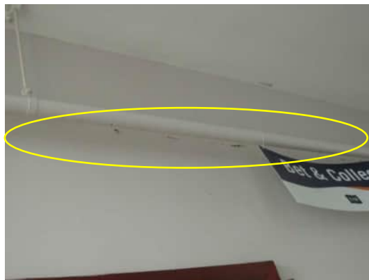
2.12 | SEPARATION BETWEEN WALL AND BEAM BETWEEN GRID C AND GRID D A-520
