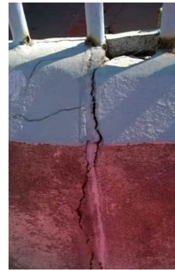
S23 A-818 | SIGNIFICANT CRACK IN LANDING SLAB AT BOTTOM OF STAIRS SHOWN IN PHOTO S22 CONTINUES INTO WALL
