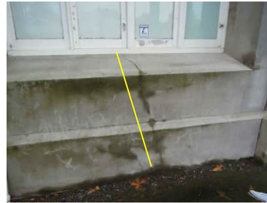
ES7 A-550 | TYPICAL VERTICAL CRACK BELOW WINDOW ON GROUND FLOOR
