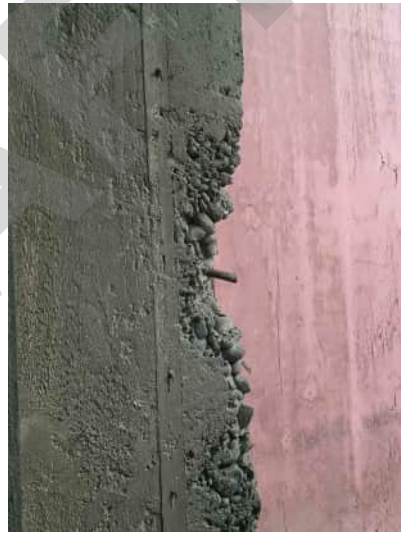
EN7 A-552 CONCRETE SPALLING WITH PROTRUDING STEEL BAR AT CORNER OF GRID 10 COLUMN
