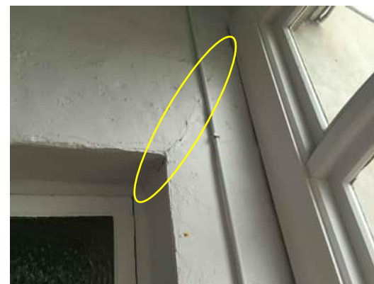
1.23 | DIAGONAL CRACK FROM TOP CORNER OF WINDOW IN WALL BETWEEN GRID B AND C A-510
