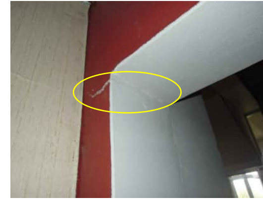
3.28 | HORIZONTAL CRACK AROUND SIDE AND BACK OF GRID 13 COLUMN A-530
