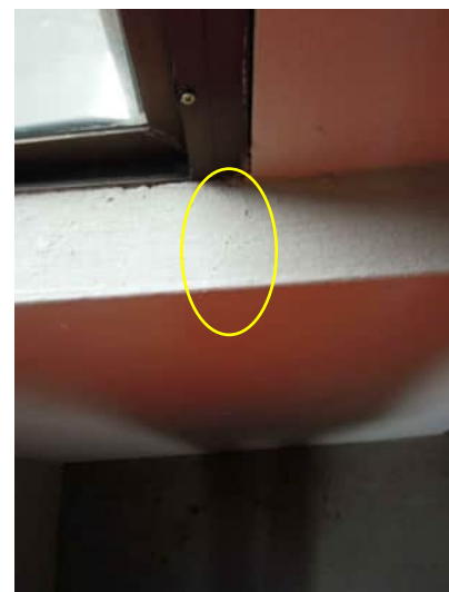
2.34 | HAIRLINE CRACK BELOW WINDOW IN LIFT SHAFT WALL ON GRID 10 A-520
