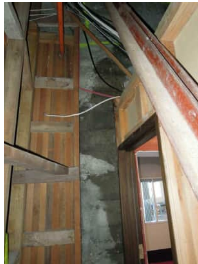
3.53 WATER INGRESS DAMAGE AT GRID 13 THROUGH CRACKING AT TOP A-530
