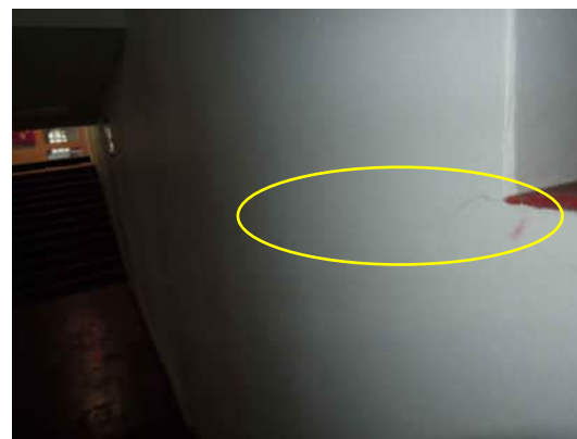
3.26 | HORIZONTAL HAIRLINE CRACK ALONG SHEAR WALL FROM GRID 10 TO GRID 12 A-530
