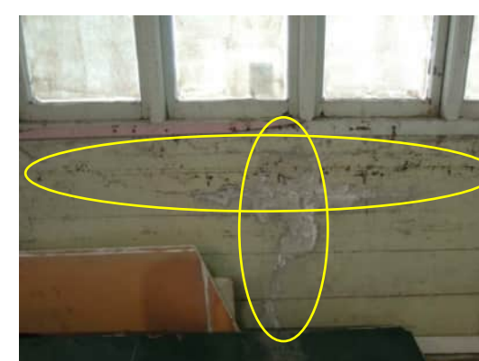
0.46 HORIZONTAL AND VERTICAL CRACK BELOW WINDOW BETWEEN GRID 4 AND 5 A-500
