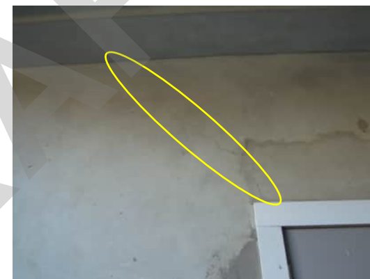
0.66 DIAGONAL CRACK ON EXTERIOR FACE OF CONCRETE WALL A-500
