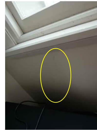
2.20 | HAIRLINE DIAGONAL CRACK BELOW WINDOW NEXT TO A-520 | GRID C COLUMN
