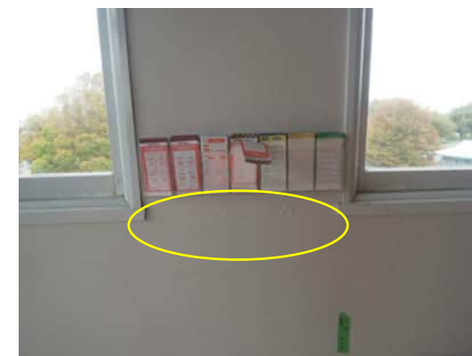
3.36 | EVIDENCE OF MOISTURE ON GRID 20 COLUMN. SIMILAR AT GRID 3 AND 5 A-530
