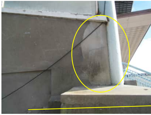
EE13 A-554 | CRACKING TO WALL ABOVE GRID A COLUMN
