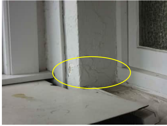
1.13 | CRACK FROM BOTTOM CORNER OF WINDOW IN WALL BETWEEN GRID B AND C A-510
