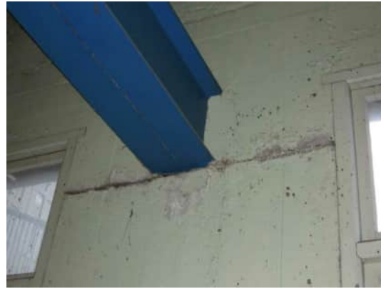
0.14 HORIZONTAL CRACK AT TOP OF WALL AT GRID B IN CONSTRUCTION JOINT, BELOW CAST-IN STEEL BEAM. A-500
