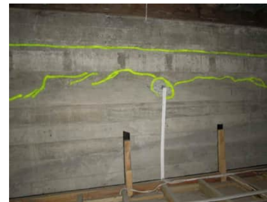
3.48 HORIZONTAL CRACKS TO SHEAR WALL. UPPER CRACK IS THROUGH POUR LINE. LOWER CRACK IS 0.2 TO 0.5MM WIDE A-530
