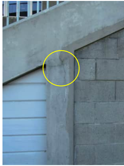
S1 A-814 | CRACKS AT THE TOP OF THE COLUMN UP TO 0.4MM
