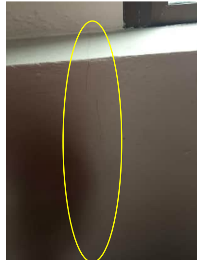
1.28 | VERTICAL CRACK UP TO 0.2mm BELOW WINDOW AT GRID 11 IN LIFT SHAFT EXTENSION A-510
