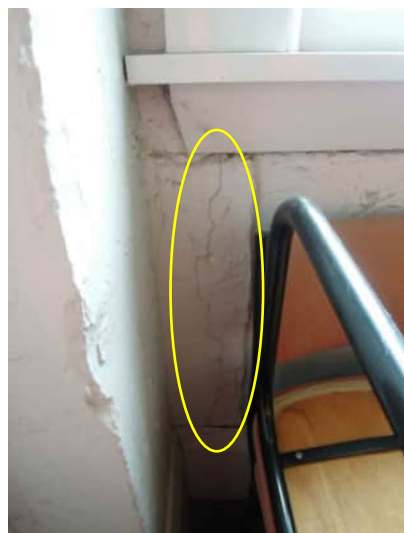
1.9 | 0.9MM VERTICAL CRACK FROM BOTTOM OF WINDOW IN GRID C COLUMN A-510
