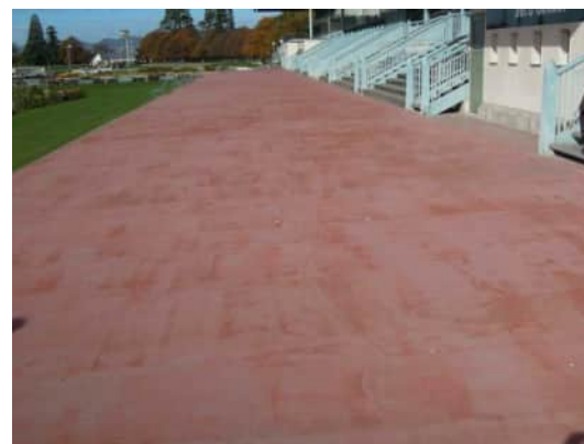
EXT.1 | CRACK ALONG ENTIRE LENGTH OF SLAB A.710
