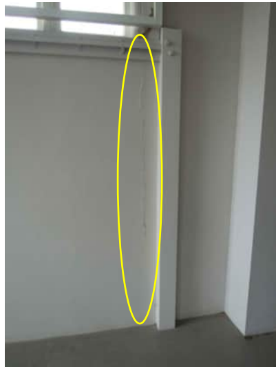
2.13 | VERTICAL CRACK BETWEEN GRID D COLUMN AND WALL A-520 | AVERAGE 2MM, UP TO 3.5MM
