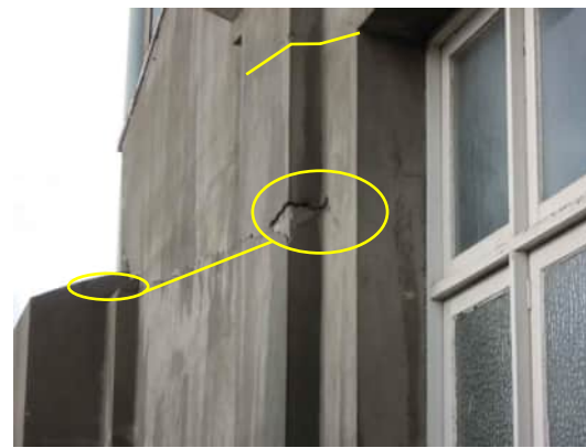
EW15 A-557 | HORIZONTAL CRACK BECOMES WIDER TOWARDS GRID A
