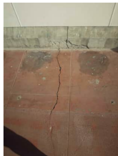
EXT.8 | CRACK IN SLAB AND RETAINING WALL A.710
