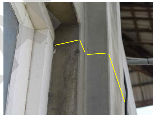
EE19 A-554 | HORIZONTAL CRACK IN COLUMN BETWEEN GRID B AND C
