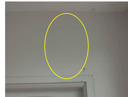
1.20 | CRACK IN WALL NEAR GRID E ABOVE WINDOW FRAME A-510
