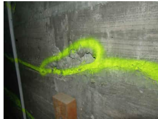
3.51 POOR QUALITY CONCRETE ON GRID 4 WITH 2MM WIDE HORIZONTAL CRACK A-530
