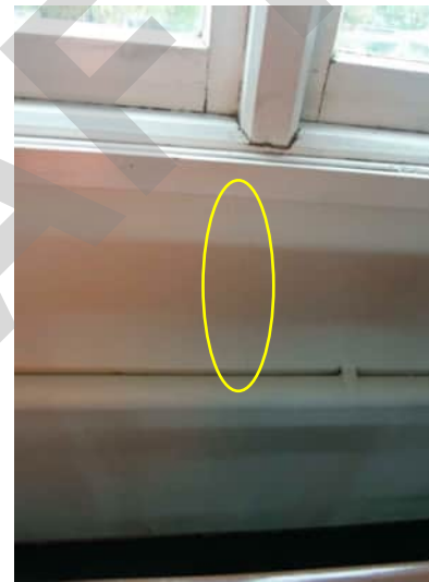
2.31 | 0.1-0.2mm WIDE VERTICAL CRACK BELOW WINDOW BETWEEN GRID 16 AND 17 A-520
