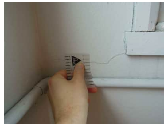
3.38 0.3MM HORIZONTAL CRACK IN GRID 21 COLUMN FROM CORNER OF WINDOW A-530
