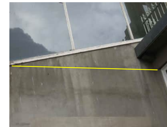
EW12 | HORIZONTAL CRACK IN CONCRETE WALL OF LOWER STAND A-557
