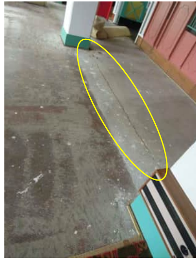
1.2 | LOCATION OF CRACK BETWEEN GRID C COLUMNS A-510
