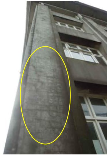
ES5 A-550 | TYPICAL CRAZED CRACKING TO RENDER
