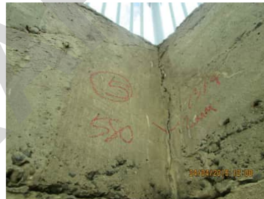
RW.7 CRACK IN CORNER OF RETAINING WALL, 2MM WIDE A.710
