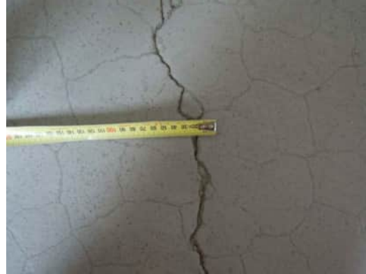
2.3 | CRACK RUNNING DIAGONALLY ACROSS SLAB, UP TO 10MM A-520
