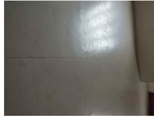
2.4 | CRACK ABOVE BEAM AT CONSTRUCTION JOINT UP TO 2.5MM A-520
