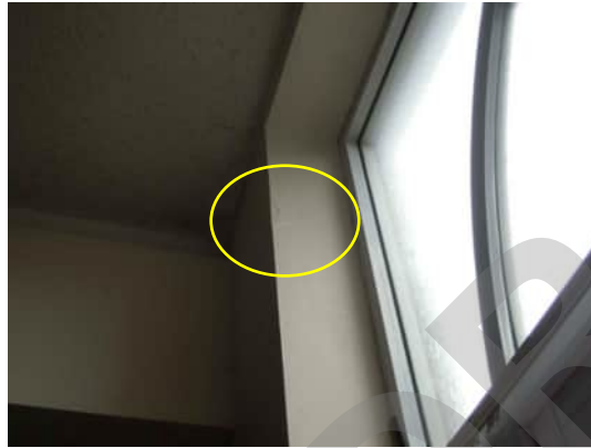
0.18 CRACKS IN DOOR FRAME BETWEEN GRID A AND B A-500
