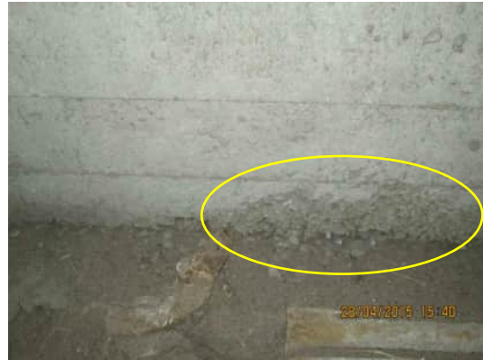
4.5 A-540 | POOR QUALITY CONCRETE OVER HANGING THE FLOOR SLAB
