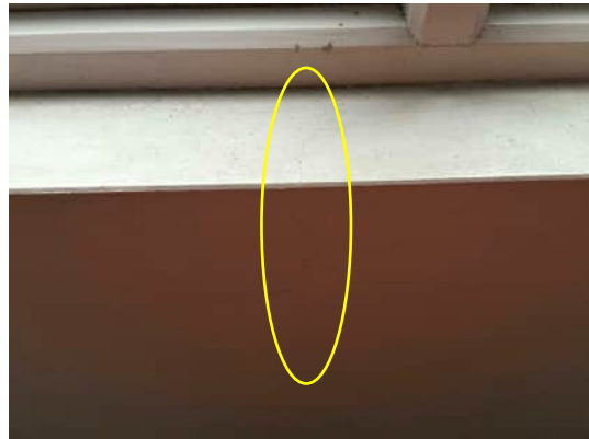
1.29 | HAIRLINE VERTICAL CRACK BELOW WINDOW BETWEEN GRID 12 AND 13 A-510
