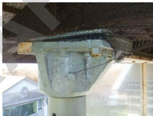
F.7 A.441 | COLUMN COLLAR CONNECTION GRID 20 RUST
