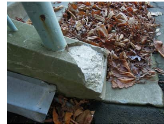
S4 A-814 | DAMAGE TO THE SURFACE OF THE CONCRETE AT BASE OF THE STRINGER
