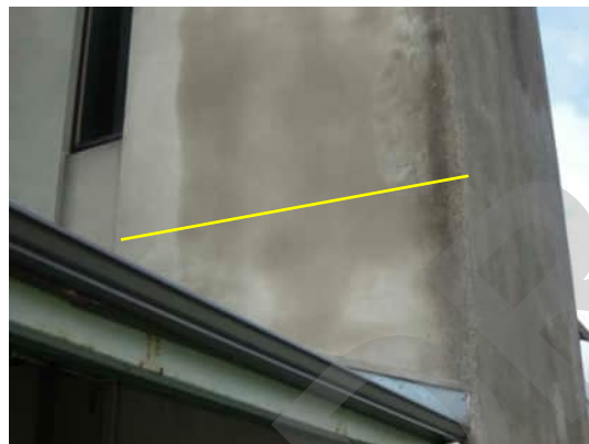
EW18 A-557 | CRACK IN LIFT SHAFT NEAR FLOOR LEVEL OF FIRST FLOOR
