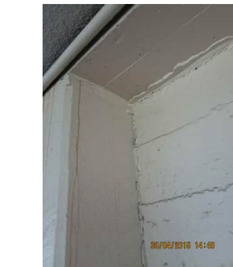
2.48 A-520 | CRACKING TO COLUMN AT GRID 13 AND ADJACENT SHEAR WALL
