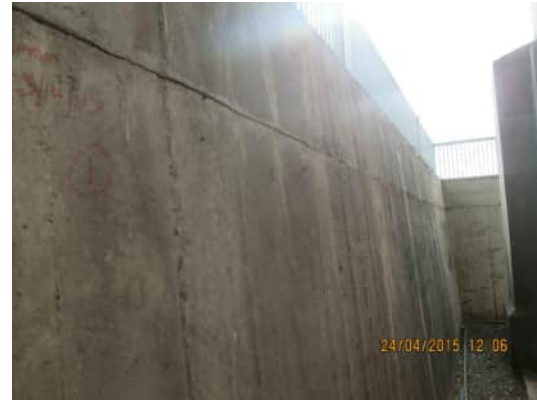
RW.2 VIEW OF RETURN OF RETAINING WALL AT WESTERN END, JOINT IS 0.6MM A.710
