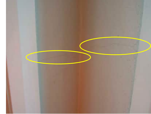
3.20 | HAIRLINE CRACK AROUND 300MM ABOVE BOTTOM WINDOW IN GRID E COLUMN A-530
