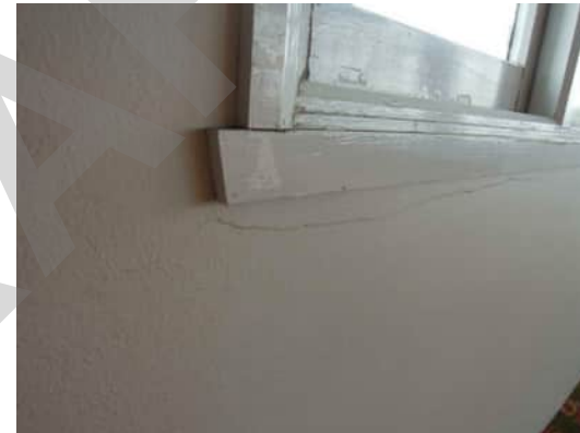
3.31 | HORIZONTAL CRACK IN WALL BELOW WINDOW BETWEEN GRID 2 AND GRID 3 A-530
