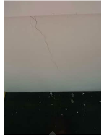
3.15 | VERTICAL CRACK BELOW WINDOW UP TO 0.4MM NEAR GRID C A-530
