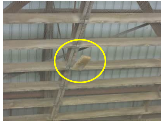
F.2 A.441 | TIMBER BLOCKING SUPPORTING BRACE FALLEN ONTO NET
