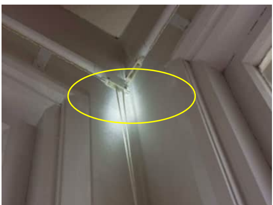
3.21 | HAIRLINE CRACK NEAR TOP OF WINDOW IN GRID E COLUMN A-530
