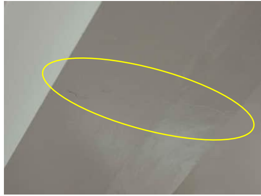
2.37 A-520 | TYPICAL CRACK IN PLASTER FINISH TO BEAM
