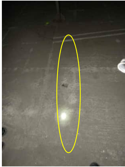
4.1 A-500 | TYPICAL CRACK NEAR GRIDLINE BETWEEN STEEL COLUMNS
