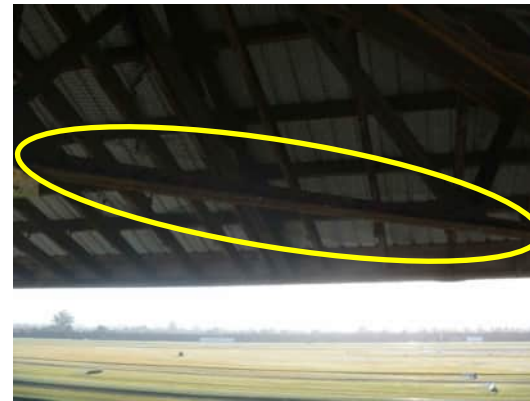
F.8 A.441 | SIGNIFICANT RUSTING TO GRID 20 TO 21 CORNER TRUSS
