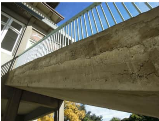
S19 | CRACKS ALONG STRINGER AS WELL AS POORLY COMPACTED CONCRETE A-816
