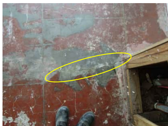
3.9 | CRACK UP TO 5MM WHICH HAS PREVIOUSLY BEEN PARTIALLY REPAIRED A-530
