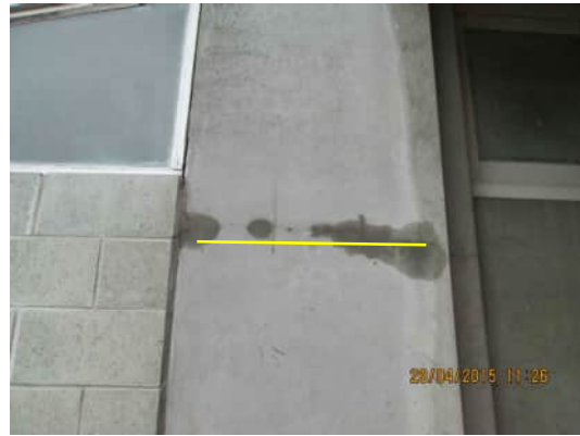
EE2 A-554 HAIRLINE CRACK TO GRID E COLUMN AT GROUND LEVEL
