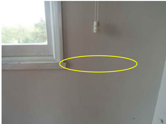
3.17 | HORIZONTAL HAIRLINE CRACK IN GRID D COLUMN AT BOTTOM OF WINDOW A-530
