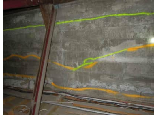
3.50 UPPER CRACK IS THROUGH POUR LINE. POOR QUALITY CONCRETE AT BOTTOM. MIDDLE HORIZONTAL CRACK 0.8 TO 1.6mm WIDE A-530
