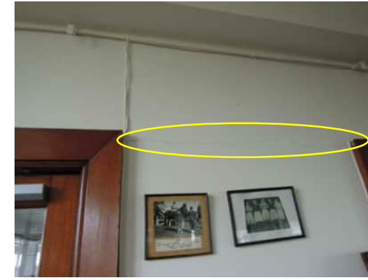
2.16 | CRACK IN WALL BETWEEN GRID C AND GRID D, A-520 | BETWEEN DOOR FRAMES
