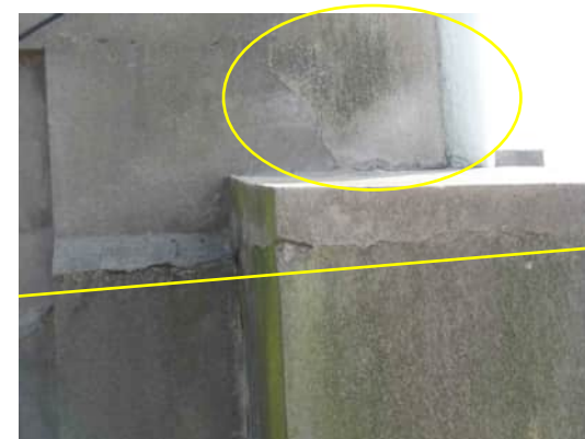
EE12 A-554 CONTINUATION OF CRACK SHOWN IN EE11 THROUGH GRID A COLUMN
