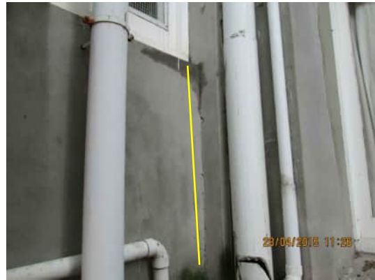
EE1 A-554 TYPICAL CRACK BETWEEN GRID D COLUMN AND CONCRETE INFILL WALL
