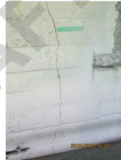
4.7 A-540 | VERTICAL CRACK ON THE EXTERNAL FACE OF THE SHEAR WALL AT GRID 6, RUNNING PARALLEL TO THE STEEL COLUMN ON INTERNAL FACE
