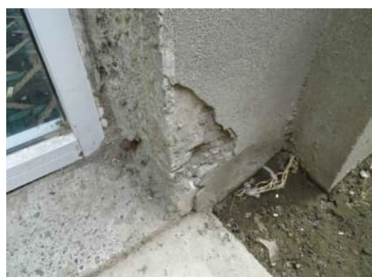
EE9 A-554 DAMAGED CONCRETE ON OTHER SIDE OF DOOR, REINFORCING IS ALSO EXPOSED (WALL APPEARS TO HAVE BEEN CUT TO FORM DOOR)
