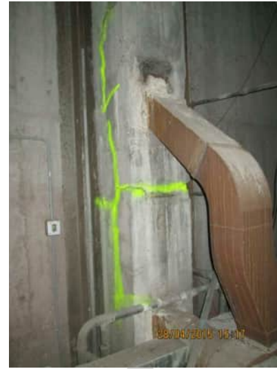
4.3 A-540 | CONCRETE COLUMN HAS SEPARATED FROM THE SHEAR WALL. THE COLUMN HAS MULTIPLE HORIZONTAL CRACKS SHOWING IT HAS BEEN BENT IN FLEXURE
