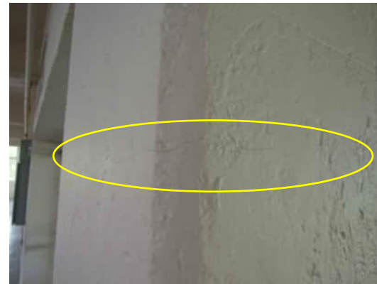
2.22 | HAIRLINE CRACK CONTINUES AROUND GRID 6 COLUMN A-520 | (GRID 3, 14 AND 15 COLUMNS SIMILAR)
