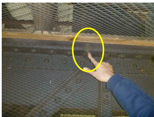
F.9 A.441 | BRACE CONNECTION TO TRUSS, LOOSE BOLT
