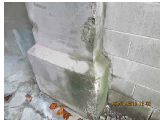
ES4 A-550 DAMAGE TO RENDER AT BASE OF GRID 12 COLUMN
