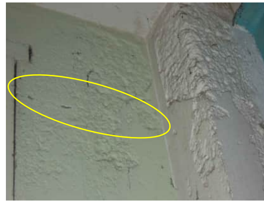
0.25 A-500 | HAIRLINE HORIZONTAL CRACK NEAR TOP OF WINDOW AT GRID 3
