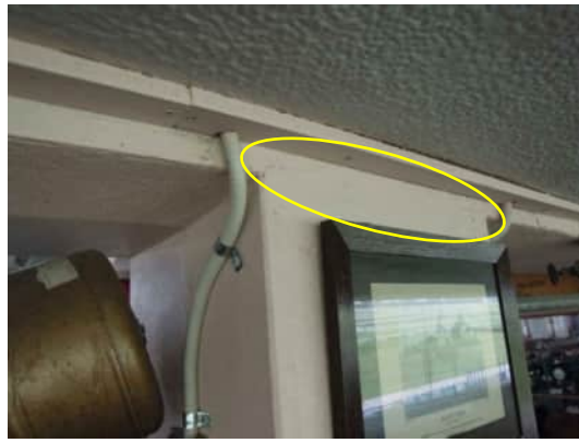
2.25 | CRACK IN BEAM COLUMN JOINT AT GRID 16 A-520
