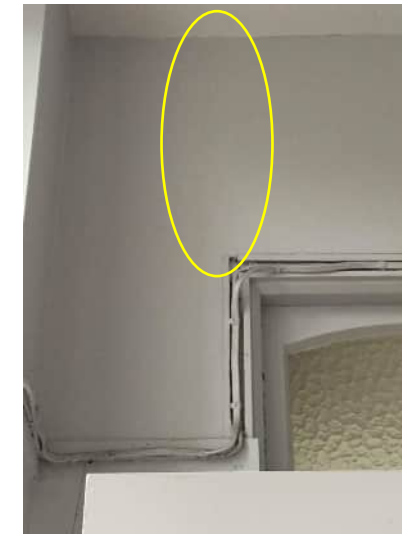
1.16 | CRACK IN GRID E COLUMN ABOVE WINDOW FRAME A-510
