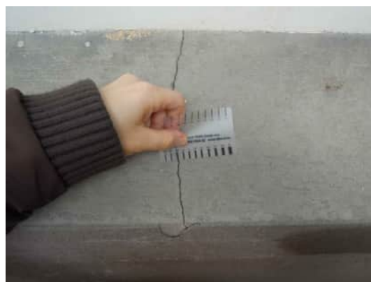
EW10 | 1.0MM VERTICAL CRACK BELOW WINDOW A-557
