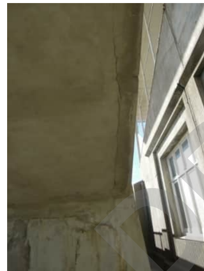
S16 | CRACK ON UNDERSIDE OF STAIRS UP TO 4MM WIDE A-816
