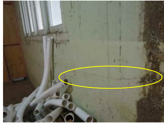
0.13 HORIZONTAL CRACK IN WALL BETWEEN GRID B AND C A-500
