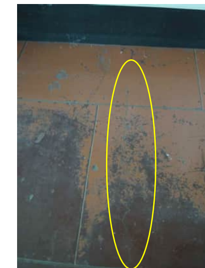
3.12 | CRACK IN COATING UP TO 3MM WIDE A-530
