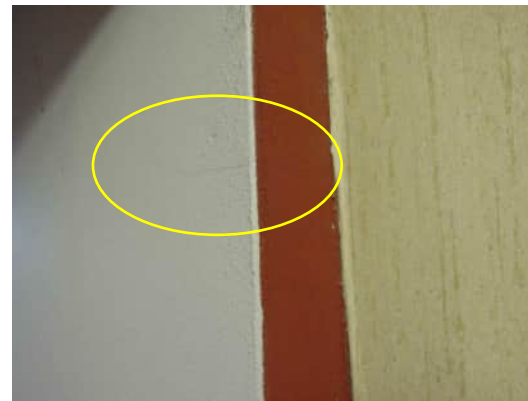
3.23 | HAIRLINE HORIZONTAL CRACK 2M UP THE GRID 9 COLUMN A-530
