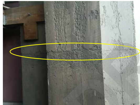
EN6 A-552 MINOR HORIZONTAL CRACK AT LOCATION OF CONSTRUCTION JOINT
