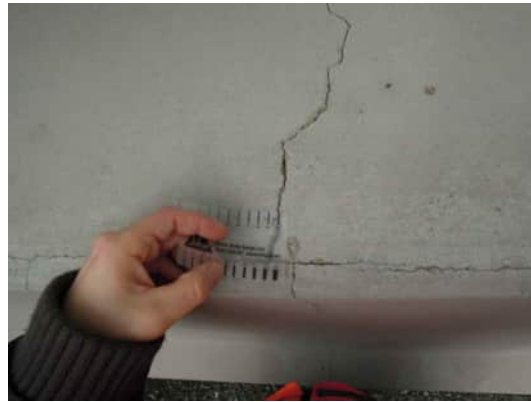
EW2 | 1.0MM VERTICAL CRACK BELOW GROUND FLOOR WINDOW A-557
