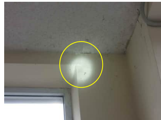
0.20 CRACK ABOVE DOOR FRAME AT GRID D A-500
