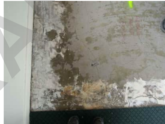
2.7 | PARTIALLY FILLED CRACKS ON SLAB, UP TO 0.8MM A-520
