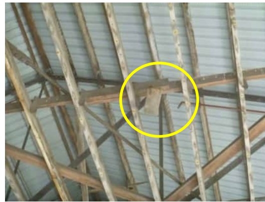
F.3 A.441 | TIMBER BLOCKING SUPPORTING BRACE FALLEN ONTO NET
