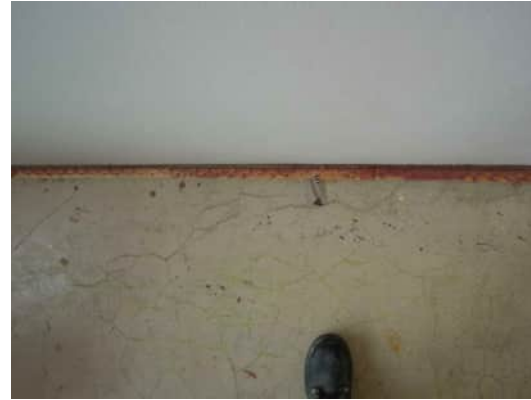
3.2 | CRACK UP TO 0.8MM ALONG GRID 1 A-530
