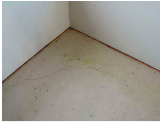
3.1 | DIAGONAL CRACKS AT CORNER OF BUILDING UP TO 3MM A-530
