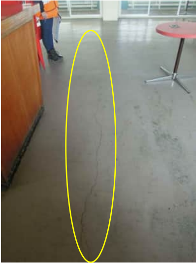
2.1 | TYPICAL CRACK ABOVE BEAM ON GRID 7, UP TO 1.6MM A-520 | TYPICAL FOR GRIDS 2-12
