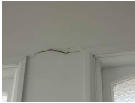
2.14 | SIGNIFICANT HORIZONTAL CRACK WITH SPALLING ON WALL A-520 | BETWEEN WINDOWS BETWEEN GRID D AND GRID E
