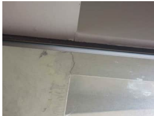
3.41 CRACK ON UNDERSIDE OF BEAMS BETWEEN GRID E BEAM AND BEAM FOR THE LIFT SHAFT EXTENSION, NEAR GRID 11 A-530
