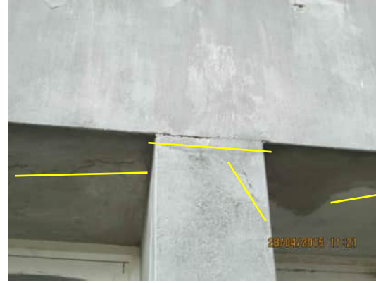
EE3 A-554 HORIZONTAL CRACK AND DIAGONAL CRACKS BETWEEN CENTRAL COLUMN AND THIRD FLOOR WALL
