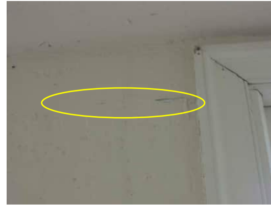
2.8 | CRACK NEAR TOP OF WINDOW ON COLUMN BETWEEN GRID C AND GRID D A-520
