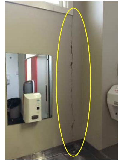
1.15 | CRACK BETWEEN GRID D COLUMN AND WALL 2-3MM WIDE WITH SPALLING UP TO 25MM ON SURFACE A-510
