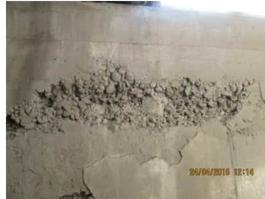
RW.3 TYPICAL AREA WITH POORLY COMPACTED CONCRETE A.710
