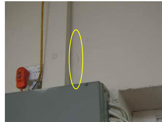
2.23 | VERTICAL CRACK IN BEAM ABOVE GRID 5 COLUMN A-520
