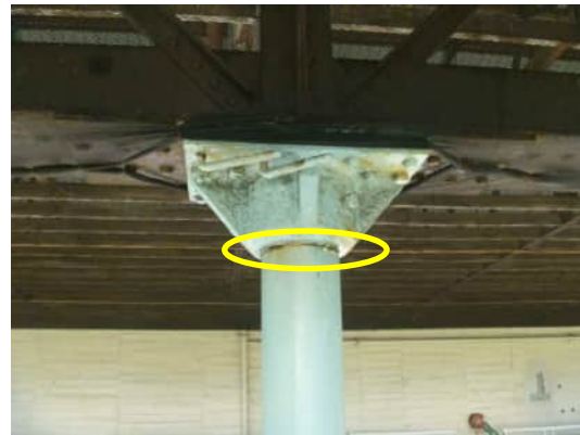
F.5 A.441 | COLUMN COLLAR CONNECTION GRID 8, PAINT SPLIT WITH RUST
