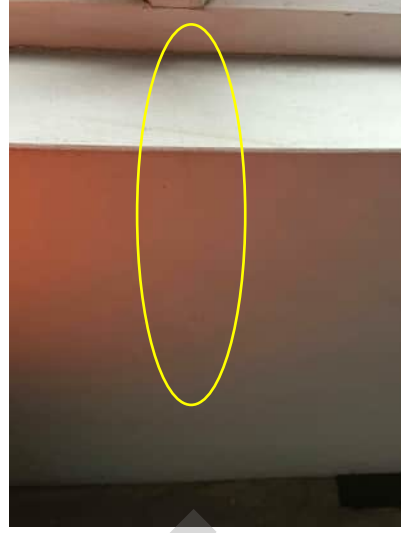
1.27 | HAIRLINE VERTICAL CRACK BELOW WINDOW BETWEEN GRID 9 AND 10 A-510
