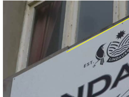
EE15 A-554 | RENDER HAS BROKEN OFF BEHIND SIGN
