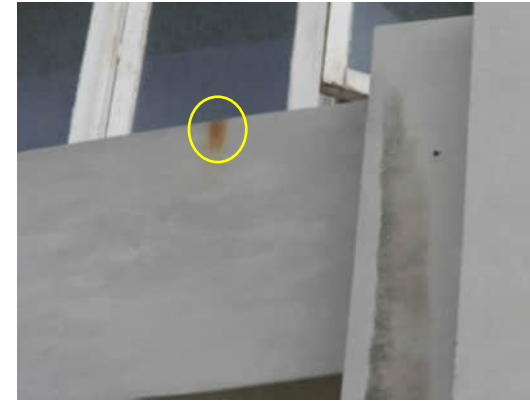
EE16 A-554 | EVIDENCE OF RUST BELOW THE THIRD FLOOR WINDOW
