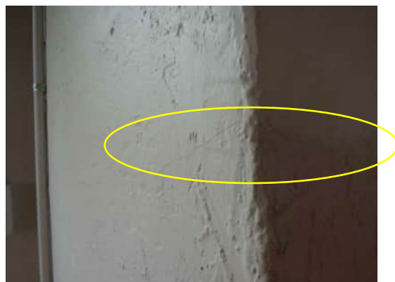
1.10 | HAIRLINE HORIZONTAL CRACK AROUND COLUMN AT MID HEIGHT A-510
