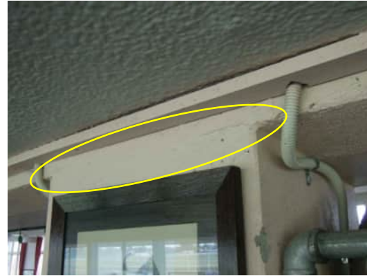
2.26 | CRACK IN BEAM COLUMN JOINT AT GRID 16 A-520
