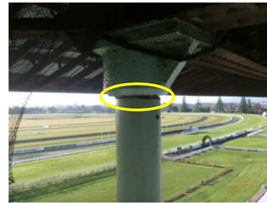
F.4 A.441 | COLUMN COLLAR CONNECTION GRID 2, PAINT SPLIT WITH RUST
