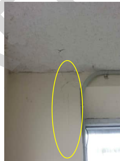
0.54 | CRACKS AT TOP OF GRID 21 COLUMN A-500
