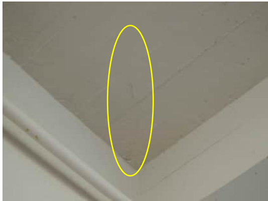
2.41 A-520 | CRACK FROM CORNER OF SLAB SOFFIT AT GRID 7/C
