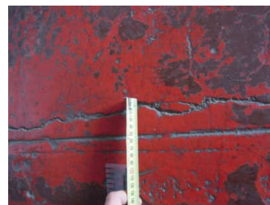
3.11 | CRACK IN COATING SPALLING UP TO 10MM WIDE AT SURFACE A-530
