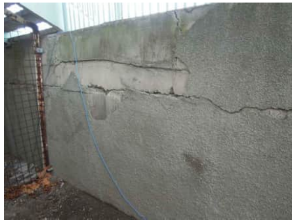
RW.5 SIGNIFICANT CRACKS UP TO 10MM AND DAMAGE TO RENDER A.710
