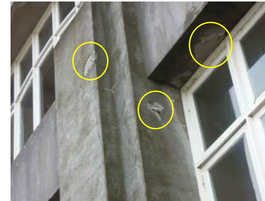
ES12 A-550 | SPALLING ON SIDE OF GRID 3 COLUMN EXPOSING REINFORCING
