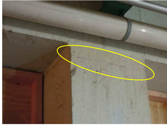
0.36 TYPICAL CRACK NEAR TOP OF COLUMN, ON ALL FACES OF COLUMN A-500
