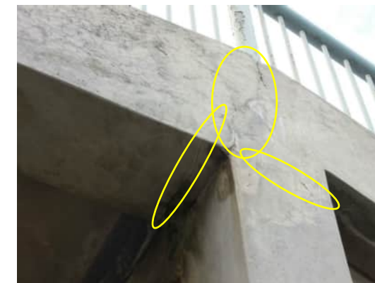
R12 A-810 CRACK THROUGH BEAM COLUMN JOINT WHERE STAIRS CONNECT TO PLATFORM
