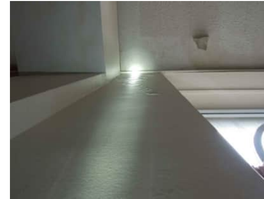
0.51 | SIGN OF MOISTURE DAMAGE TO TOP OF COLUMN ON GRID 17, ALSO OCCURS AT GRID 20 A-500
