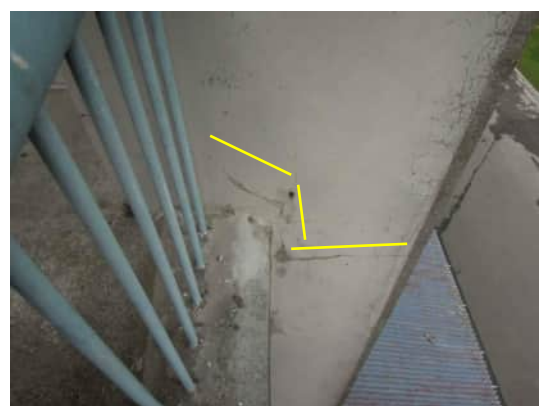
EW21 A-557 | CRACKING TO GRID E COLUMN NEAR WHERE STAIRS CONNECT AT SECOND FLOOR UP TO 0.5MM
