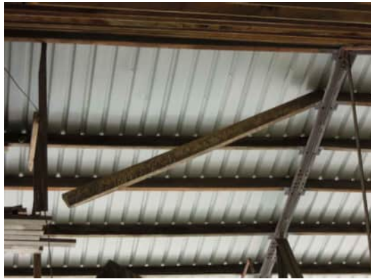
F.1 A.441 | TIMBER PURLIN END CONNECTION FAILED
