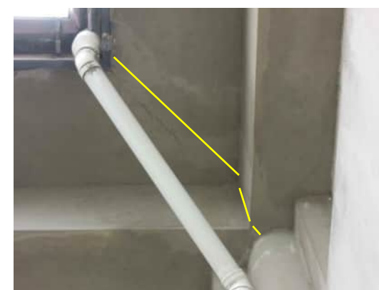
EW24 A-557 | CRACKING TO THE SOFFIT AT GRID D
