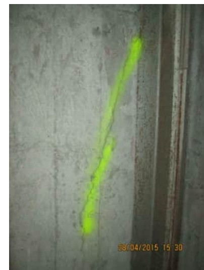
4.4 A-540 | CRACK RUNNING FROM THE STEEL COLUMN VERTICALLY
