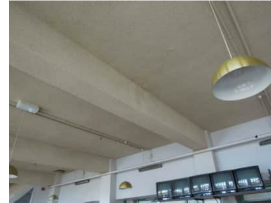
3.44 MOISTURE DAMAGE TO BEAM AND CEILING AT GRID 7 A-530
