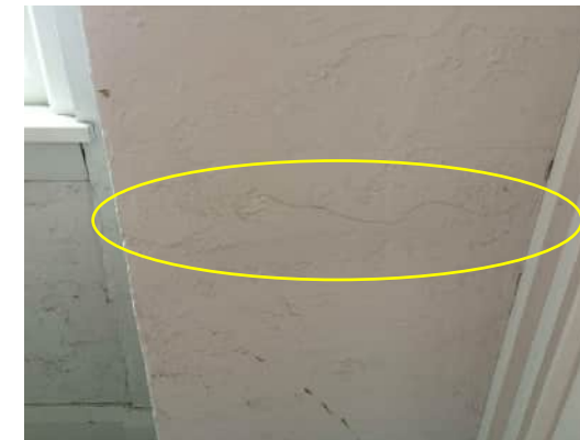
1.24 | HORIZONTAL CRACK AROUND GRID C COLUMN 1m FROM FLOOR A-510
