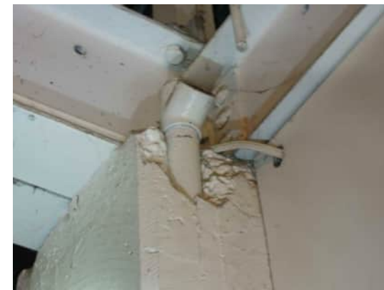
0.31 A-500 | DAMAGE AROUND PIPE CAST INTO COLUMN ON GRID 10
