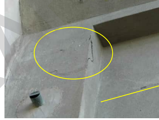
EE7 A-554 CRACKS AND DAMAGE TO RENDER ON THE GRID C COLUMN
