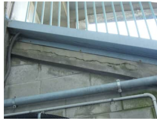
S3 A-814 | CRACK UP TO 5MM ALONG THE OTHER SIDE OF THE STRINGER
