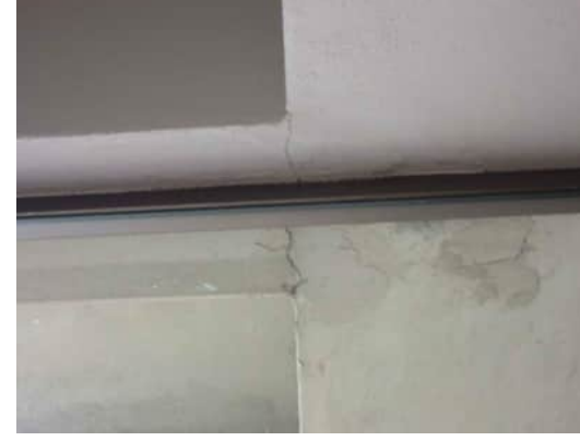
3.40 CRACK ON UNDERSIDE OF BEAMS BETWEEN GRID E BEAM AND BEAM FOR THE LIFT SHAFT EXTENSION, NEAR GRID 10 A-530
