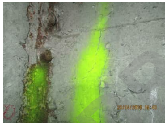
4.6 A-540 | VERTICAL CRACKS NEAR THE CONNECTION BETWEEN SHEAR WALL AND BUTTRESS. POOR CONCRETE AROUND THE CONNECTION
