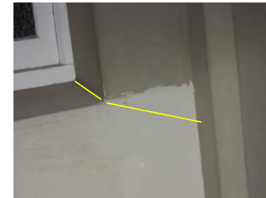
EW8 | DIAGONAL CRACK BELOW WINDOW ON COLUMN BETWEEN GRID B AND GRID C A-557
