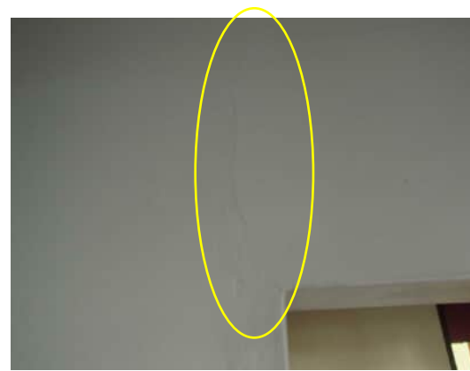
3.27 | VERTICAL CRACK IN SHEAR WALL ABOVE DOOR OPENING NEAR GRID 12 A-530
