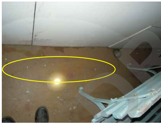
0.6 A-500 | MINOR CRACK TO SURFACE COATING ONLY
