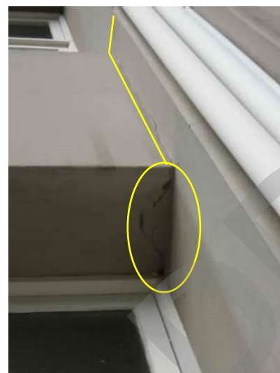
EW6 | TYPICAL SEPARATION BETWEEN WALLS AND COLUMNS A-557
