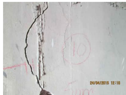
RW.10 1.8M LONG VERTICAL CRACK, UP TO 5MM WIDE, STARTING FROM THE BOTTOM OF THE WALL A.710
