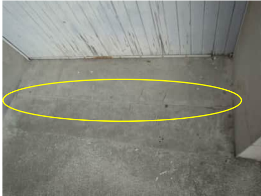
R17 A-810 | CRACK IN SLAB WHERE THE RAMP CONNECTS TO THE BUILDING
