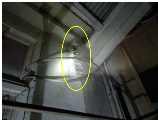
0.28 A-500 | POORLY COMPACTED CONCRETE ON EDGE OF GRID 16 COLUMN
