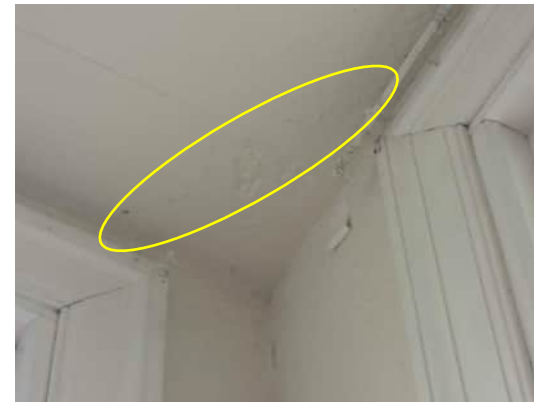
2.39 A-520 | CRACK IN CORNER OF SLAB SOFFIT AT GRID 1/C
