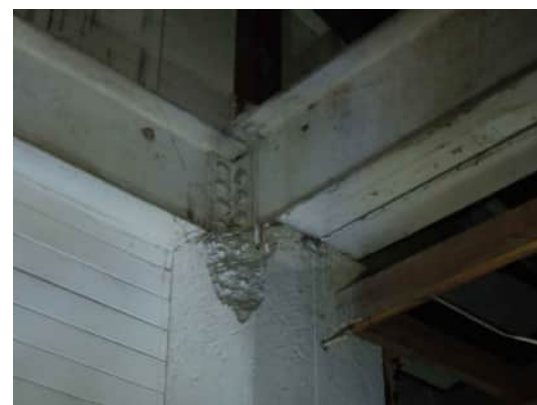
0.32 A-500 | DAMAGE TO TOP OF GRID 12 COLUMN
