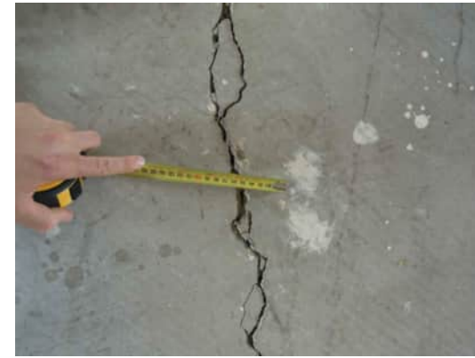
1.4 | SPALLING OF CRACK BETWEEN GRID C COLUMNS A-510
