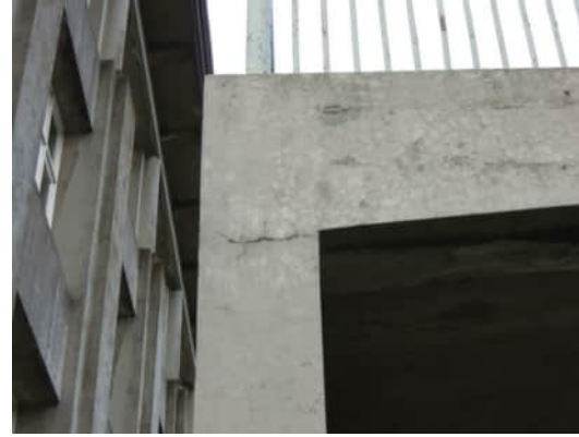
R14 A-810 | HORIZONTAL CRACK AT TOP OF COLUMN
