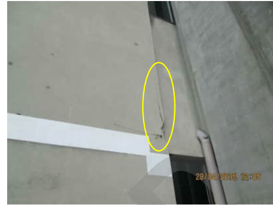
EE6 A-554 DAMAGE TO LIFT SHAFT AT CONNECTION TO MAIN BUILDING
