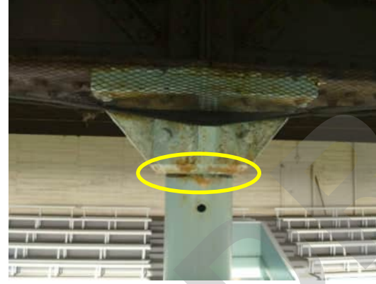
F.6 A.441 | COLUMN COLLAR CONNECTION GRID 14, PAINT SPLIT WITH RUST
