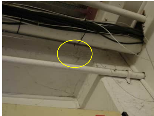
0.37 SIGNIFICANT CRACK TO BEAM NEAR BEAM COLUMN JOINT ON GRID 9 A-500
