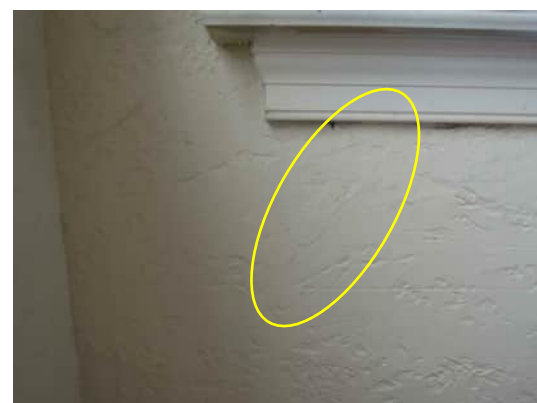
2.10 | 0.1MM DIAGONAL CRACK FROM BOTTOM OF WINDOW AT GRID D A-520
