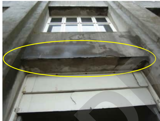
ES10 A-550 | RENDER HAS BROKEN OFF ABOVE DOOR OPENING BETWEEN GRID 5 AND 6
