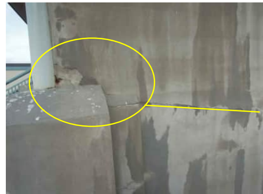
EW17 A-557 | HORIZONTAL CRACK AT GRID A COLUMN WITH SPALLING AND EVIDENCE OF RUST
