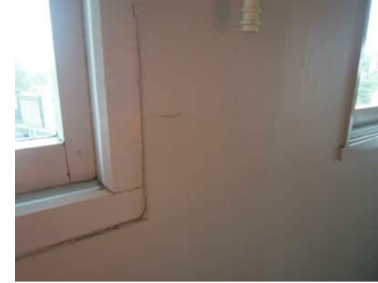
3.32 | SEPARATION OF GIB FROM WINDOW FRAME AND HORIZONTAL CRACK UP TO 0.8MM IN GRID 6 COLUMN A-530
