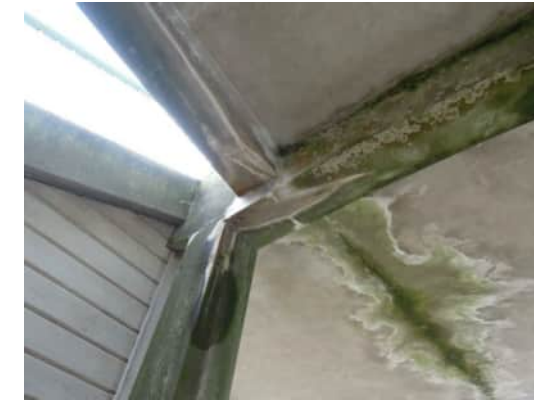
R16 A-810 | MULTIPLE CRACKS TO BEAMS AND COLUMNS WHERE RAMP'S CONNECTS TO LANDING
