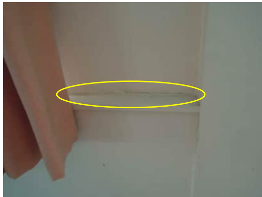
0.52 | HORIZONTAL CRACK IN WALL ON GRID 17 IN LINE WITH BOTTOM OF WINDOW A-500
