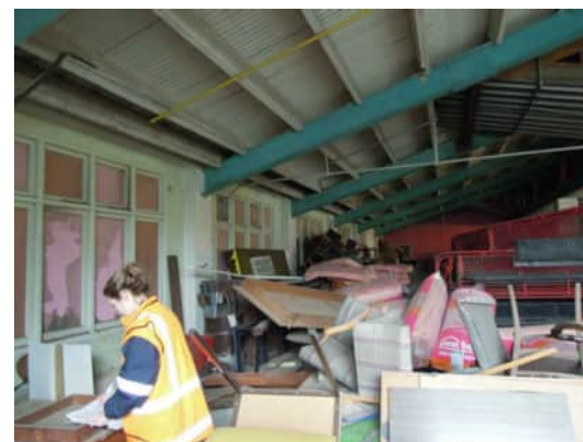
0.22 VIEW OF GRID 3 TO 9, LIMITED ACCESS DUE TO STORED GOODS BLOCKING WALL A-500
