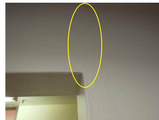
3.24 | DIAGONAL HAIRLINE CRACK IN SHEAR WALL FROM CORNER OF DOORWAY AT GRID 10 A-530
