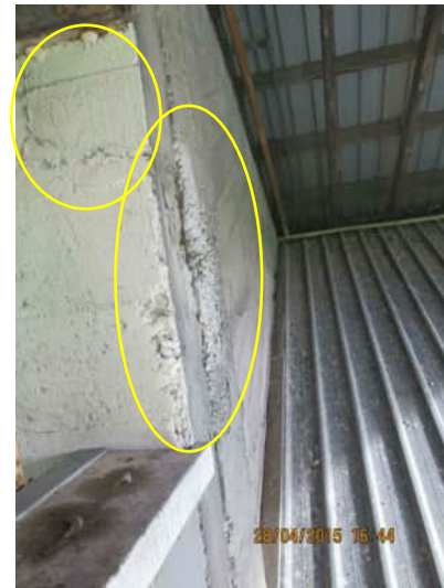
4.11 A-540 | VIEW OF THE WESTERN WING WALL FROM UPPER STAND SHOWING DAMAGE AROUND CONNECTION OF SHEAR WALL TO BUTTRESS WALL
