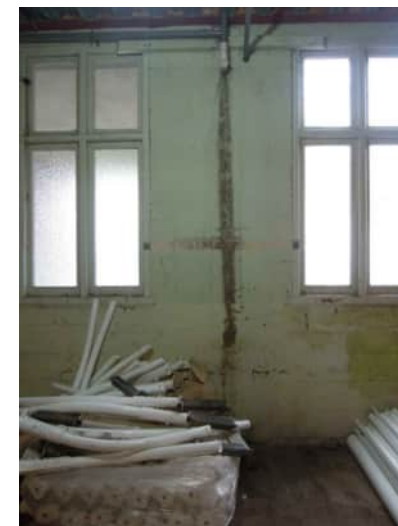
0.12 A-500 | PIPE AT TOP OF COLUMN BETWEEN GRID B AND C, WITH WATER DAMAGE BELOW
