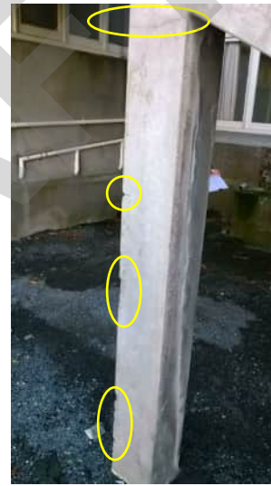
S7 A-814 | HAIRLINE HORIZONTAL CRACK AT TOP OF COLUMN AND SPALLING DAMAGE ALONG HEIGHT
