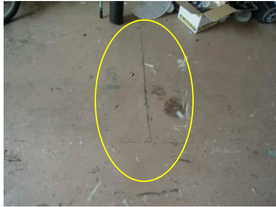
0.1 A-500 | 1.5mm WIDE CRACK
