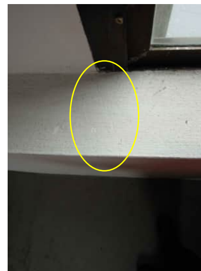
2.35 | HAIRLINE CRACK BELOW WINDOW IN LIFT SHAFT WALL ON GRID 11 A-520
