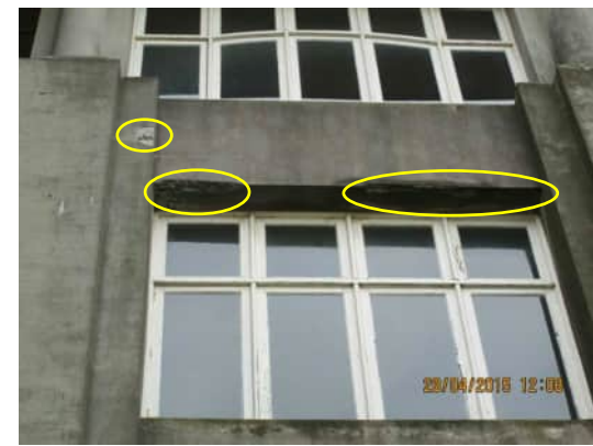
ES3 A-550 DAMAGED RENDER ABOVE SECOND FLOOR WINDOW EXPOSING REINFORCEMENT
