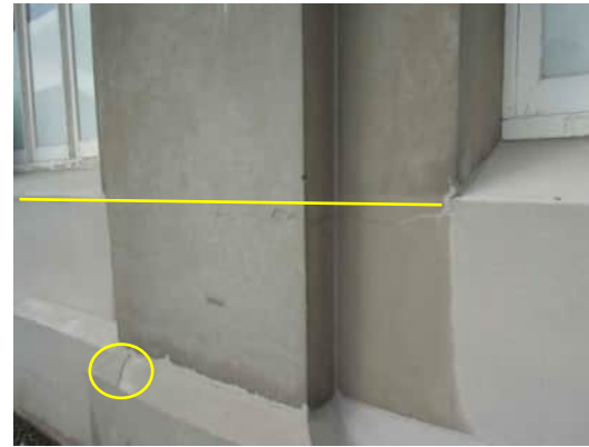
EW3 | 0.2MM HORIZONTAL CRACK NEAR BASE OF CENTRAL COLUMN A-557
