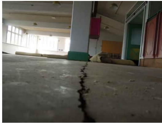
1.3 | CRACK BETWEEN GRID C COLUMNS UP TO 10MM WIDE WITH 5MM VERTICAL DISPLACEMENT A-510
