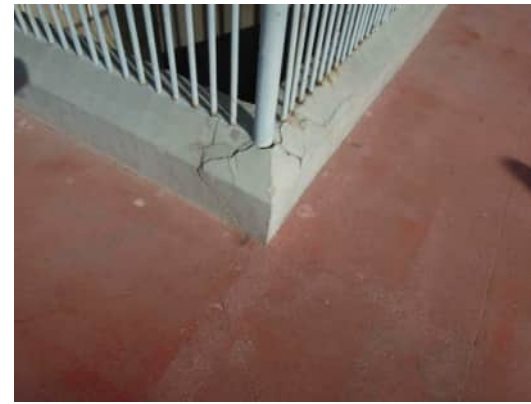
EXT.2 | DAMAGE TO TOP OF RETAINING WALL AROUND CAST-IN HANDRAIL A.710
