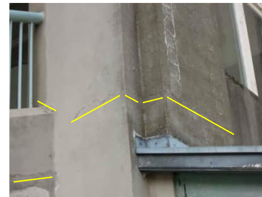
EW20 A-557 | HORIZONTAL CRACK AROUND GRID E COLUMN
