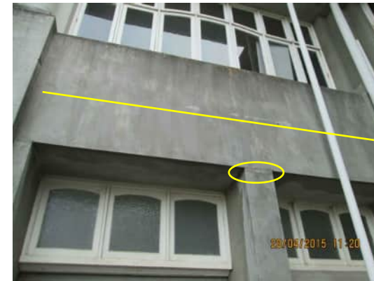
EE4 A-554 HORIZONTAL CRACK ALONG WALL ON THE THIRD FLOOR
