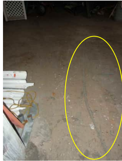
0.2 A-500 | DAMAGE TO FLOOR, 10mm WIDE ON SURFACE ONLY
