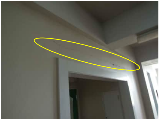
1.17 | HORIZONTAL CRACK ALONG WALL BELOW THE BEAM ABOVE OPENING A-510
