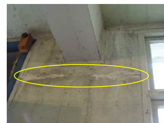
0.47 CRACK IN CONSTRUCTION JOINT ON GRID 5 COLUMN A-500
