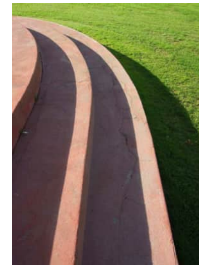
EXT.11 | CRACK ALONG LOWER STEP A.710
