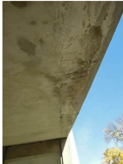
S15 | CRACK ON UNDERSIDE OF STAIRS UP TO 4MM WIDE A-816
