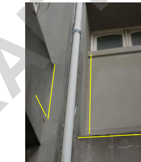
EW19 A-557 | SEPARATION BETWEEN GRID D COLUMN AND INFILL WALL
