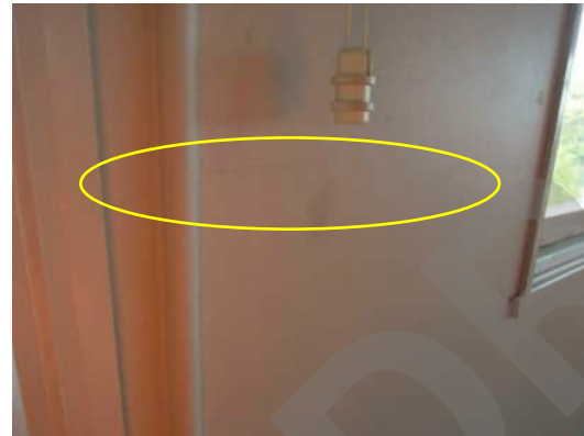
3.30 | HORIZONTAL HAIRLINE CRACK ALONG GRID 4 COLUMN AROUND 300MM ABOVE BOTTOM OF WINDOW (GRIDS 1-9 AND GRIDS 14-19 SIMILAR) A-530
