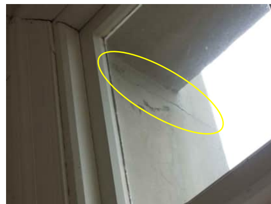
2.9 | CRACK NEAR TOP OF WINDOW ON COLUMN BETWEEN GRID C AND GRID D CONTINUES TO EXTERIOR A-520
