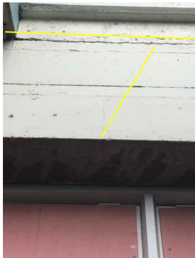
EN9 A-552 SIGNIFICANT HORIZONTAL CRACK AND MINOR VERTICAL CRACK ABOVE WINDOW BETWEEN GRID 10 AND 11, AT LOCATION WHERE STAIRS TO STANDS HAVE BEEN CAST INTO THE WALL
