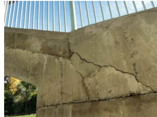
S18 | CRACKS UP TO 15MM AT TOP OF WALL WHERE STAIRS BEGIN A-816
