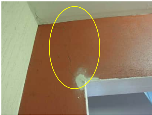
3.25 | 0.8MM DIAGONAL CRACK ON BACK OF SHEAR WALL FROM CORNER OF DOORWAY AT GRID 10 A-530
