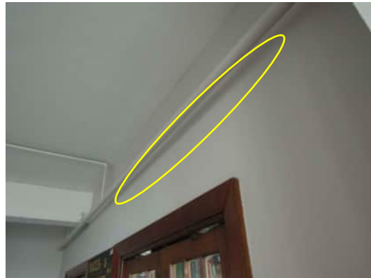
2.17 | SEPARATION BETWEEN WALL AND BEAM BETWEEN A-520 | GRID C AND GRID D
