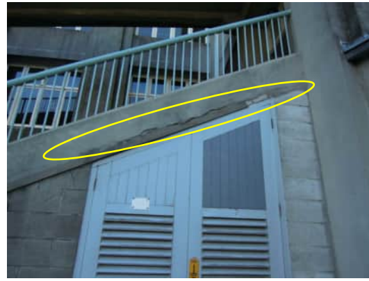
S2 A-814 | CRACK UP TO 20MM ALONG THE SIDE OF THE STRINGER
