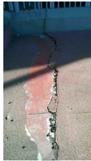
S22 A-818 | SIGNIFICANT CRACK IN LANDING SLAB AT BOTTOM OF STAIRS SHOWN IN PHOTO S20 HAS EVIDENCE OF SETTLEMENT TO THE STAIR SIDE
