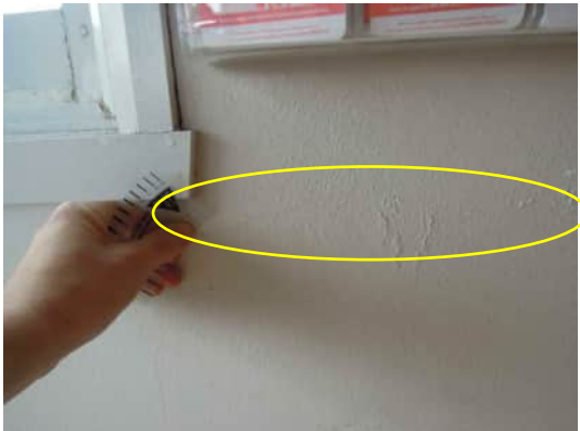
3.29 | HORIZONTAL HAIRLINE CRACK ALONG GRID 20 COLUMN AT BOTTOM OF WINDOW (GRID 1, 2, 3 AND 21 SIMILAR) A-530
