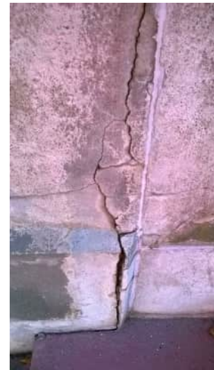
S24 A-818 | SIGNIFICANT CRACK IN WALL WITH SPALLING UP TO 10MM WIDE
