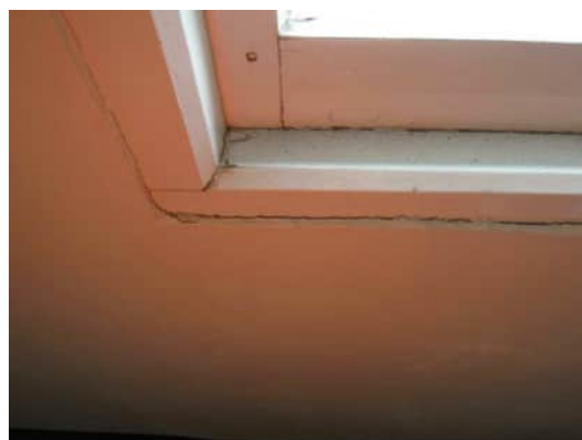
3.34 | SEPARATION OF GIB FROM WINDOW FRAME BETWEEN GRID 15 AND 16. GRID 14 TO 15 SIMILAR. THESE WINDOW FRAMES DIFFER FROM OTHERS ALONG THIS WALL A-530
