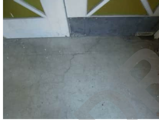
S6 A-814 | CRACK UP TO 1.6MM IN THE SLAB AT THE TOP OF THE STAIRS
