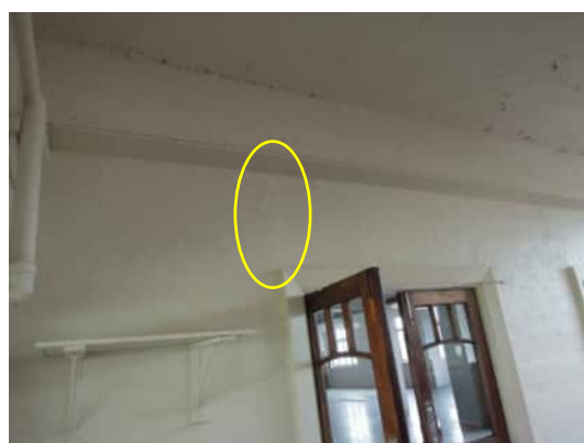
2.11 | CRACKS ABOVE DOOR FRAME IN WALL ALONG GRID 8 BETWEEN GRID C AND GRID D A-520
