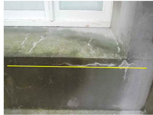
ES6 A-550 | TYPICAL HORIZONTAL CRACK BELOW WINDOW
