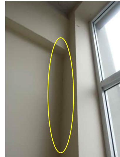
0.43 SEPARATION BETWEEN GRID 21 COLUMN AND WALL A-500
