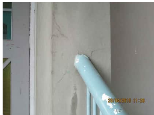
EE5 A-554 CRACKING AROUND CAST-IN HANDRAIL AT THE FIRST FLOOR
