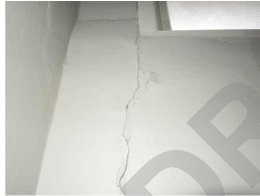
1.18 | 1.6MM VERTICAL CRACK BETWEEN WALL AND COLUMN AT GRID D A-510
