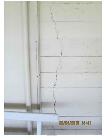
2.51 A-520 | VERTICAL 3.5mm WIDE CRACK TO SHEAR WALL
