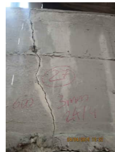
RW.12 APPROXIMATELY 600MM LONG VERTICAL CRACK, STARTING FROM THE TOP OF THE WALL, UP TO 3MM WIDE A.710
