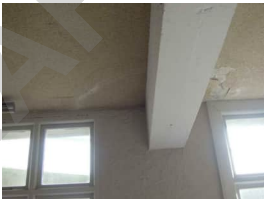
1.31 | TYPICAL MOISTURE DAMAGE TO CEILING AT BEAM COLUMN JOINTS ALONG GRID D A-510
