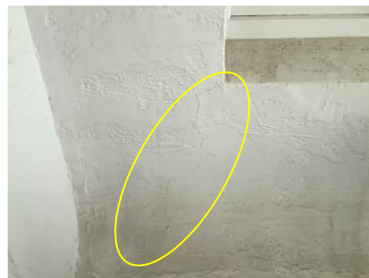
1.22 | DIAGONAL CRACK FROM BOTTOM CORNER OF WINDOW IN GRID C COLUMN A-510
