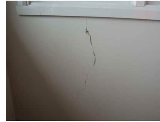
3.16 | 3MM VERTICAL CRACK BELOW WINDOW, CRACK HAS SPALLED UP TO 15MM A-530
