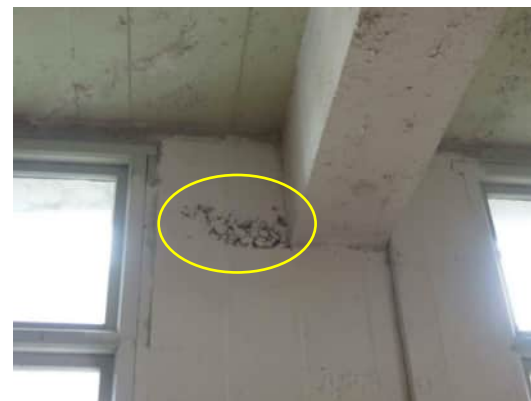
0.45 POORLY COMPACTED CONCRETE AT TOP OF COLUMN, TYPICAL BETWEEN GRID 1 AND GRID 4 A-500
