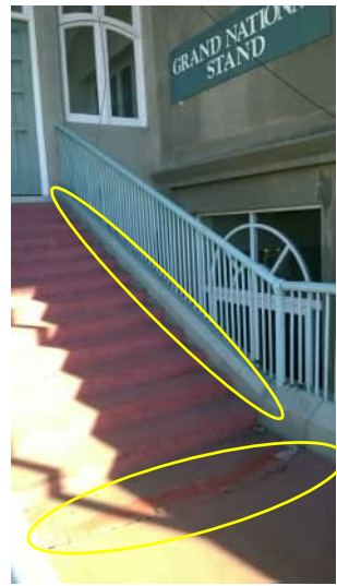
S20 A-818 | SIGNIFICANT CRACK ALONG STRINGER AND ANOTHER SIGNIFICANT CRACK ACROSS LANDING SLAB AT BOTTOM OF STAIRS
