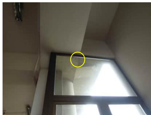
3.39 CRACK ON UNDERSIDE OF BEAMS BETWEEN GRID E BEAM AND BEAM FOR THE LIFT SHAFT EXTENSION, NEAR GRID 11 A-530
