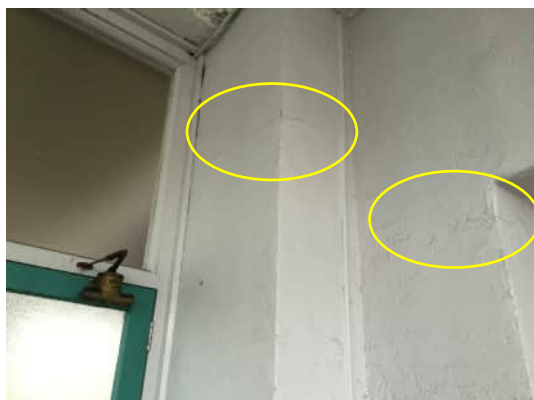
1.21 | HORIZONTAL CRACK IN GRID C COLUMN 0.5m FROM TOP OF COLUMN. CRACK IN WALL NEAR TOP OF WINDOW FRAME A-510
