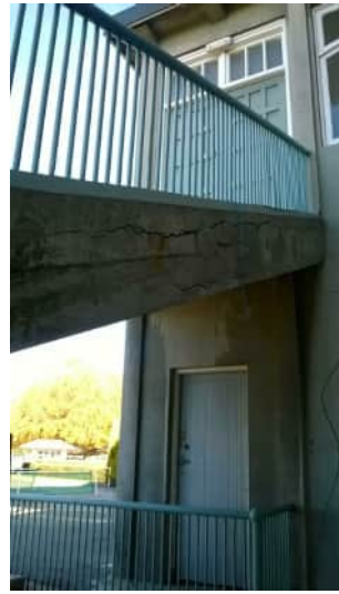
S21 A-818 | SIGNIFICANT CRACK ALONG STRINGER SHOWN IN PHOTO S20 IS ALSO VISIBLE ON OUTSIDE OF STAIRS
