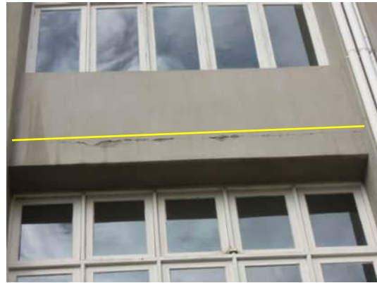
EW1 | SIGNIFICANT CRACK ABOVE FIRST FLOOR WINDOW BETWEEN GRID C AND GRID D A-557
