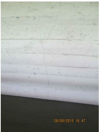
4.9 A-540 | VERTICAL CRACK ON THE EXTERNAL FACE OF THE SHEAR WALL RUNNING PARALLEL TO THE STEEL COLUMN ON INTERNAL FACE
