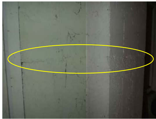
0.24 A-500 | HAIRLINE HORIZONTAL CRACK AT LOCATION OF CONSTRUCTION JOINT ON GRID 3
