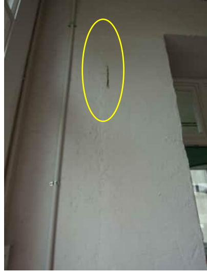
1.26 | DAMAGE TO SURFACE BETWEEN GRID 1 COLUMN AND CONCRETE DOOR FRAME A-510
