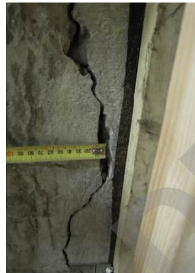
3.54 FULL HEIGHT VERTICAL CRACK UP TO 15MM WIDE A-530
