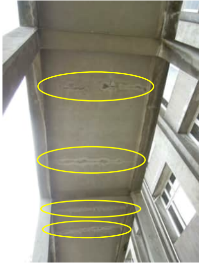
R1 A-810 TYPICAL CRACKS ON UNDERSIDE OF RAMP
