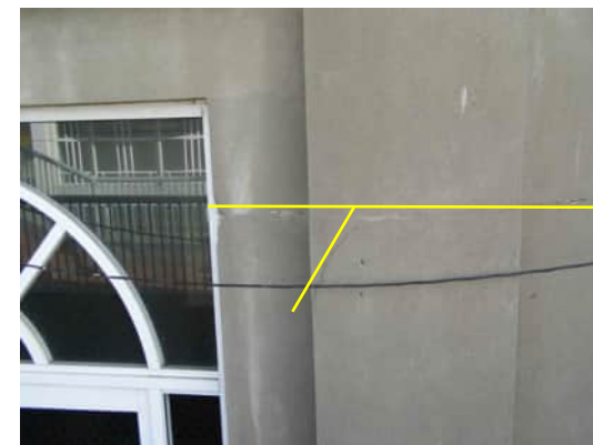
EE10 A-554 SIGNIFICANT HORIZONTAL CRACK ALONG WALL
