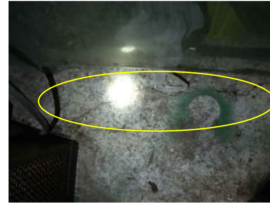
0.4 A-500 | MINOR CRACK IN SLAB
