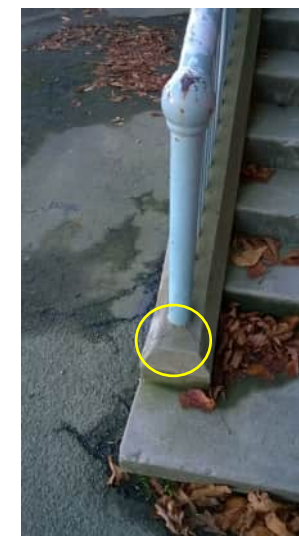
S8 A-814 | CRACKING AROUND WHERE HANDRAIL IS CAST INTO THE CONCRETE
