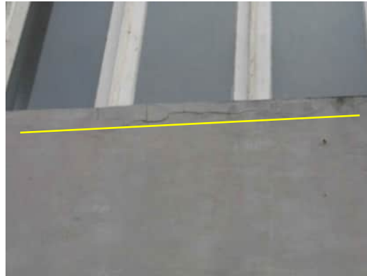
EE14 A-554 | CRACKS BELOW WINDOW BETWEEN GRID C AND GRID D
