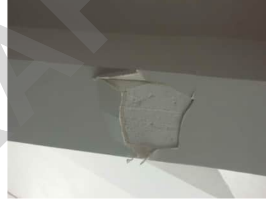
2.43 A-520 | PLASTER BREAKING OFF BEAM UNDERNEATH STAIRS
