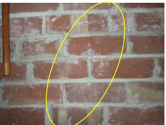
0.68 DIAGONAL STEP CRACKING IN RED BRICK INFILL PANEL A-500
