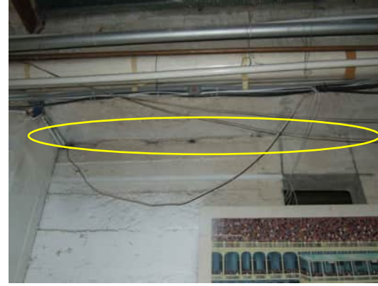
0.38 SEPARATION BETWEEN CONCRETE WALL AND BEAM/COLUMNS BETWEEN GRID 12 AND 13 A-500
