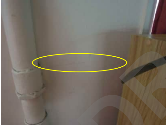
2.30 | HORIZONTAL HAIRLINE CRACK IN COLUMN AT GRID 14 (GRID 8, 17 AND 19 SIMILAR) A-520
