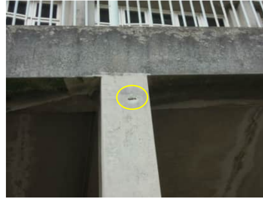
R3 A-810 SPALLING EXPOSING THE REINFORCING
