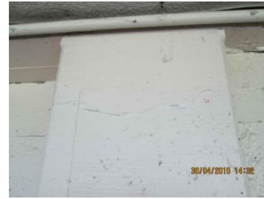
2.47 A-520 | CRACKING TO COLUMN AT GRID 9
