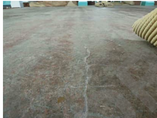
1.6 | TYPICAL CRACK OVER THE CENTRE OF BEAMS RUNNING BETWEEN GRID C AND GRID D A-510
