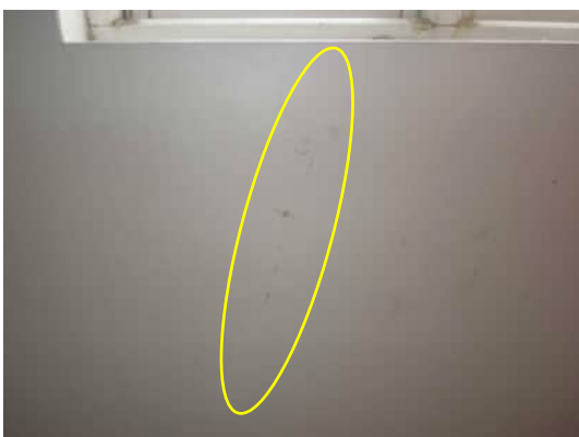
2.33 | HAIRLINE DIAGONAL CRACK BELOW WINDOW BETWEEN GRID 9 AND 10 WITH SOME MOISTURE SEEPAGE A-520
