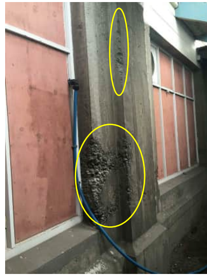
EN2 A-552 AREA OF SEGREGATED CONCRETE ON COLUMN FACE AND SIDES
