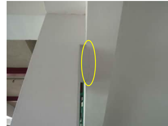
2.44 A-520 | SEPARATION BETWEEN COLUMN AND CEILING AT STAIRS
