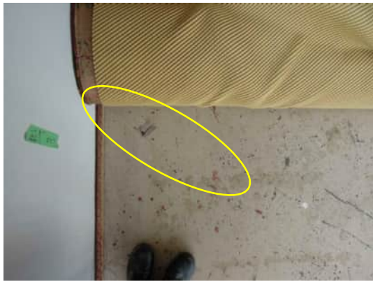
3.13 | CRACK ALONG GRID 20 UP TO 0.9MM WIDE A-530
