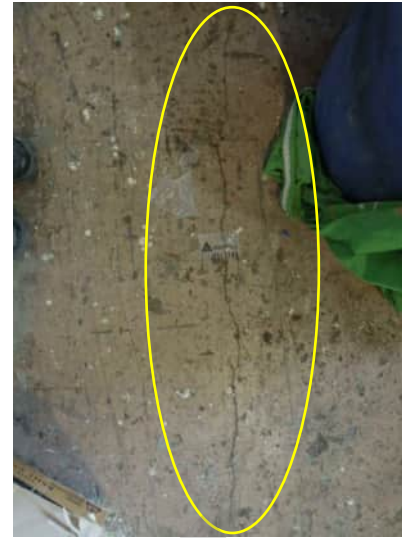
0.3 A-500 | CRACK IN SLAB, UP TO 2mm WIDE
