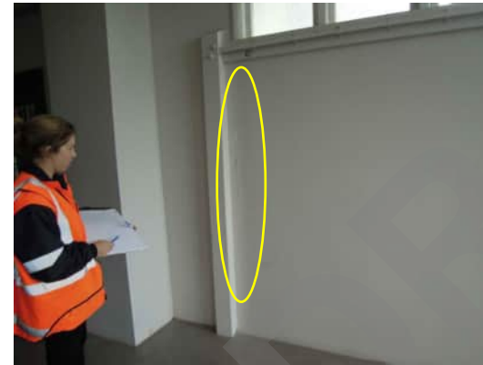
2.18 | 0.7MM VERTICAL CRACK BETWEEN GRID D COLUMN AND A-520 | WALL
