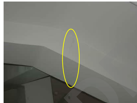
2.42 A-520 | CRACK ON BEAM UNDER STAIRS
