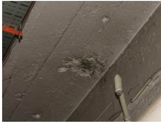
0.60 VOID ON CEILING EXPOSING THE REINFORCING AT GRID 10 A-500
