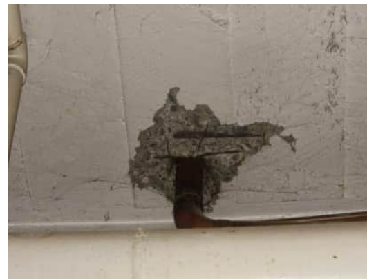
0.61 PIPE THROUGH CEILING WITH SPALLING WHICH HAS EXPOSED REINFORCING A-500
