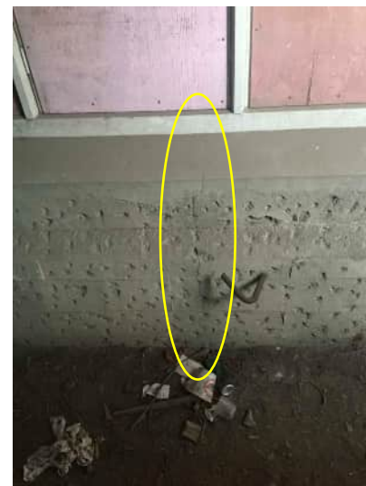
EN4 A-552 VERTICAL CRACK BELOW WINDOW
