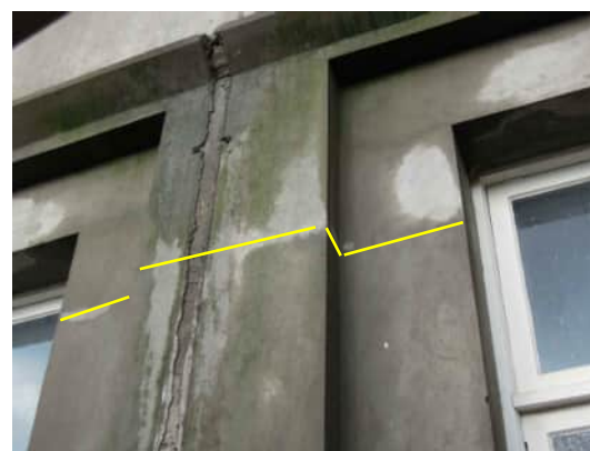
EW14 A-557 | HORIZONTAL CRACK NEAR CEILING LEVEL OF GROUND FLOOR ON COLUMN AT GRID B
