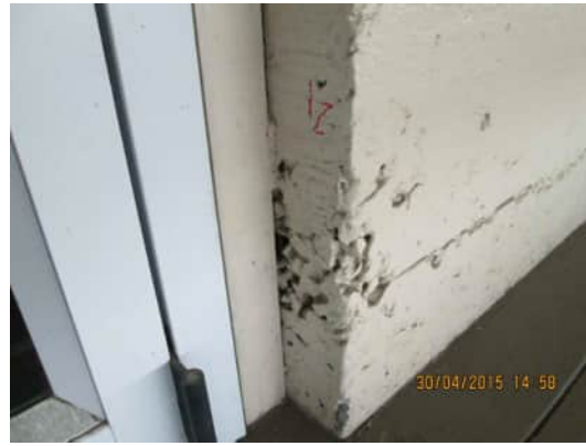
2.50 A-520 | CONCRETE SEGREGATION AT THE BOTTOM OF SHEAR WALL
