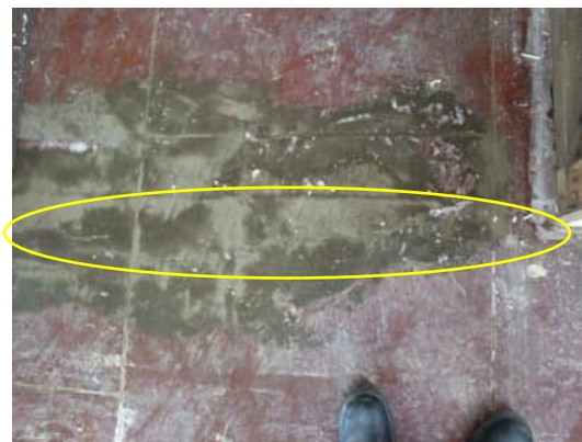
3.10 | CRACK UP TO 2MM WHICH HAS BEEN PREVIOUSLY REPAIRED A-530
