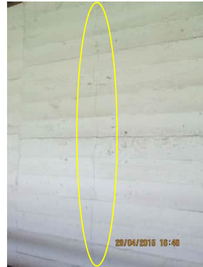
4.8 A-540 | VERTICAL CRACK ON THE EXTERNAL FACE OF THE SHEAR WALL RUNNING PARALLEL TO THE STEEL COLUMN ON INTERNAL FACE
