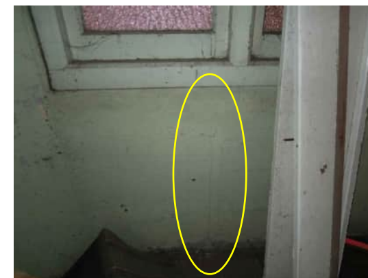
0.23 0.2mm VERTICAL CRACK BELOW WINDOW BETWEEN GRID 2 AND 3 A-500
