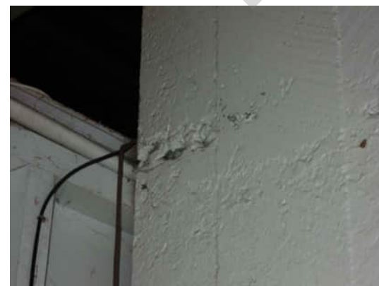
0.33 A-500 | POORLY COMPACTED CONCRETE ON GRID 14 COLUMN
