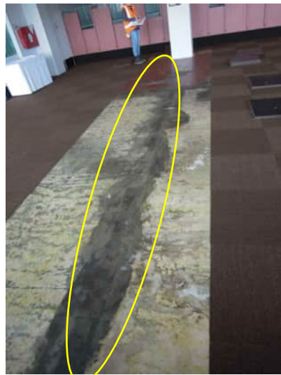
3.5 | CRACK ABOVE GRID 6 BEAM WHICH HAS BEEN PARTIALLY REPAIRED A-530
