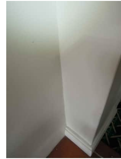
0.39 SEPARATION BETWEEN GRID 13 COLUMN AND GIB LINED WALL A-500
