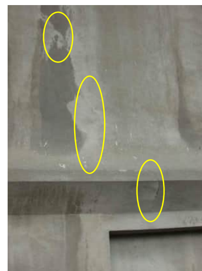
EW11 | VERTICAL CRACK ABOVE GROUND FLOOR WINDOW GRID A AND GRID B A-557
