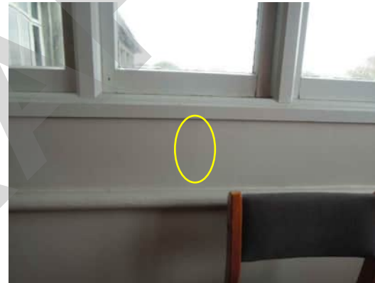
3.19 | HAIRLINE CRACK IN WALL BELOW WINDOW BETWEEN GRID D AND E A-530
