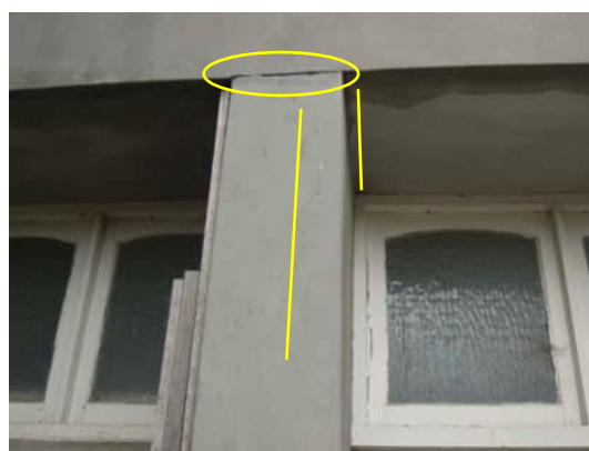
EW22 A-557 | VERTICAL CRACKING TO CENTRAL COLUMN AND SEPARATION BETWEEN THE COLUMN AND THE WALL BETWEEN THE SECOND AND THE THIRD FLOOR
