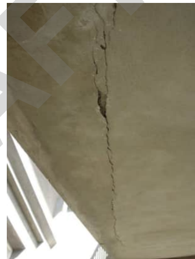
S17 | CRACK ON UNDERSIDE OF STAIRS UP TO 4MM WIDE WITH LOCALISED SPALLING TO RENDER A-816
