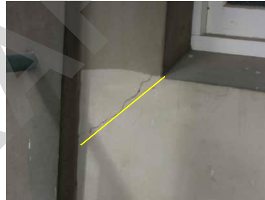
EW7 | DIAGONAL CRACK BELOW WINDOW ON COLUMN BETWEEN AND GRID C A-557
