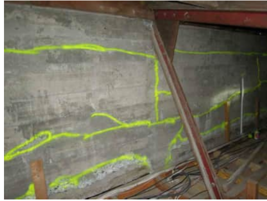
3.49 MULTIPLE CRACKS TO SHEAR WALL. UPPER CRACK IS THROUGH POUR LINE. VERTICAL CRACK UNDER TRUSS IS 1.2MM WIDE. POOR QUALITY CONCRETE IN BEAM AT BOTTOM. MIDDLE HORIZONTAL CRACK IS 1.8 TO 2MM WIDE A-530
