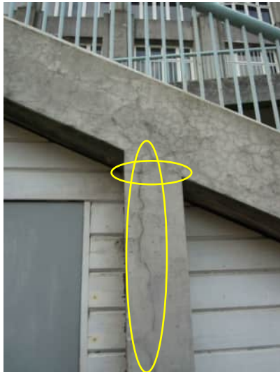
R5 A-810 VERTICAL CRACK DOWN COLUMN AND HORIZONTAL CRACK AT JOINT
