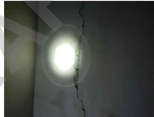
1.19 | SPALLING OF CRACK BETWEEN WALL AND COLUMN AT GRID D A-510
