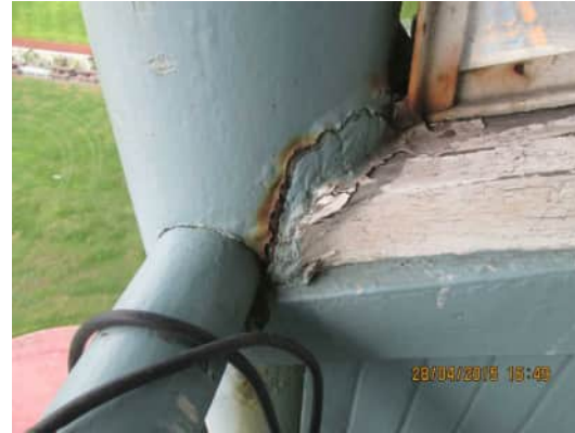
4.15 A-540 | DAMAGE TO INTERFACE BETWEEN COLUMN AND TIMBER INFILL
