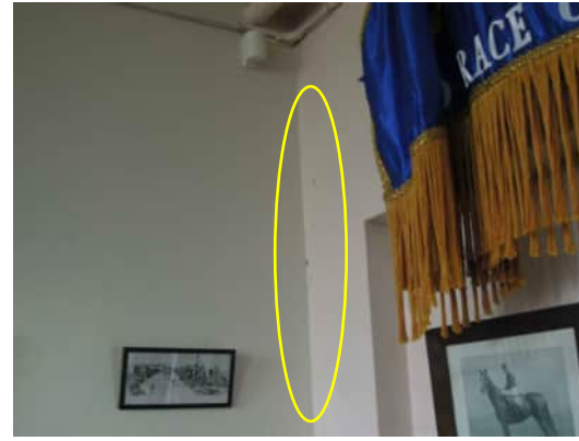
2.15 | SEPARATION BETWEEN GRID D COLUMN AND WALL A-520
