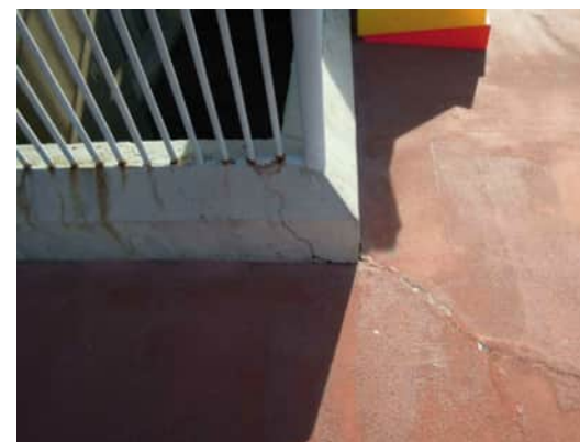
EXT.10 | CRACK IN SLAB FROM CORNER OF RETAINING WALL A.710
