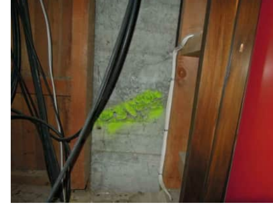
3.52 POOR QUALITY CONCRETE BETWEEN TWO VOIDS A-530
