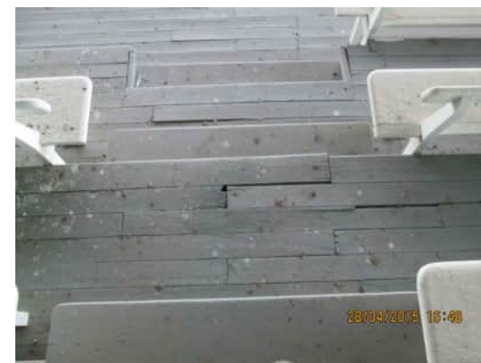
4.12 A-540 | CONDITION OF TIMBER DECKING ON THE UPPER STAND
