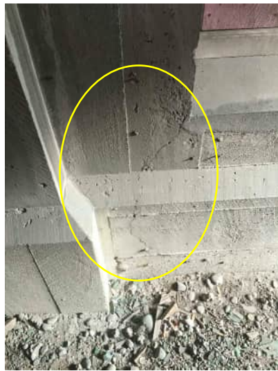
EN5 A-552 CRACK FROM CORNER OF WINDOW
