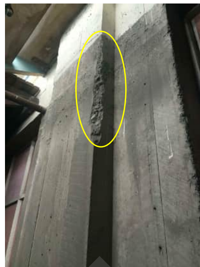
EN3 A-552 SPALLING TO CORNERS OF COLUMNS
