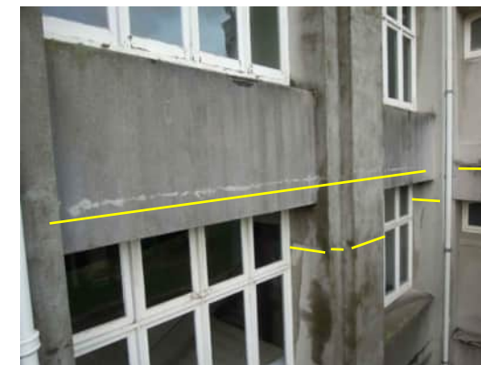
ES8 A-550 | TYPICAL HORIZONTAL CRACK ABOVE WINDOW AND HORIZONTAL CRACK AROUND COLUMN
