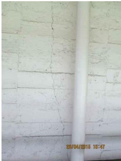
4.10 A-540 | VERTICAL CRACK ON THE EXTERNAL FACE OF THE SHEAR WALL RUNNING PARALLEL TO THE STEEL COLUMN ON INTERNAL FACE
