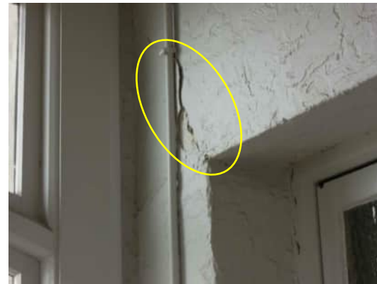
1.12 | DIAGONAL CRACK FROM TOP CORNER OF WINDOW IN WALL BETWEEN GRID B AND C A-510
