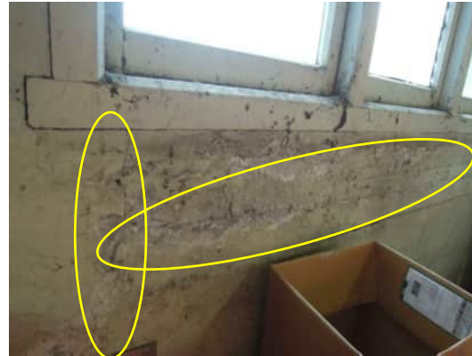
0.49 | HORIZONTAL AND VERTICAL CRACK BELOW WINDOW BETWEEN GRID 7 AND 8 A-500
