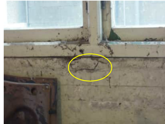
0.50 | SIGNIFICANT CRACK BELOW WINDOW BETWEEN GRID 8 AND 9 A-500
