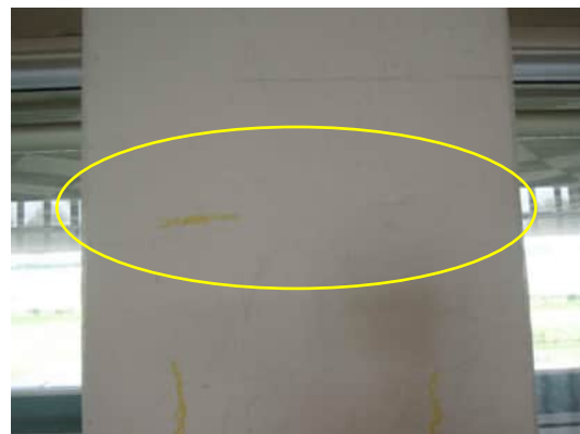
2.21 | HAIRLINE CRACK AROUND GRID 6 COLUMN A-520 | (GRID 3, 14 AND 15 COLUMNS SIMILAR)
