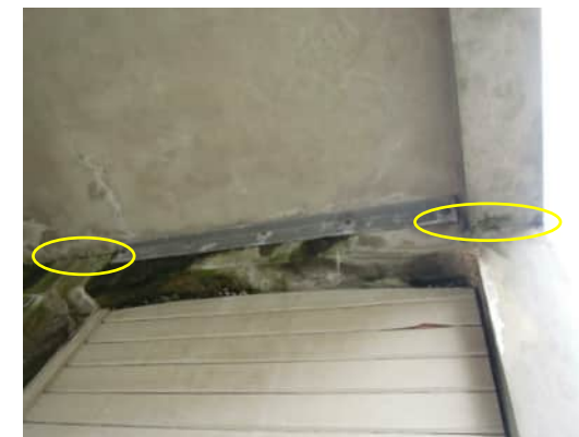
R8 A-810 CRACK CONTINUES TO OTHER SIDE OF PLATFORM
