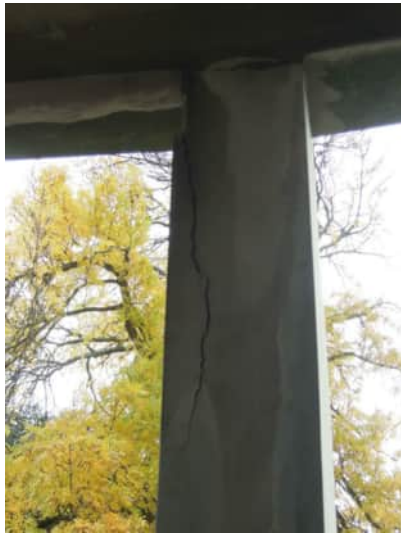
R13 A-810 | CORNER SPALLING OFF COLUMN
