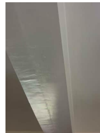
2.36 | TYPICAL CRACKS ALONG LENGTH OF BEAM A-520
