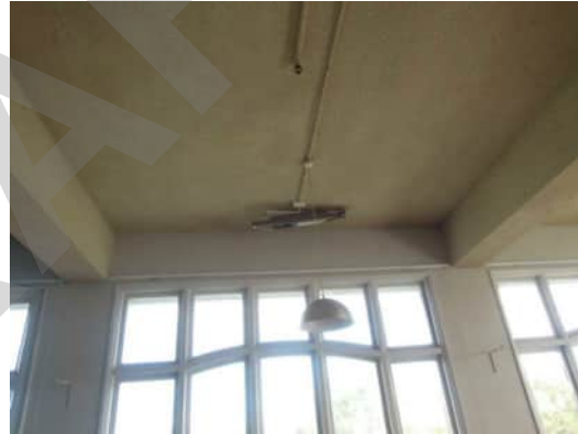
3.43 HEATER INADEQUATELY CONNECTED TO CEILING - HAZARD A-530
