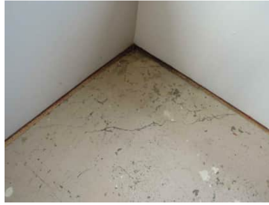
3.14 | CRACKS IN CORNER UP TO 0.6MM A-530
