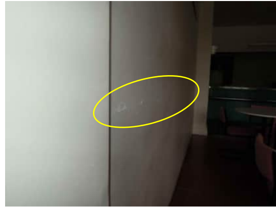
0.17 CRACK TO THE PLASTER A-500
