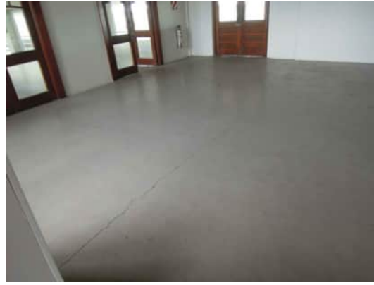
2.2 | CRACK ABOVE BEAM ON GRID 9, UP TO 10MM A-520
