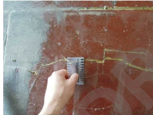
3.6 | CRACK ABOVE GRID 6 BEAM IS UP TO 5MM WIDE A-530
