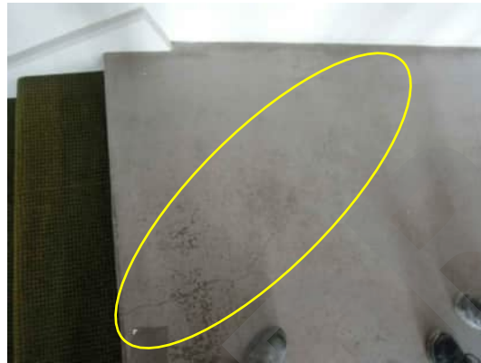
2.6 | CRACK AT TOP OF STAIRS UP TO 1.6MM A-520
