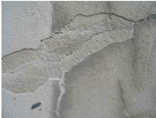
EE17 A-554 | 0.2MM CRACK IN GRID C COLUMN
