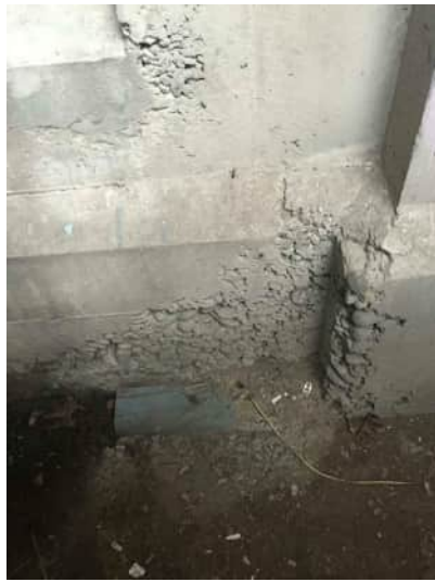
EN1 A-552 AREA OF SEGREGATED CONCRETE AT BASE OF COLUMN AND WALL
