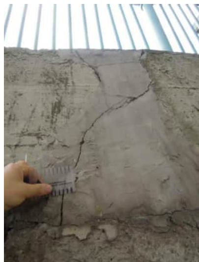
RW.9 CRACKS UP TO 2.5MM WHICH HAVE PREVIOUSLY BEEN REPAIRED BUT HAVE REAPPEARED A.710
