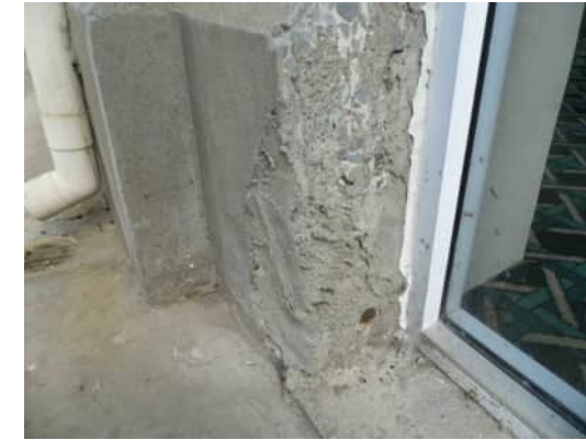
EE8 A-554 DAMAGED CONCRETE AROUND DOOR WITH REINFORCING EXPOSED (WALL APPEARS TO HAVE BEEN CUT TO FORM DOOR)
