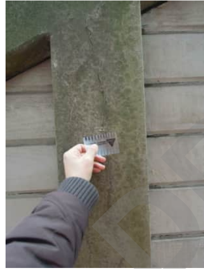
R6 A-810 VERTICAL CRACK DOWN COLUMN UP TO 1.2MM
