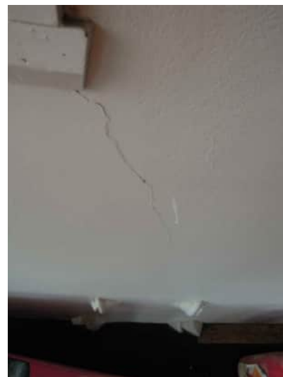
3.22 | 0.3MM DIAGONAL CRACK FROM BOTTOM OF WINDOW AT GRID 2 COLUMN A-530
