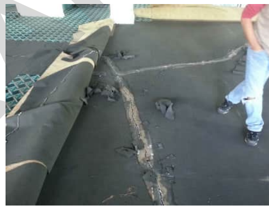
0.7 A-500 | SIGNIFICANT CRACKS IN SLAB WHERE CARPET HAS BEEN PULLED UP
