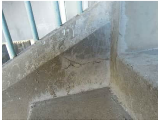
S5 A-814 | CRACK WHERE THE STAIRS CONNECT TO THE BUILDING
