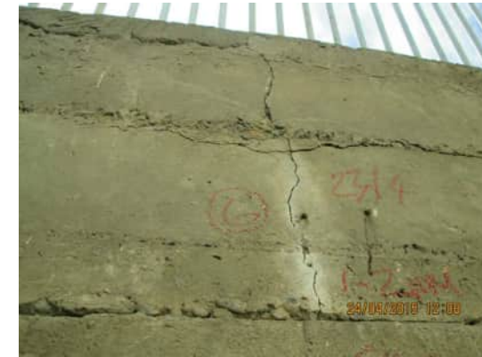
RW.8 VERTICAL CRACK FROM TOP OF WALL TO JOINT AND A HORIZONTAL CRACK RUNNING THROUGH A.710
