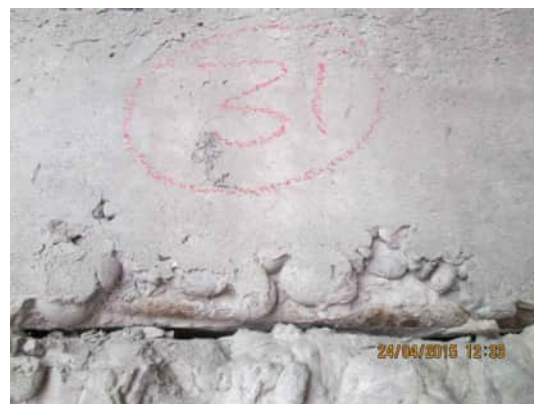
RW.13 | SIGNIFICANT HORIZONTAL CRACK AT JOINT AND EXPOSED REINFORCEMENT AT APPROXIMATELY 600MM FROM THE TOP OF THE WALL A.710
