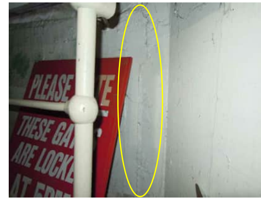
0.27 A-500 | VERTICAL CRACKS BELOW WINDOW BETWEEN GRID 13 AND 14
