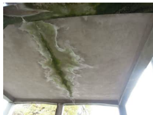
R10 A-810 SIGNIFICANT CRACK THROUGH PLATFORM
