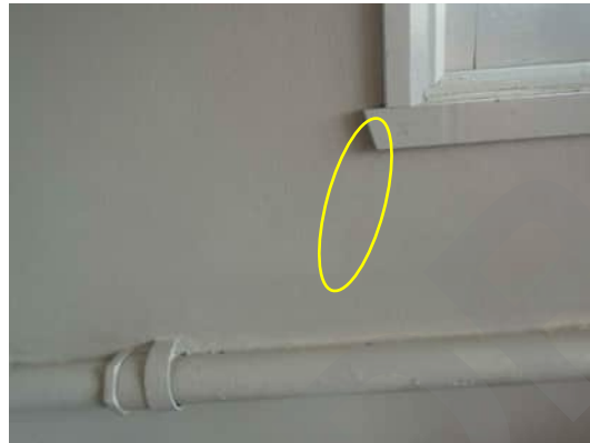
3.18 | HAIRLINE CRACK FROM CORNER OF WINDOW IN GRID D COLUMN A-530
