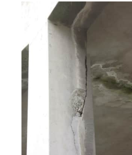
R11 A-810 CORNER BREAKING OFF COLUMN EXPOSING REINFORCING
