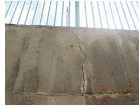
RW.4 TYPICAL CRACK FROM TOP OF WALL TO JOINT, CRACKS RANGE FROM 0.2MM TO 5MM A.710
