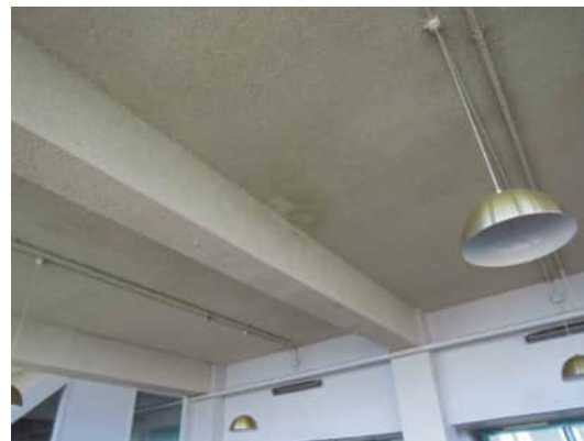
3.47 MOISTURE DAMAGE TO BEAM AND CEILING AT GRID 15 A-530
