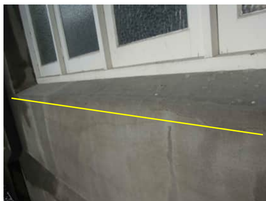
EW9 | HORIZONTAL CRACK BELOW WINDOW A-557
