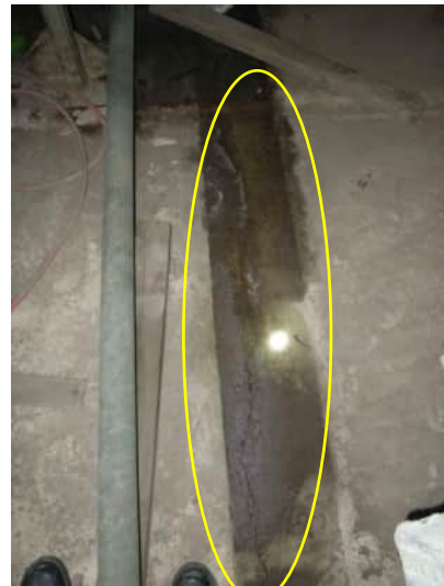
4.2 A-540 | CRACK THROUGH DRAINAGE CHANNEL, UP TO 1.4MM
