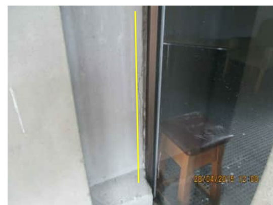
ES2 A-550 SEPARATION BETWEEN GRID 10 COLUMN AND LIFT SHAFT EXTENSION
