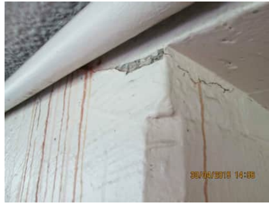
2.49 A-520 | CRACKING TO TOP OF COLUMN AT GRID 13
