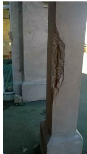
R22 A-810 | CORNER SPALLED OFF COLUMN EXPOSING REINFORCING
