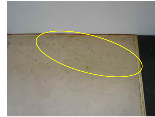
3.4 | DIAGONAL CRACK IN CORNER UP TO 1.2MM A-530
