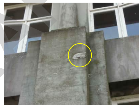
ES11 A-550 | SPALLING NEAR TOP OF GRID 3 COLUMN EXPOSING REINFORCING
