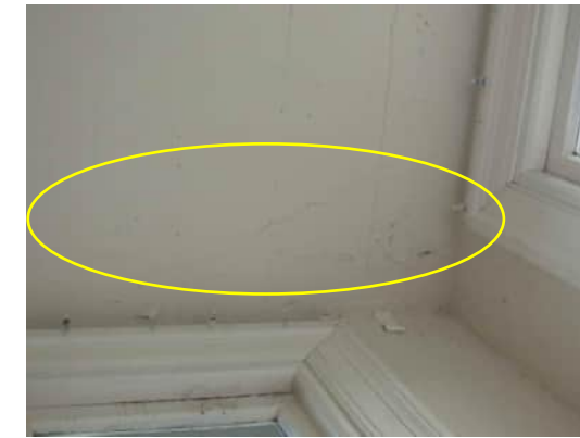
2.40 A-520 | CRACK IN CORNER OF SLAB SOFFIT AT GRID 1/D
