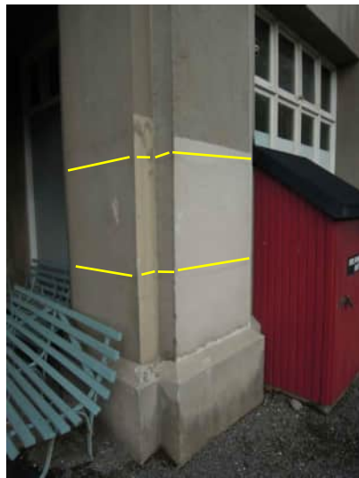
EW5 | 0.2MM HORIZONTAL CRACKS NEAR BASE OF GRID C COLUMN A-557
