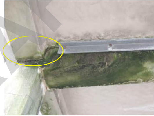
R7 A-810 SIGNIFICANT CRACK BETWEEN BEAM AND SLAB, BENEATH STEEL ANGLE
