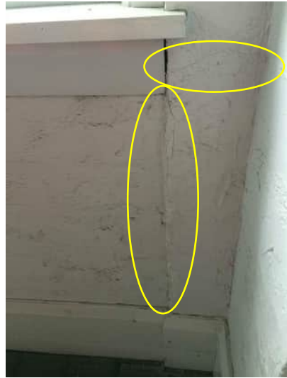
1.25 | CRACK IN CORNER OF GRID C COLUMN BELOW WINDOW A-510
