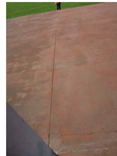
EXT.7 | TYPICAL CRACK IN JOINT A.710
