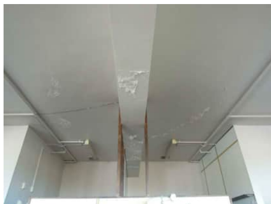
3.46 MOISTURE DAMAGE TO CEILING AND BEAM ON GRID 11 A-530
