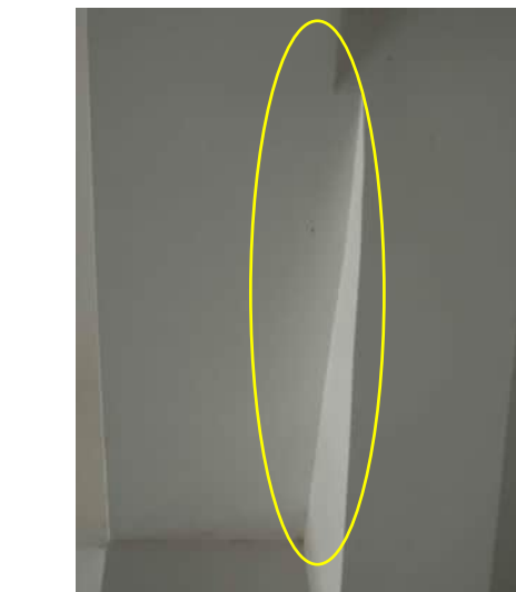
2.45 A-520 | SEPARATION BETWEEN CEILING AND STAIRS
