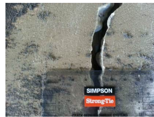
0.8 A-500 | CRACK UP TO 15mm
