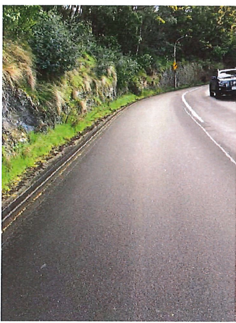
Lack of general maintenance Road side overgrowth
