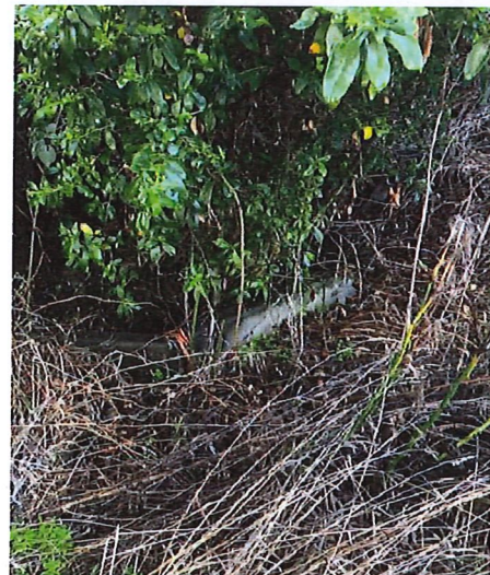
Over grown main storm water sump
