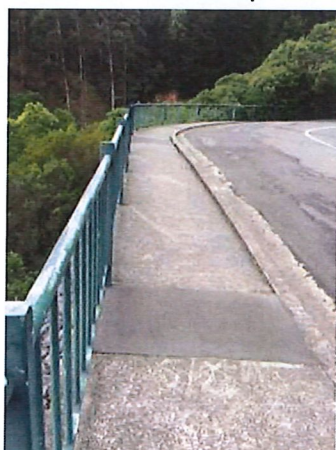
Kerb elevated above footpath
