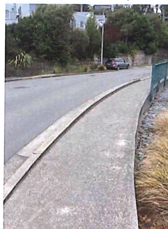
Kerb elevated above footpath
