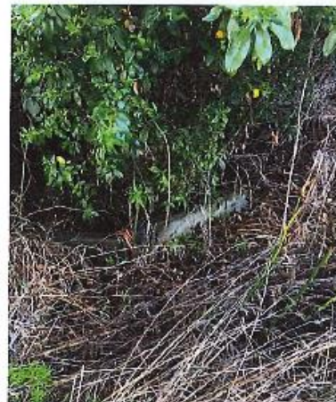
Over grown main storm water sump
