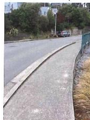
Kerb elevated above footpath
