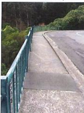
Kerb elevated above footpath
