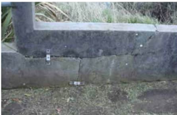
Cracks in concrete surrounding wall. Note "telltales"
