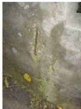
Damage caused by rusting reinforcing.
