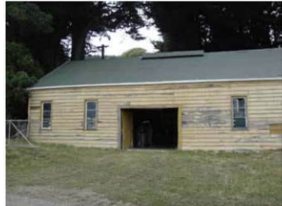
West wall. Note flaking paint and other defects
