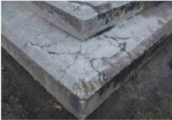
Base of monument showing cracking
