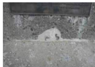
Patch to base of monument
