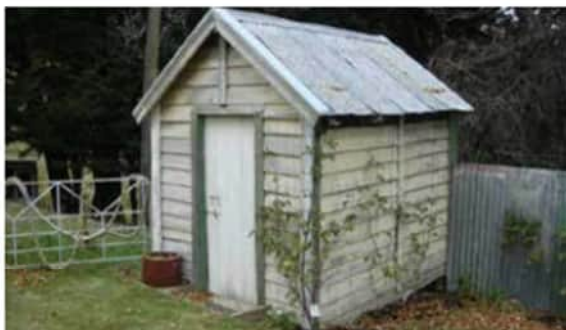
Outbuilding, possibly used originally as a dairy. It appears to have been built with material "left over" when the barracks was reconstructed.
