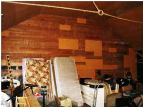
Barracks interior. Note patches on wall over earlier linings
