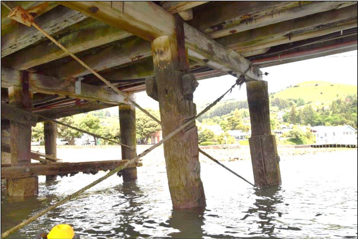
Photo 6 An example of repairs and alterations to a bent – original timber bracing cut off either side of the central pile; diagonal steel braces installed; and a steel jacket added to the right-hand pile.
