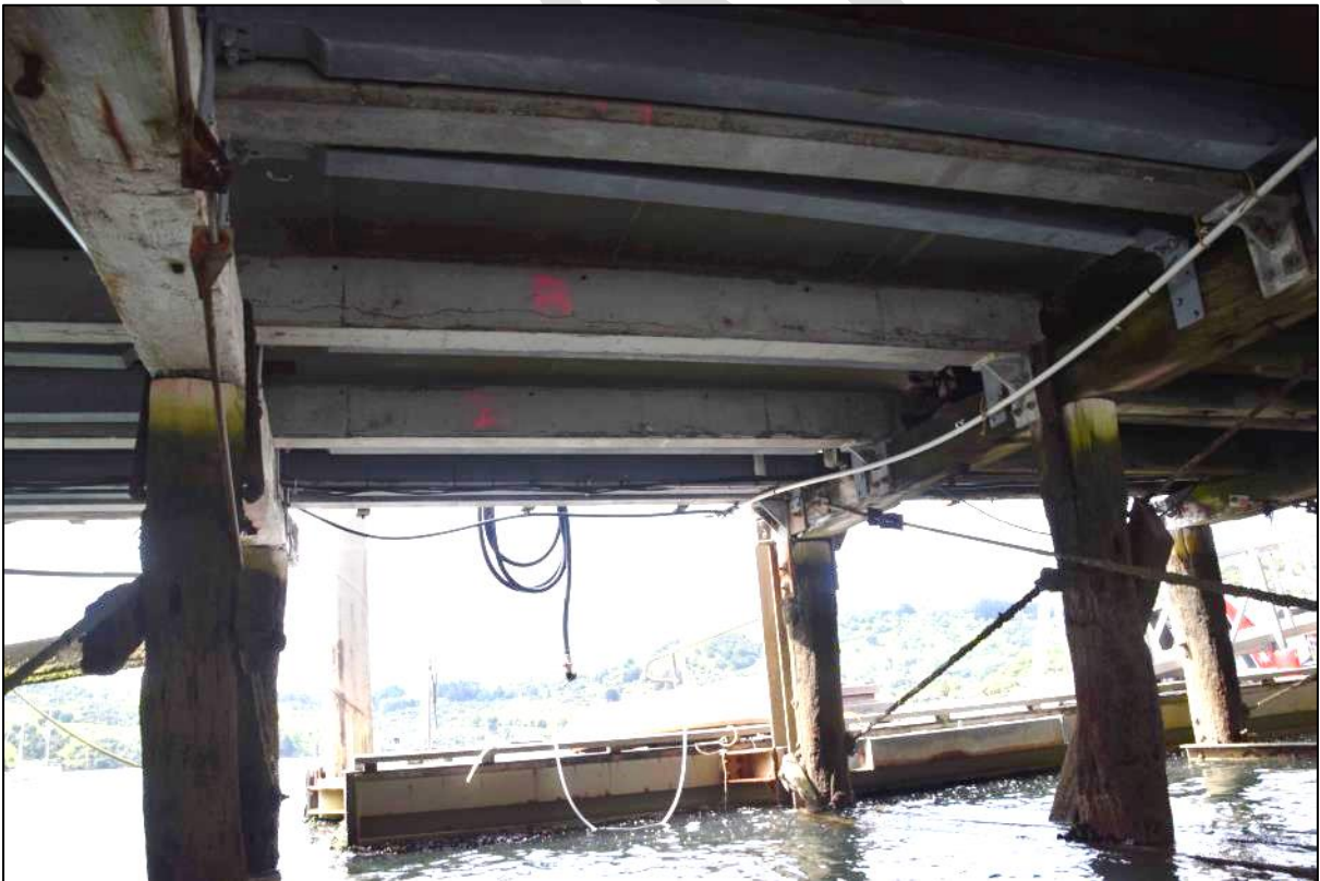
Photo 41 A close-up of inserted concrete and steel beams (Photo 40) – some of the concrete beam are cracked. Poorly restrained and concealed modern conduits.
