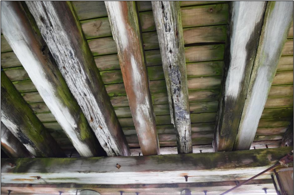
Photo 28 Additional stringers inserted to strengthen the deck at the western end of the wharf. There is considerable erosion and decay in many of the stringers here.
