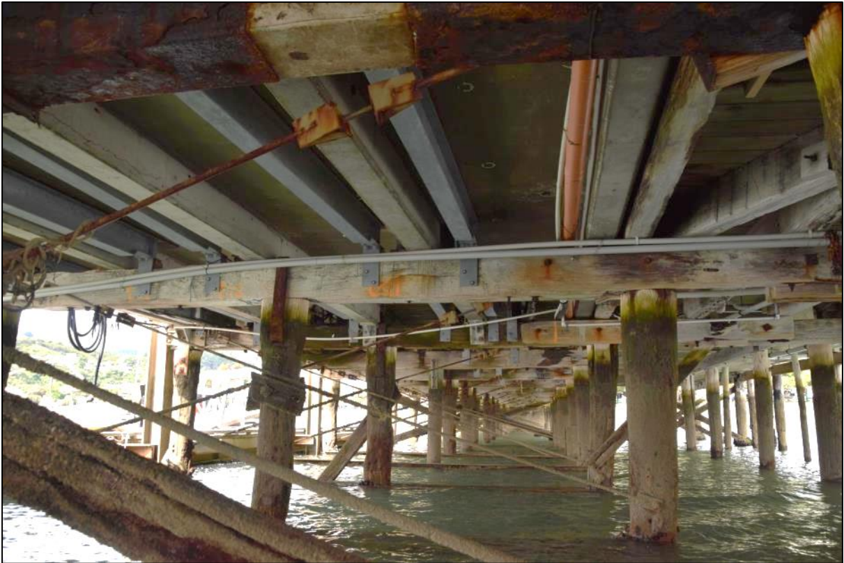
Photo 40 Substantial alterations/repairs with steel and concrete beams below the deck adjacent to the north floating pontoon.
