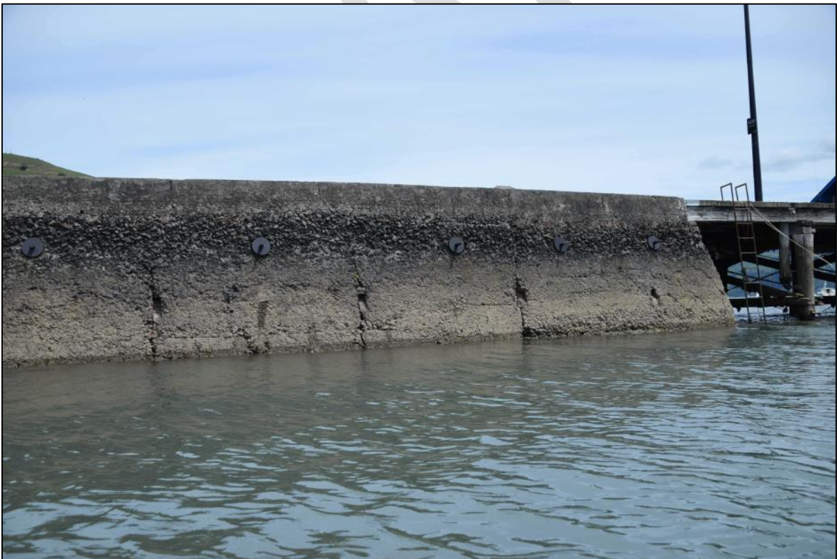
Photo 3 The outer north wall of the abutment with drainage holes, circular pattress plates to the end of the tie rods and many cracks in the masonry.
