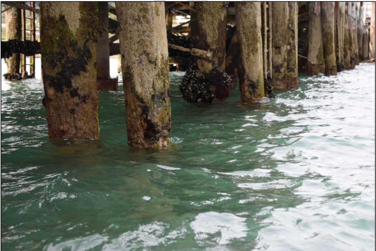
Photo 27 Severe decay at the water line to a fender pile on the south side of the wharf towards the western end. The photograph shows rows of piles and adjacent fender piles, many of which are thought to be original and of Ironbark timber.
