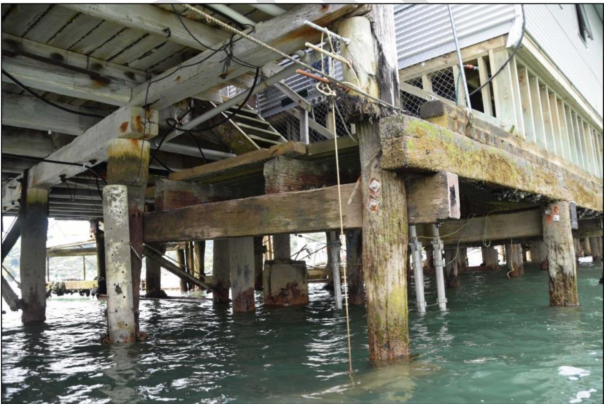
Photo 21 Between about bents 13 and 15 from the abutment, the south side of the wharf has been lowered in the past. None of the historic photographs show this lower and, hence, it seems to have been a 1970s or later alteration. In order to maintain the floor level, the corner of the modern shed (top right) has had to be built up on jack studs (with an area for services and plastic tanks below the floor). Note the steel props under the lowered deck.
