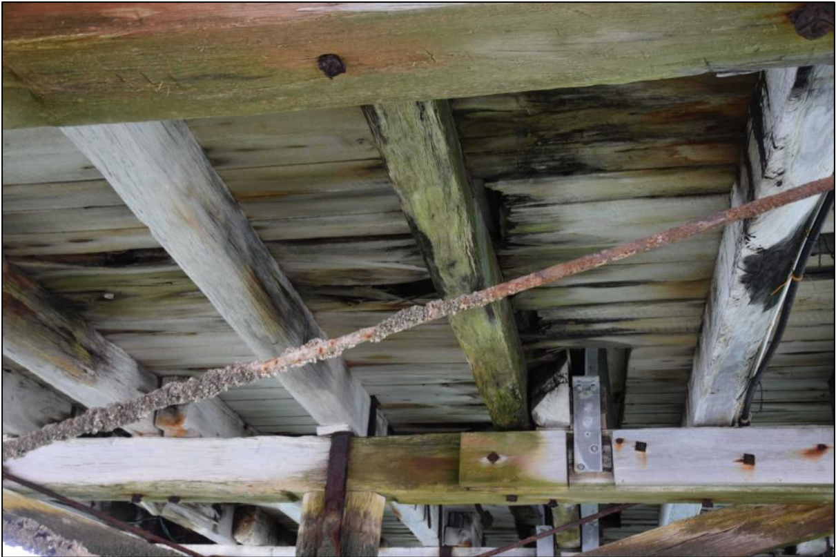
Photo 32 Decay in the decking boards and modern steel straps added.
