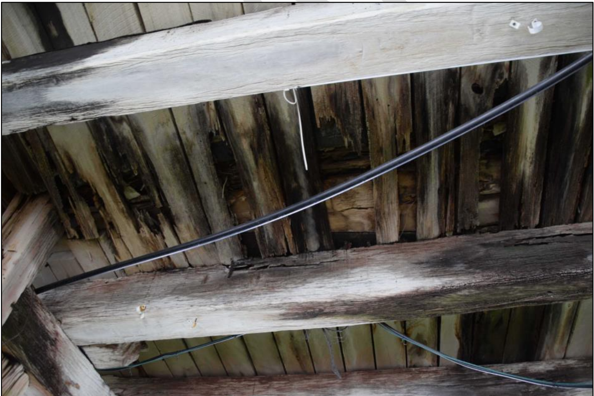
Photo 37 Further decay in decking boards beneath the existing deck finish.
