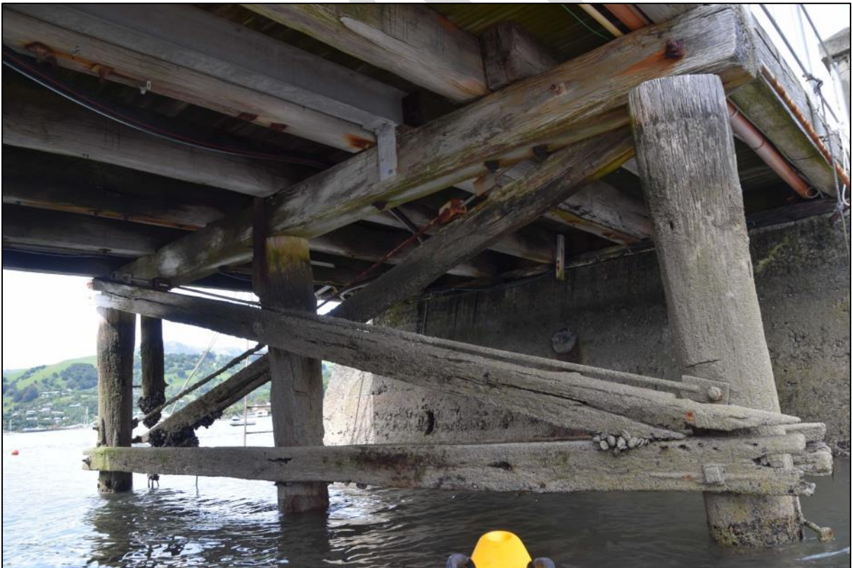
Photo 45 The first bent and the stringer/deck connection to the abutment. This part of the structure contains many original elements, including the pile cap, central pile with wrought iron strap connection to the cap, bracing timbers and horizontal wale between the piles, and timber stringers between the pile cap and modern decking boards.
