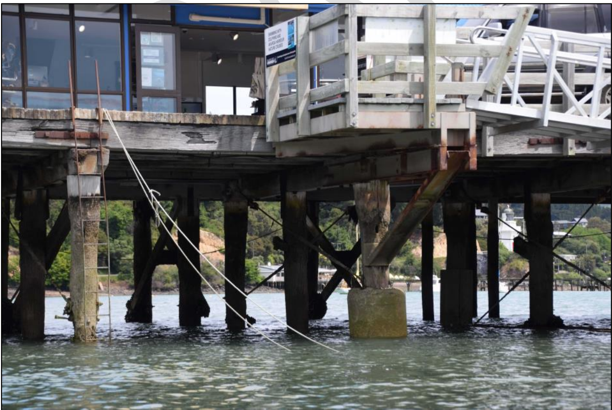
Photo 7 Further alterations on the north side of the wharf with steel added to support the gantry to the floating pontoon and concrete cast to the base of the pile supporting the steel framing.
