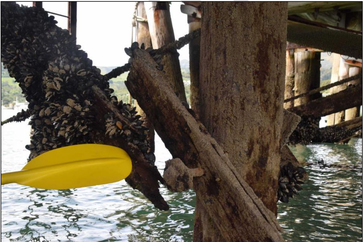
Photo 33 Broken timber brace.
