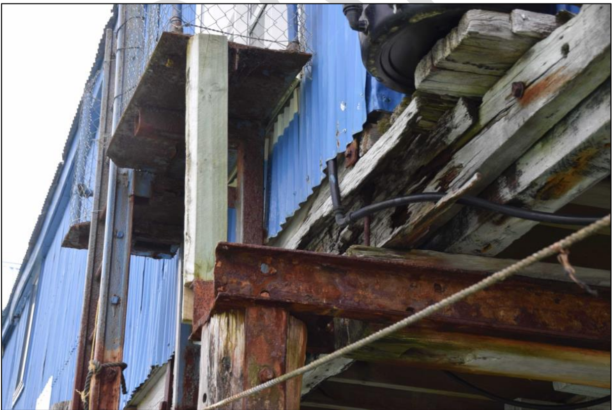
Photo 19 Timber decay and corrosion at the junction of two of the modern sheds (south side approx. 16th bent from the abutment).
