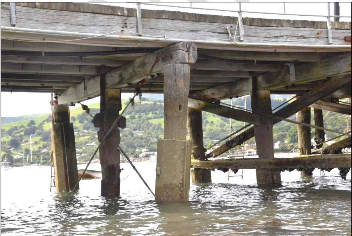
Photo 25 The same bent as in Photo 6, but from the south side. Both outer piles have 'jacket' repairs and the bent is missing its original horizontal brace. The diagonal timber braces have been cut off and replaced by steel rods.
