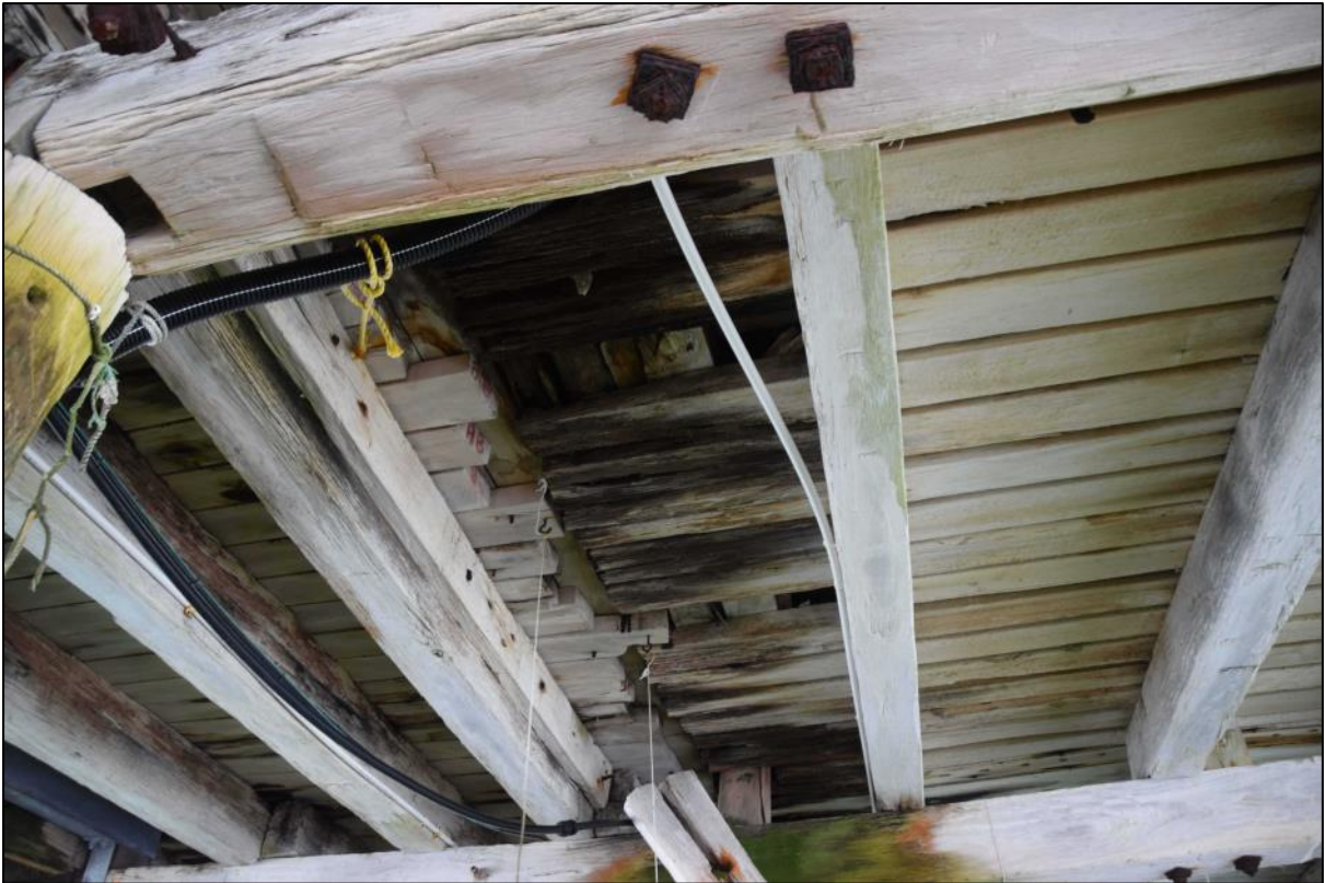
Photo 36 Decay in decking boards beneath the existing deck finish. Corrosion to original iron bolts and nuts.
