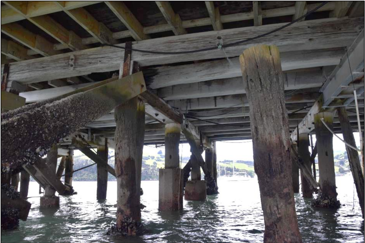
Photo 16 An image underneath the western end of the sheds showing the modern tanalised floor structure to one of the sheds (top) and steel strengthening added to the pile caps (centre and right foreground).
