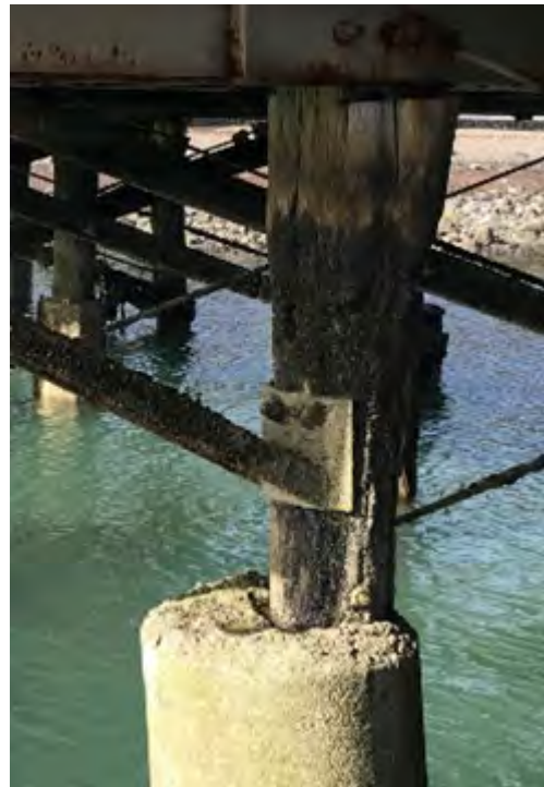
Figure 7: Pile with necking and concrete encasement repair.
