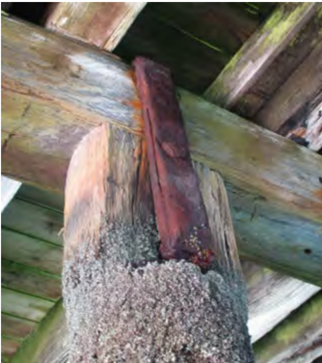
Figure 6: Corrosion to fixing at top of pile. Fixing consistent with original 1878 detailing.
