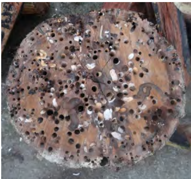
Figure 11: Marine borer damage to hardwood pile
