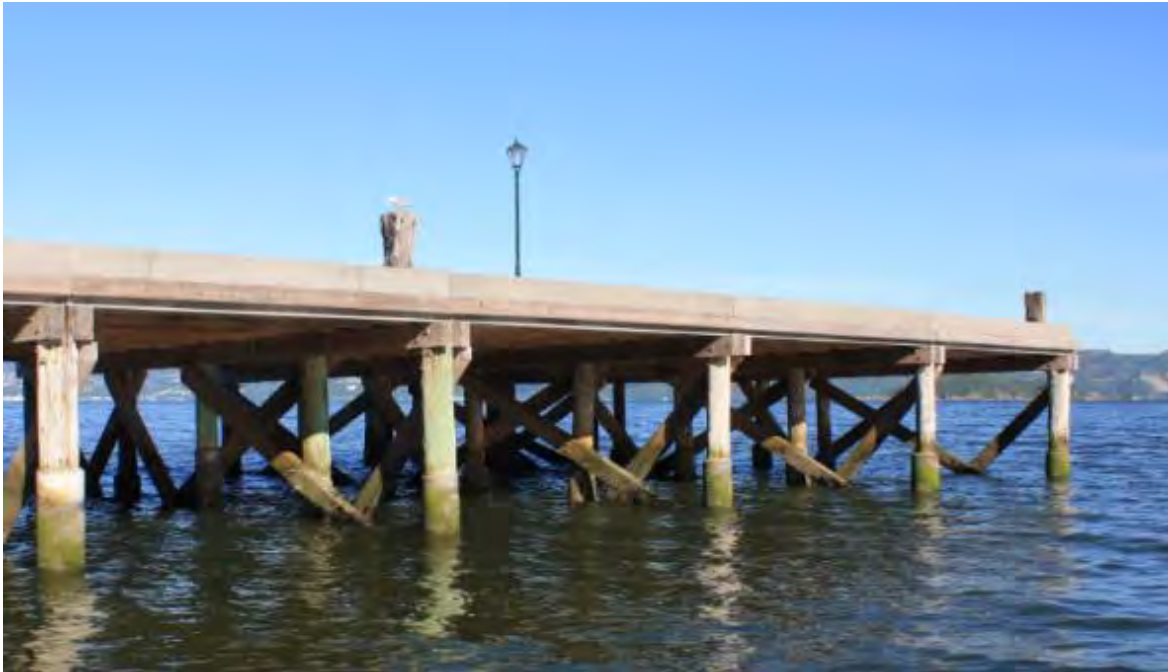
Figure 20: Rona Bay Wharf, timber piles and bracing with concrete edge beam and deck
