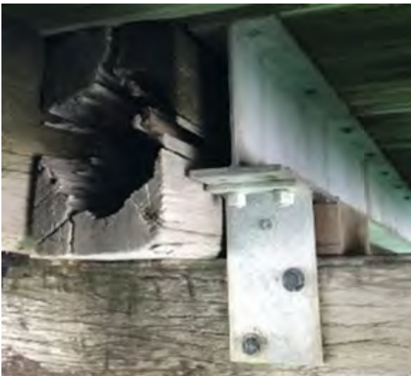
Figure 4: Deteriorated timber beam with new galvanised steel installed alongside
