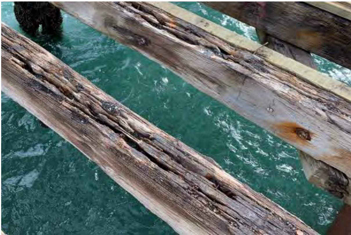
Figure 10: Stringer deterioration from freshwater ingress, typical for traditional hardwood structures
