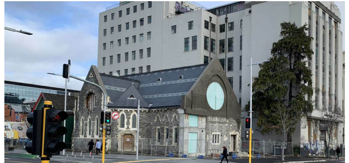
D View of the site owned by the Christchurch Heritage Trust (historic Trinity Congregational Church). The building has been stabilised and is being preserved after experiencing significant earthquake damage, currently cordoned off with temporary fencing. This listed as a heritage item (580), the Shands building (256) has been relocated into the site to the left of the church (behind the church), and the Former State Insurance Building at 116 Worcester Street (577).
