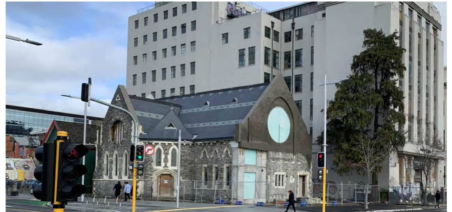
D View of the site owned by the Christchurch Heritage Trust (historic Trinity Congregational Church). The building has been stabilised and is being preserved after experiencing significant earthquake damage, currently cordoned off with temporary fencing. This listed as a heritage item (580), the Shands building (256) has been relocated into the site to the left of the church (behind the church), and the Former State Insurance Building at 116 Worcester Street (577).
