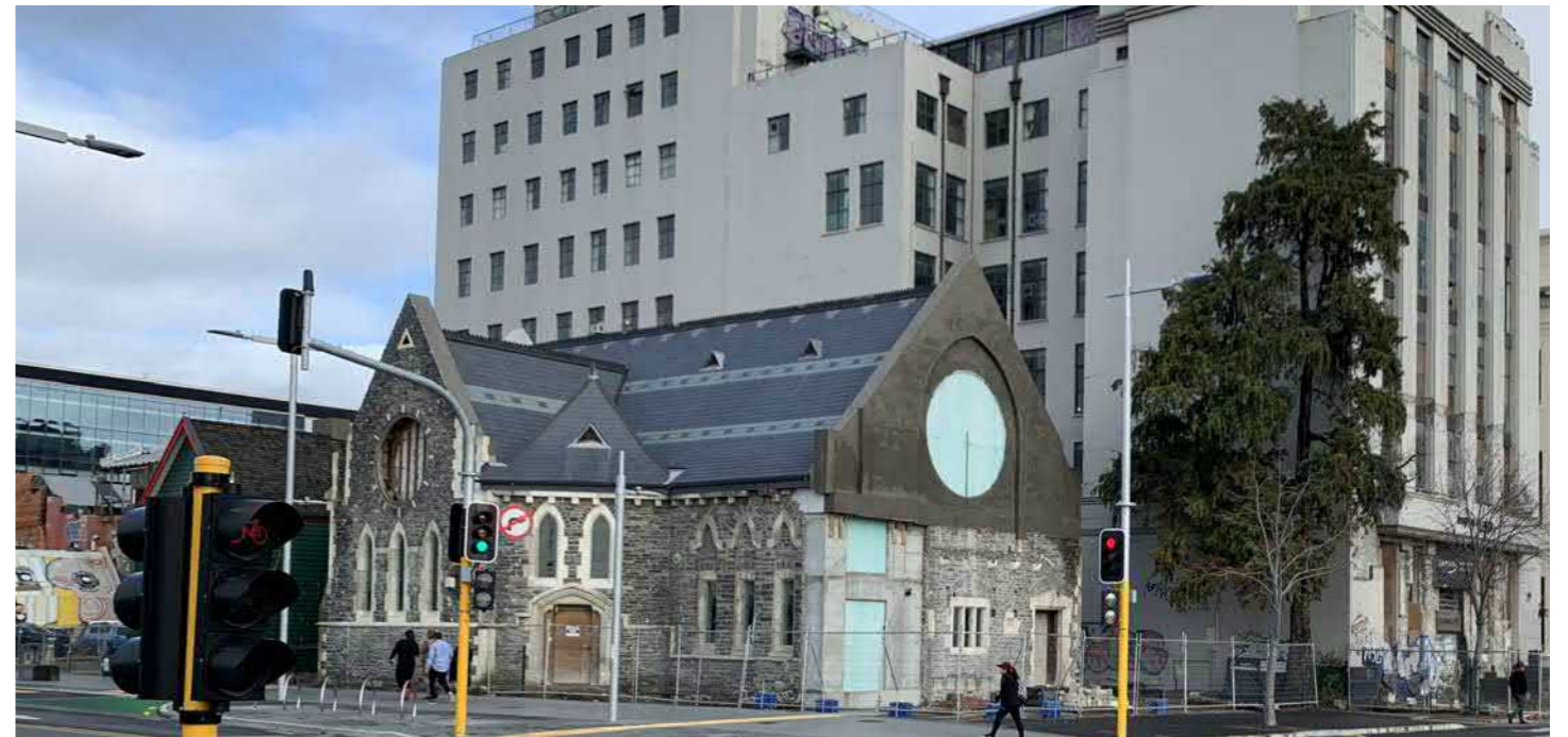
D View of the site owned by the Christchurch Heritage Trust (historic Trinity Congregational Church). The building has been stabilised and is being preserved after experiencing significant earthquake damage, currently cordoned off with temporary fencing. This listed as a heritage item (580), the Shands building (256) has been relocated into the site to the left of the church (behind the church), and the Former State Insurance Building at 116 Worcester Street (577).
