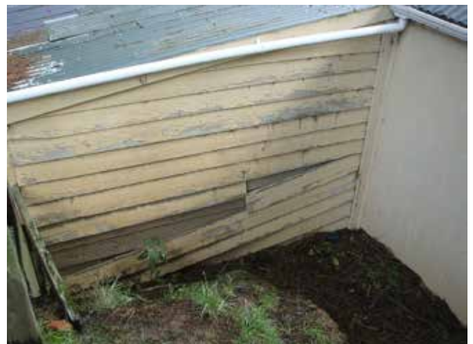
Loose weatherboards on eastern lean-to. Note fibre-cement sheathing on adjacent wall.
