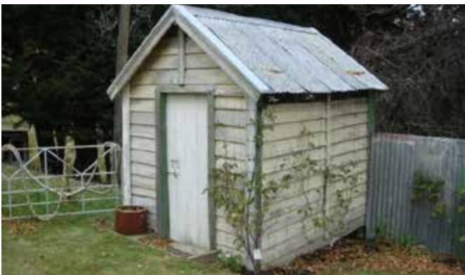
Outbuilding, possibly used originally as a dairy. It appears to have been built with material “left over” when the barracks was reconstructed.
