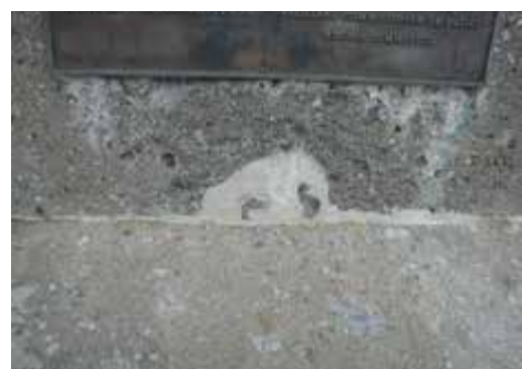
Patch to base of monument
