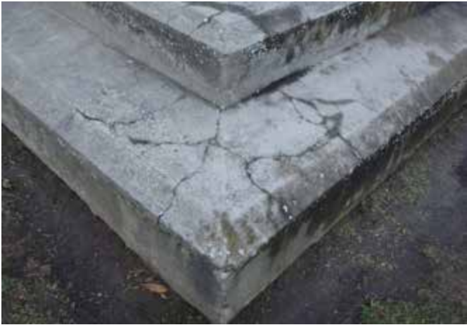
Base of monument showing cracking
