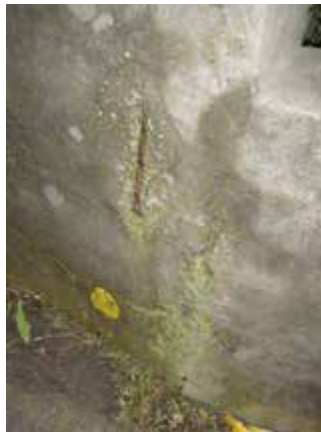
Damage caused by rusting reinforcing.
