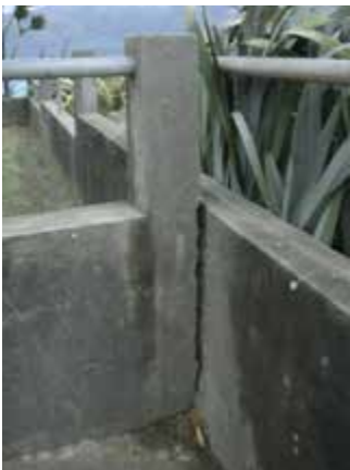
Evidence of ground movement as seen by walls separating
