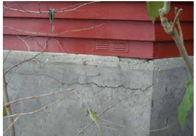
Cracks in foundation wall and spalling of plasterwork
