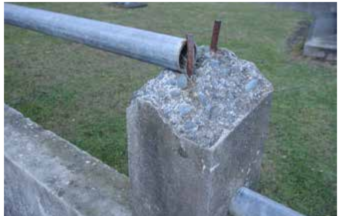
Spalling plasterwork and missing top section of post
