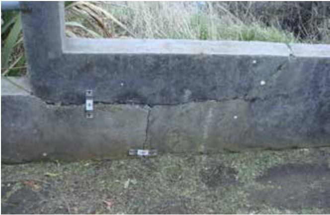
Cracks in concrete surrounding wall. Note “telltales”
